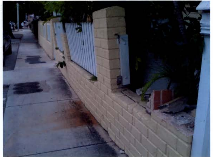
Sections of the wall have fallen onto Sidewalk & been cleared
