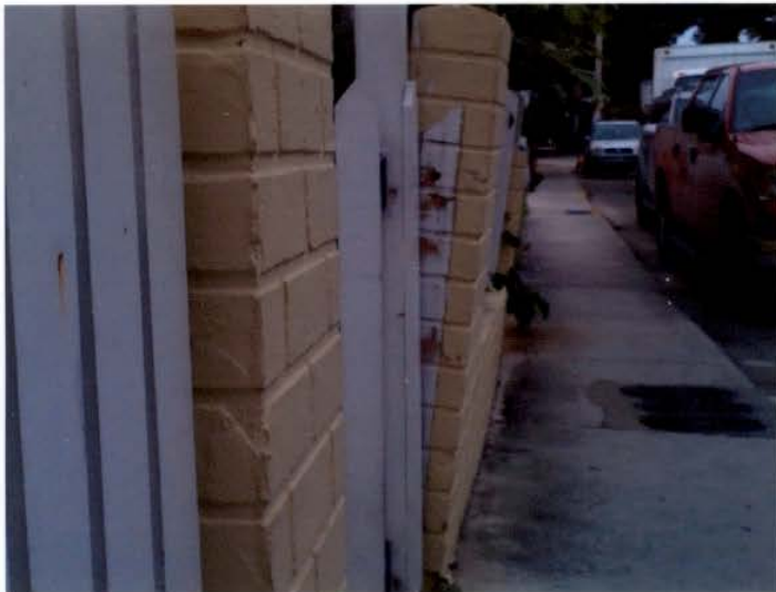
Wall being pushed by plants
