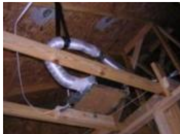
Poor installation (U bend)
