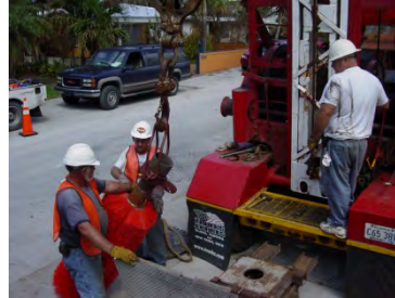
The pump-assisted storm water injection wells implemented by our team have helped resolve chronic flooding in key tourist areas.
