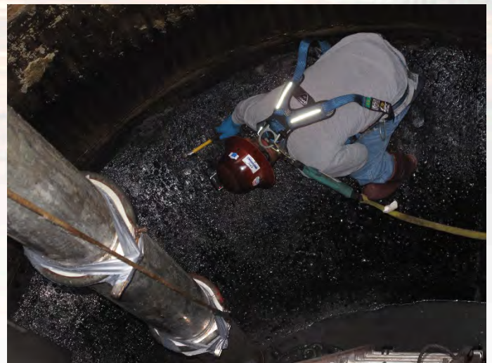
CH2M's proposed Program Manager, Lower Keys resident Sean McCoy, P.E., at work in a wetwell on the Wastewater Pump Station H & B Rehabilitation project for the City of Key West.
