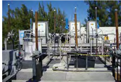
The Headworks Modifications allow the City to treat wastewater flow more efficiently as well as treating additional flow to the plant during extreme weather conditions.
