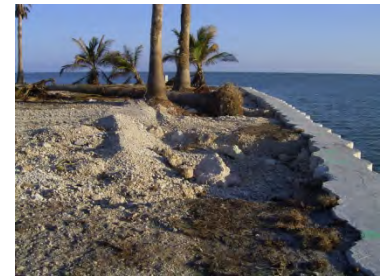
Strengthening of the bulkheads and seawalls in the Keys, will provide greater protection during storm events.
