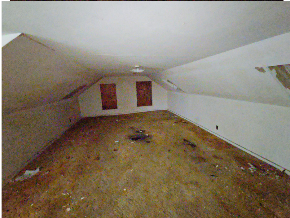
1/2 STORY WATER DAMAGE
