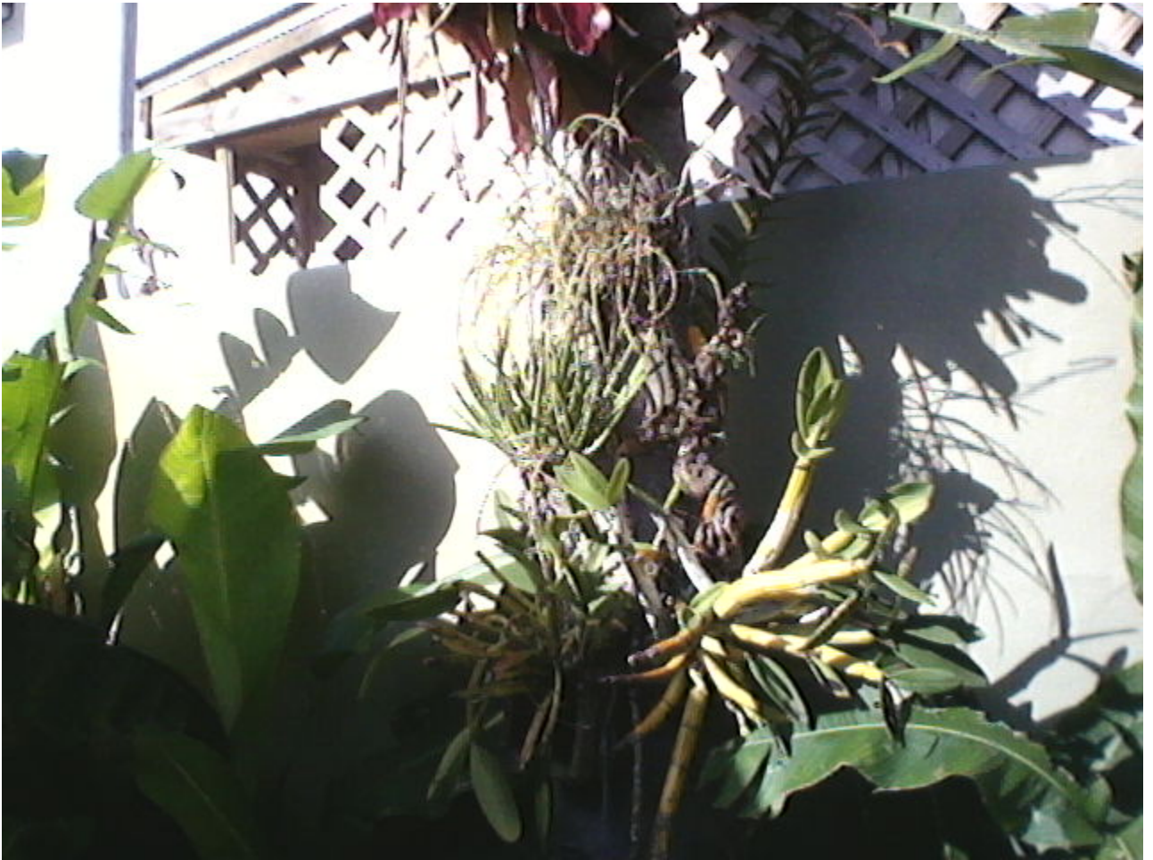
Picture of trunk next to wall and cracks in the wall
