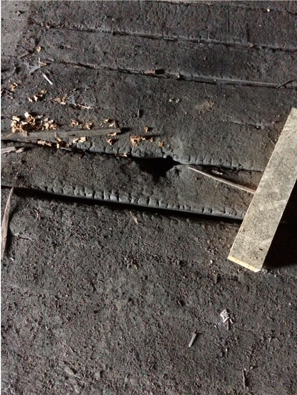
Photo: Existing Conditions; Charred Attic Flooring
