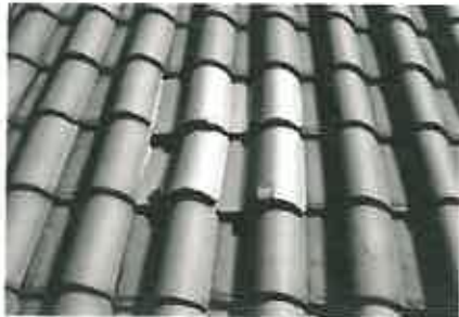
Repairs on this pantile roof were made with new tiles held in place with metal hangers. Photo: NPS files.
