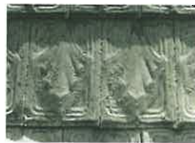
Tin shingles, commonly embossed to imitate wood or tile, or with a decorative design, were popular as an inexpensive, textured roofing material. Photo: NPS files.
