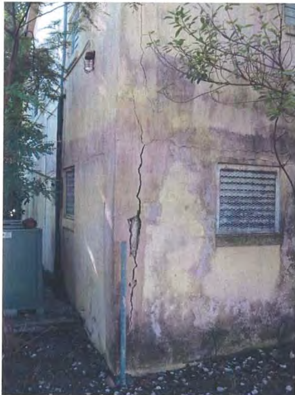
Detail photo of spalling at NE corner of building. Contractor to repair spalling at tie beams and columns and patch stucco. See structural details and specifications.
