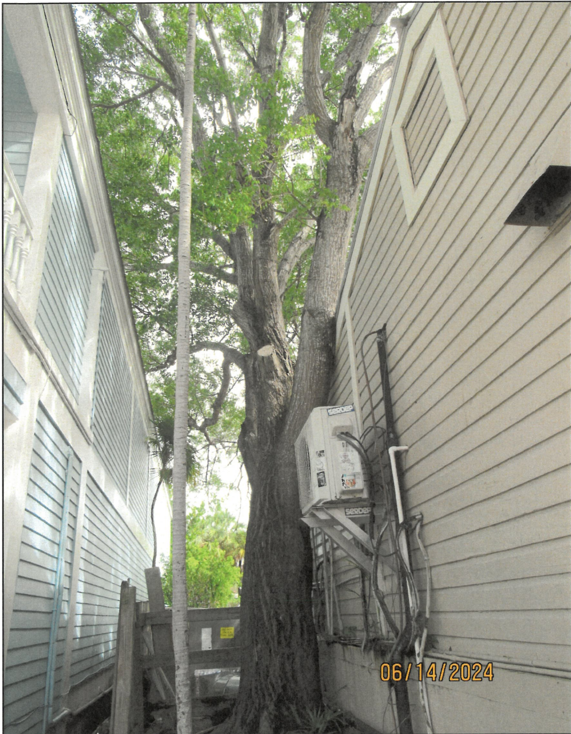
This mahogany tree was a volunteer, and not planted. It was not intended to be a tree. It's location is causing damage to the roof of the building on the right.
