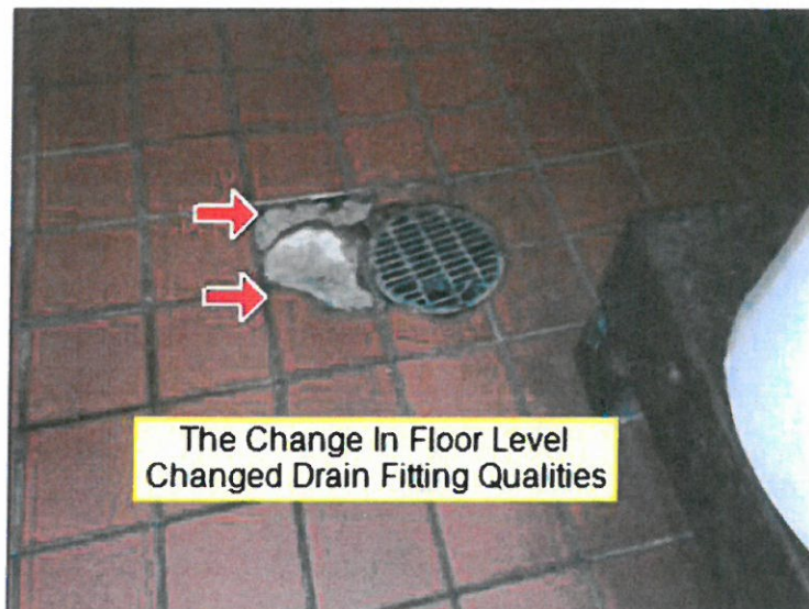
4.0 Picture 2 Kitchen Drain System
