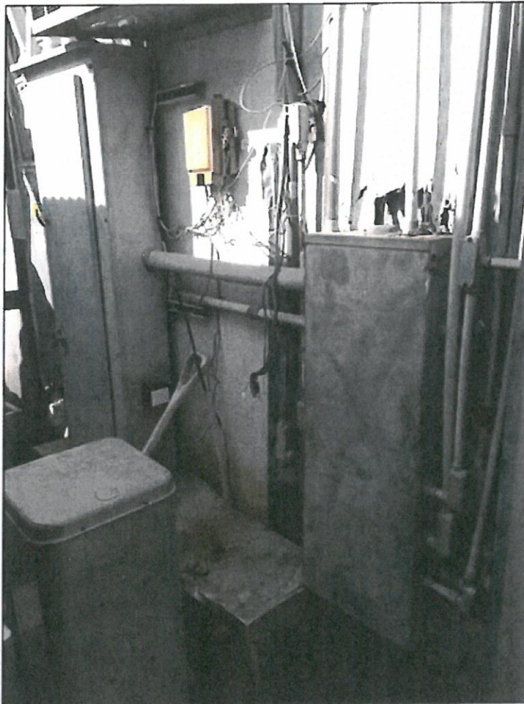
8.1 Picture 1 Underground Service Entrance
