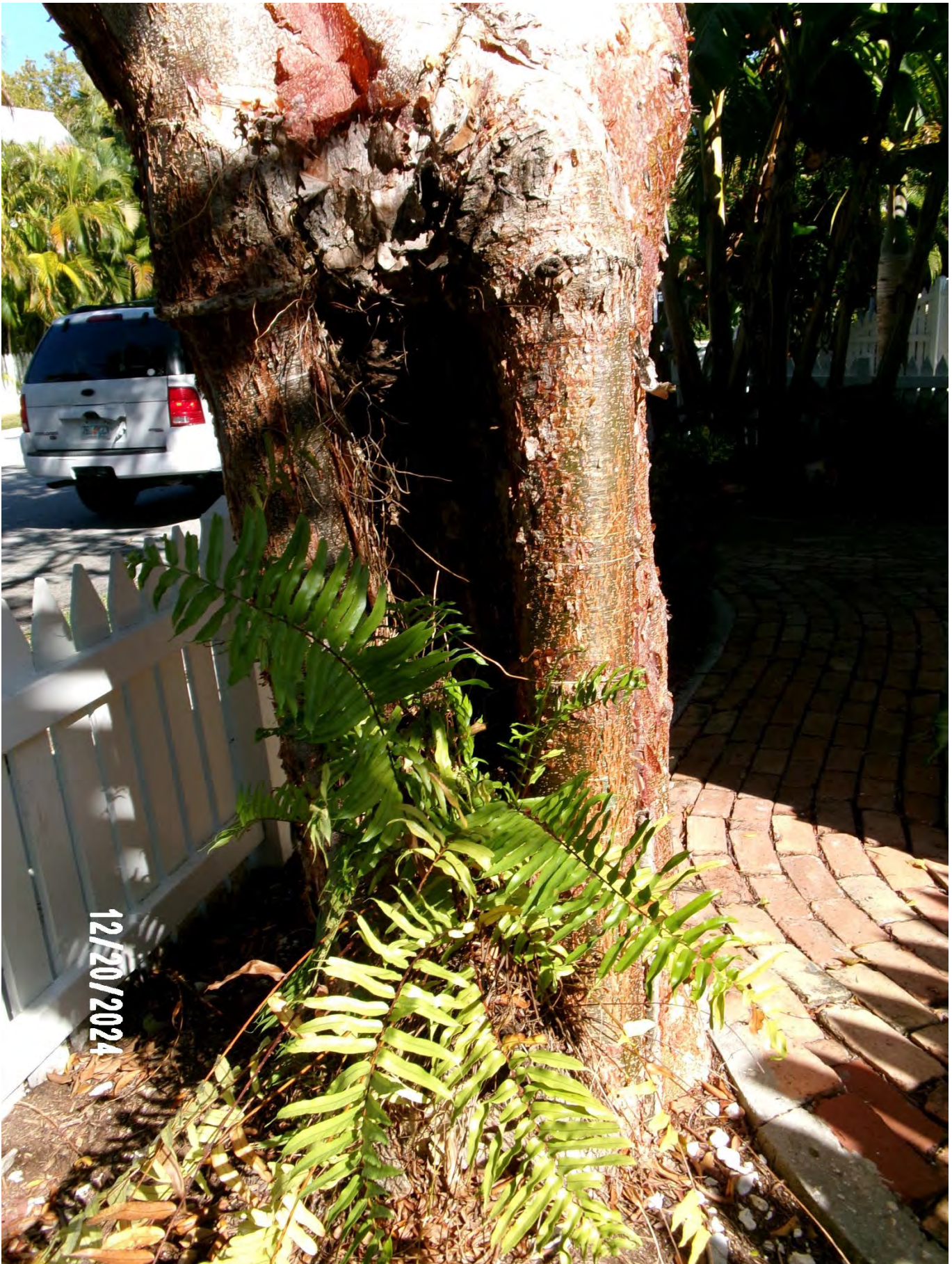
Photo of large decay area in main trunk. This appears to be an old injury.
