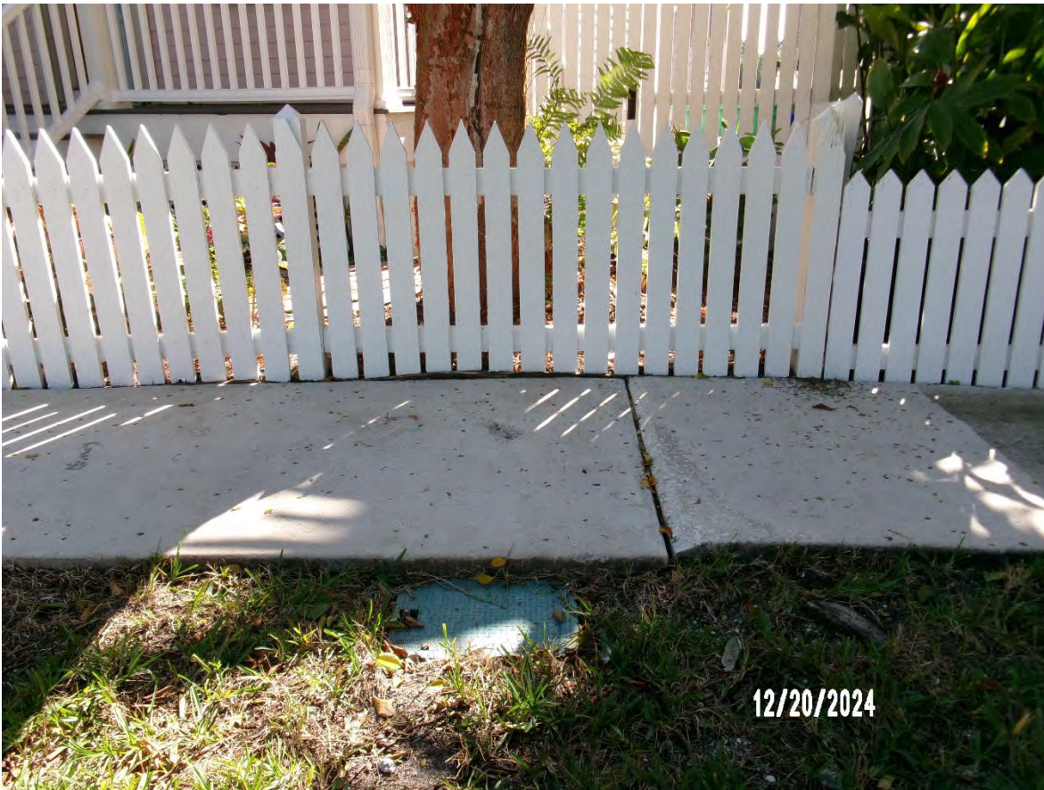
Photo showing base area of tree and impacts to public sidewalk.
