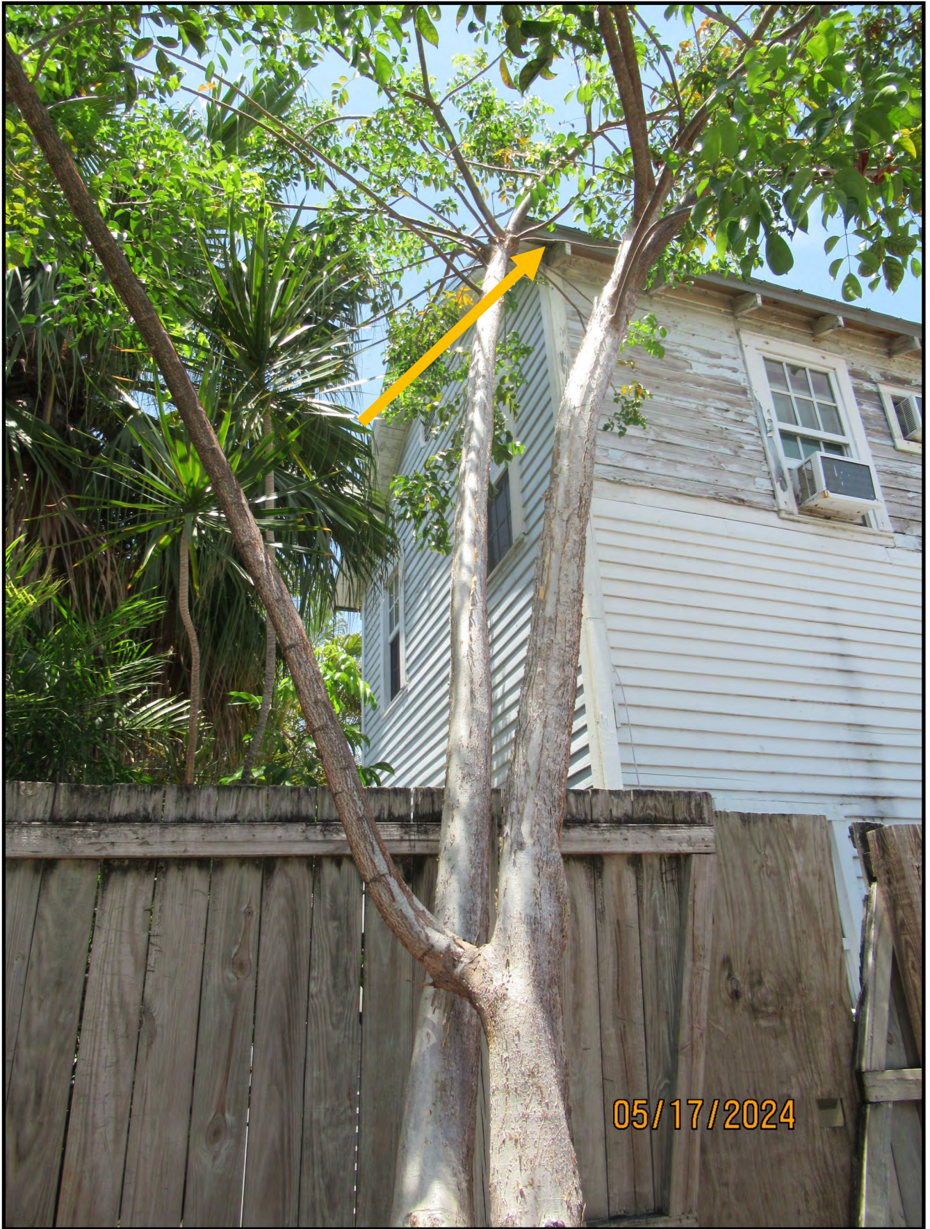
Codominant trunks of gumbo limbo, with alternate view of canopy encroaching the neighboring structure.
