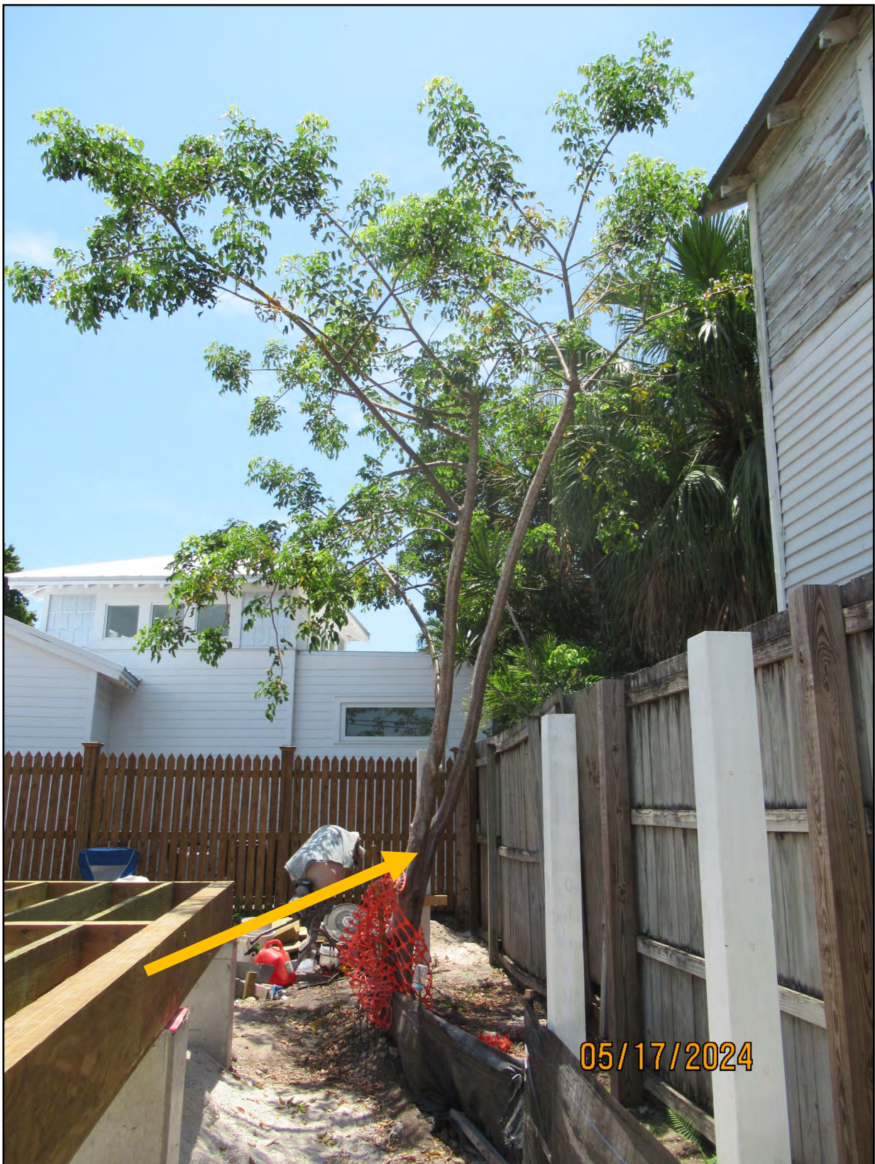
Gumbo limbo is a volunteer and leaning toward neighboring structure.
