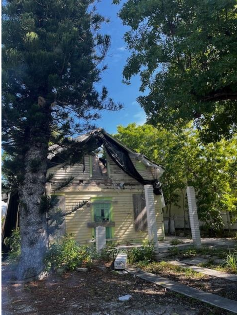
Current conditions at front (west) elevation. Notice caved on roof.
