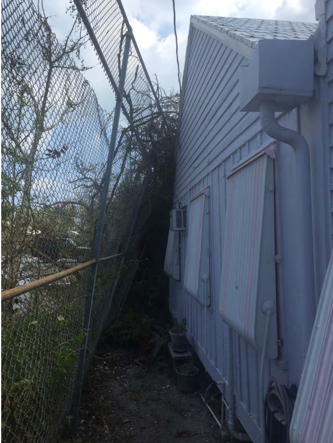
DAMAGED FENCE – HURRICANE IRMA SEPT. 2017
