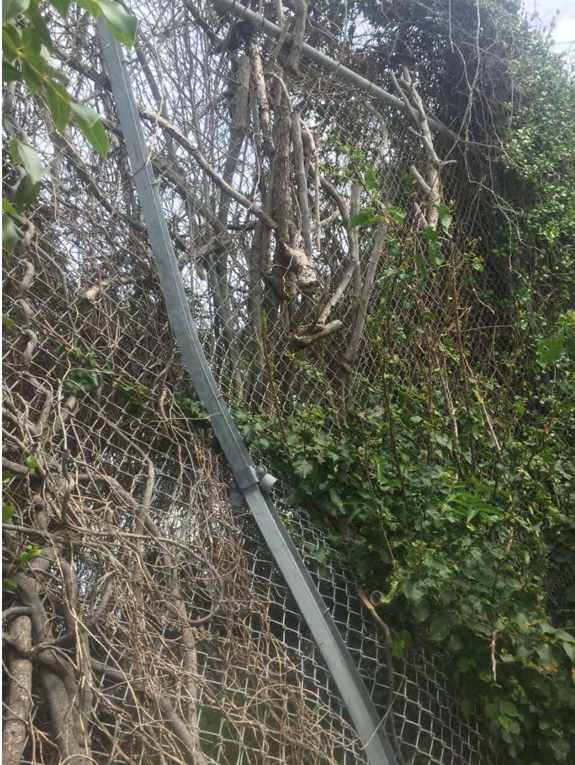
CURRENT CONDITION OF FENCE
