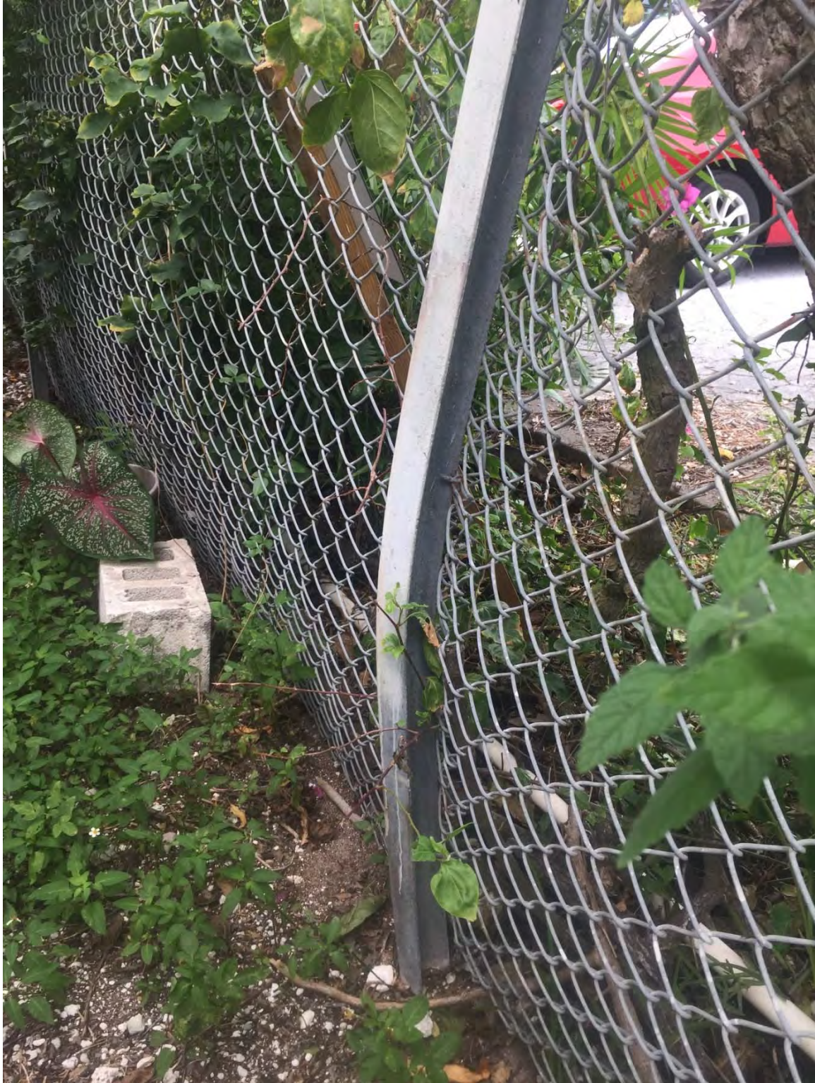
CURRENT CONDITION OF FENCE
