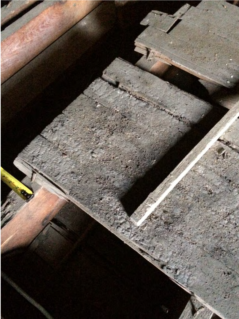
Photo: Existing Conditions; Charred Attic Flooring with Original 2" Joists
