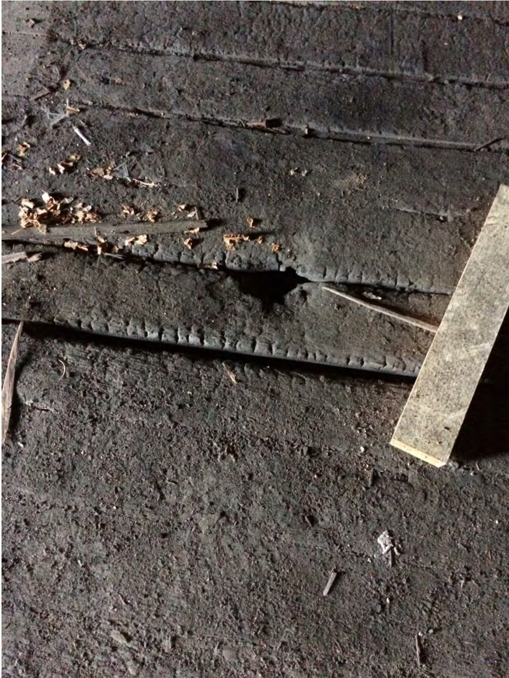
Photo: Existing Conditions; Charred Attic Flooring
