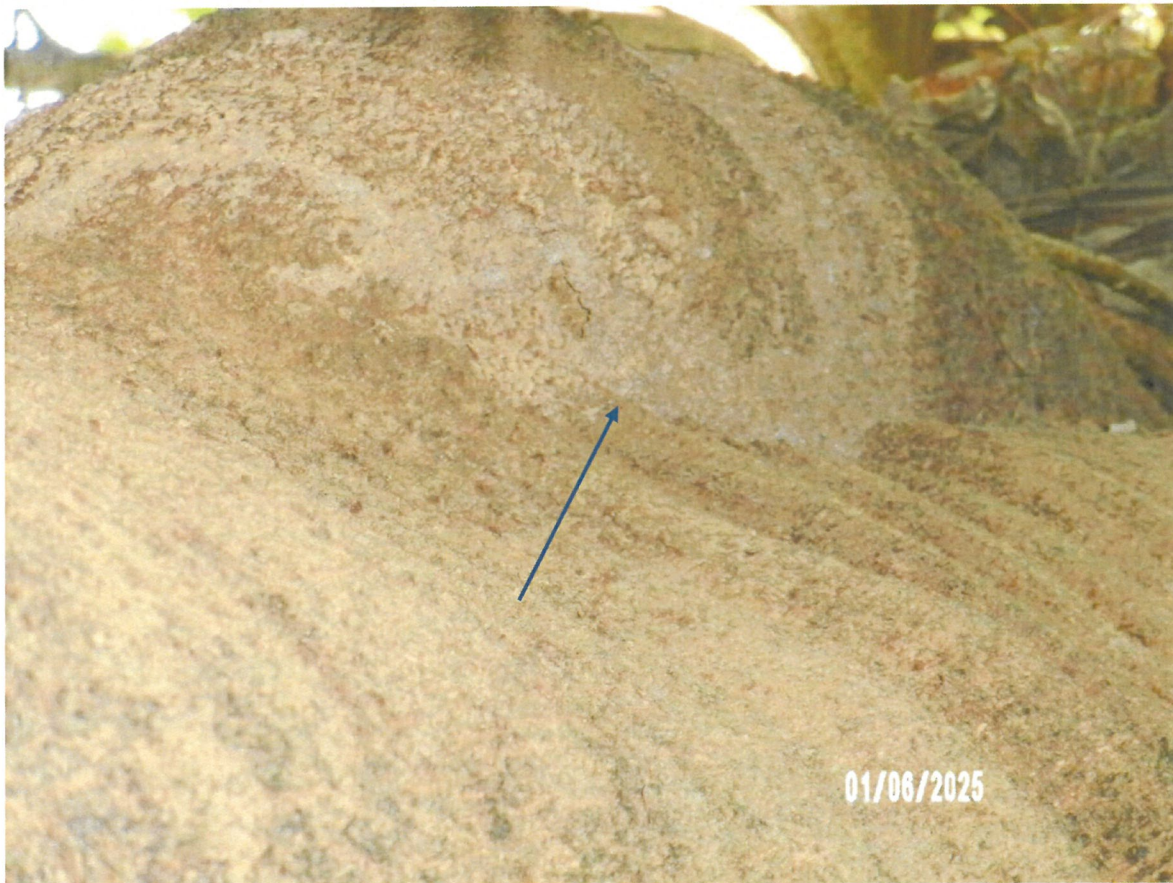
Close up photo of mud trail on trunk near base in back of tree-no live termites found.
