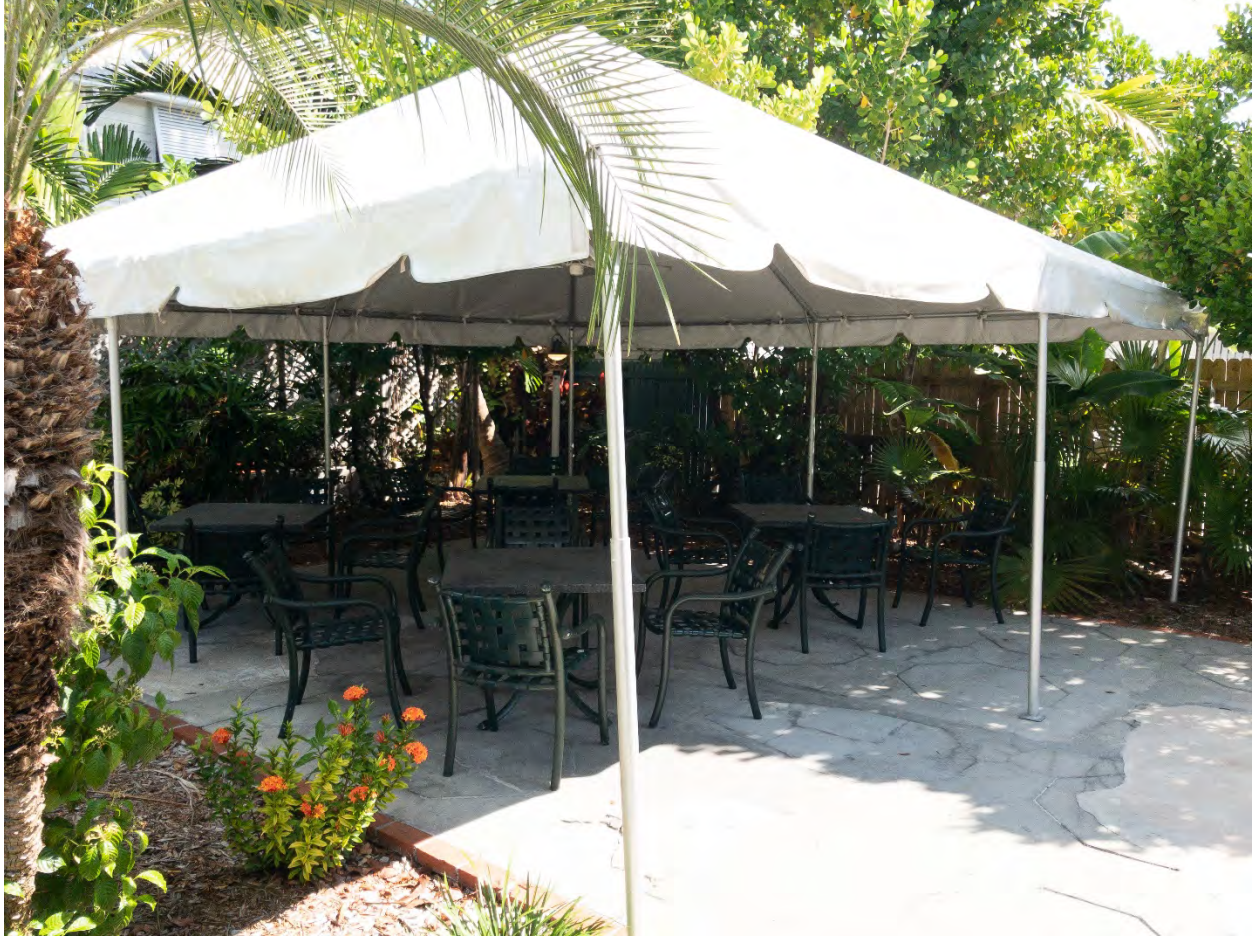
VIEW NORTHEAST – Demo of concrete pad and temporary tent structure and canvas.
