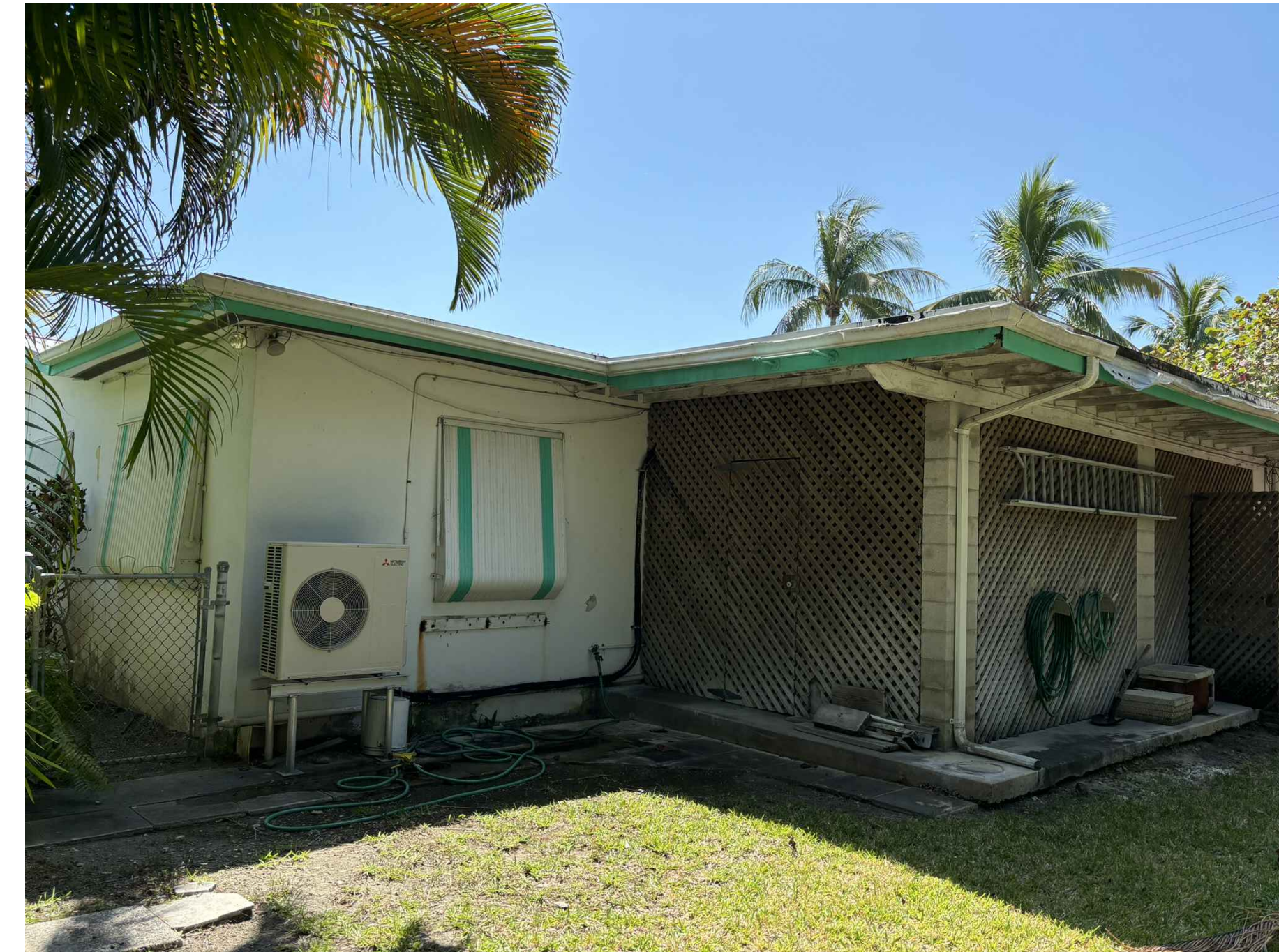
3 A8 VIEW OF THE BACK OF THE HOUSE (EXISTING NORTH ELEVATION) SCALE: N.T.S.
