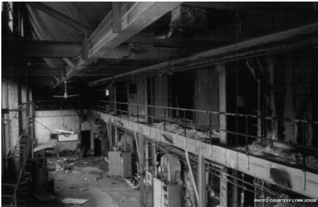
The interior of the Power Plant in 2000. Photo taken for the City Hospital Historic District National Register of Historic Places nomination.
