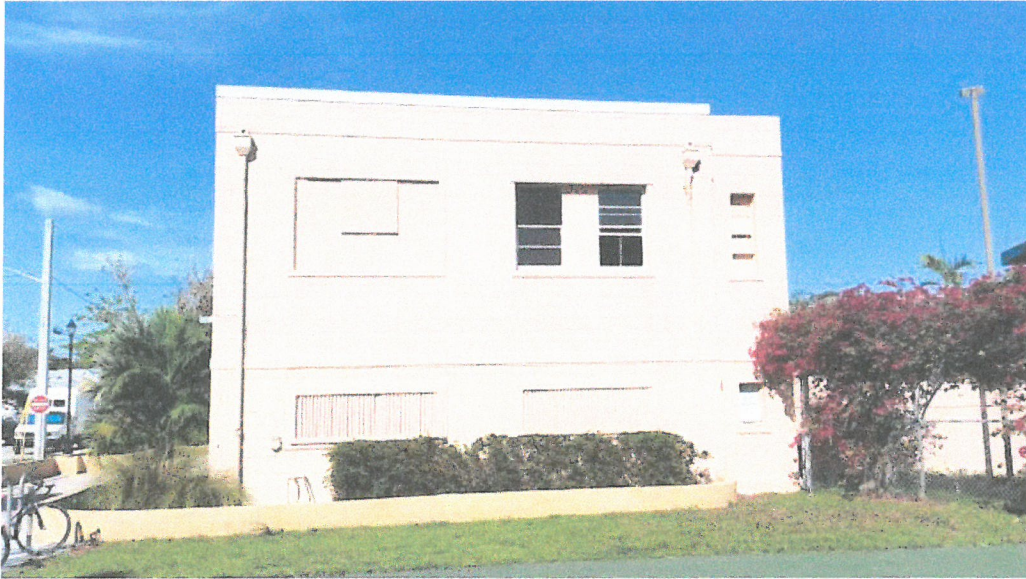
Figure 9. Right Side elevation. Undersized scuppers and damaged downspout on right side.
