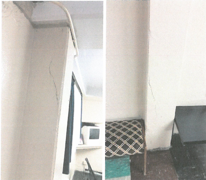
Figure 14. Concrete spalling of columns. Grade level interior spaces.
