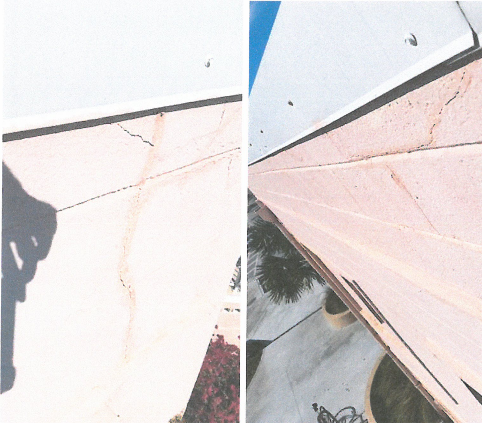
Figure 11 and 12. Cracks in CMU parapet wall.
