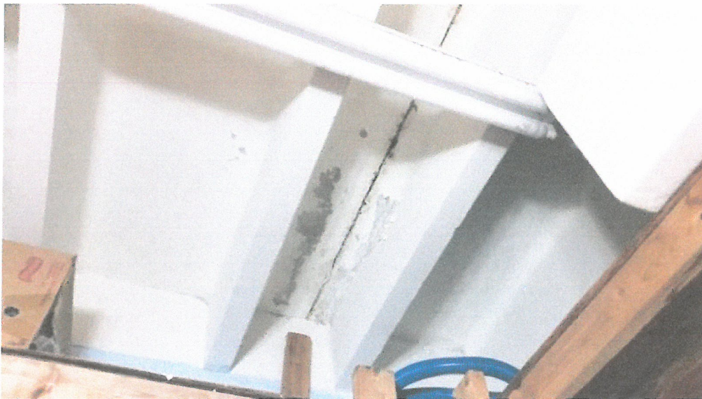
Figure 6. Signs of water leaks in the storage area.
