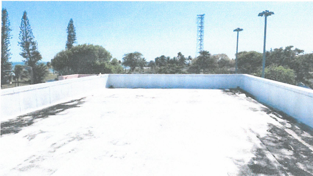
Figure 8. Roof surface with stains from algae grows in standing water.
