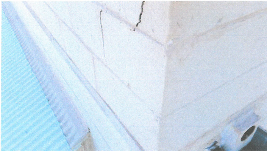
Figure 10. Cracks in CMU at the left back side.
