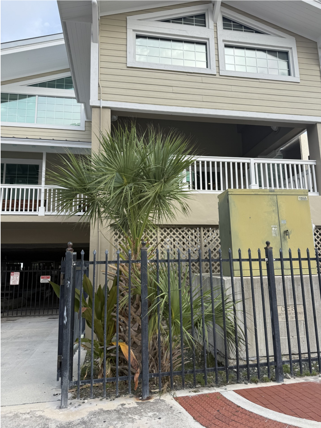
a Jamaica Caper used to be here. Not sure how it was lost but it is accounted for on the site plan/landscape plan. Currently there is a volunteer Sabal Palmetto.
