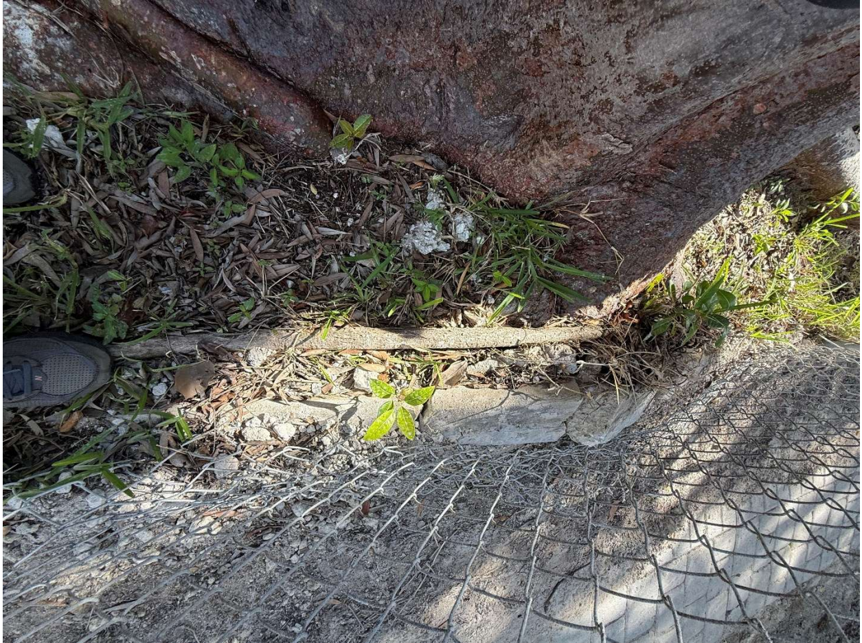
Tree's roots show severe girdling from fence line and other adjacent compaction factors.
