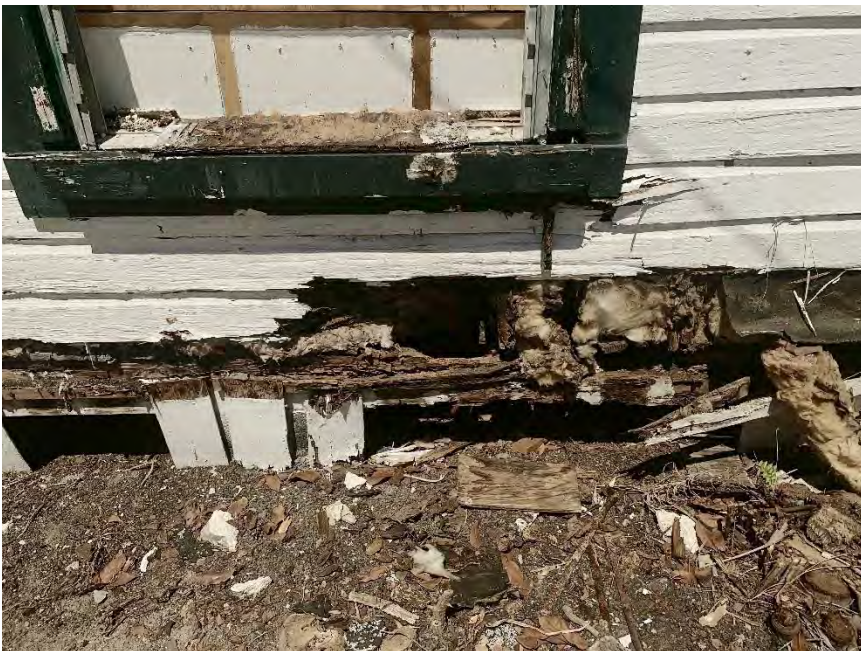
DETERIORATED FRONT SILL BEAM AT SIDE ADDITION
