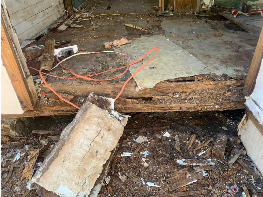
DETERIORATED REAR SILL BEAM AT SAWTOOTH
