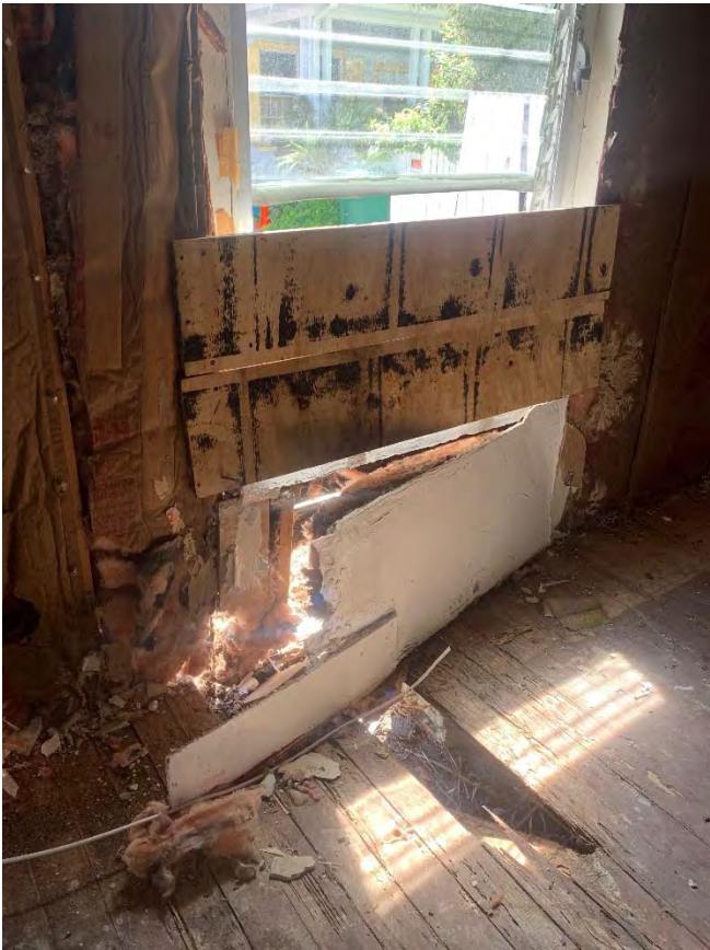
INSIDE OF DILAPIDATED SIDE ADDITION (TO BE REMOVED)
