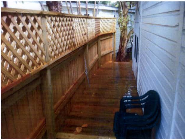
SOUTH WEST SIDE OF HOUSE LOOKING TOWARDS THE REAR RED TAGGED DECK & FENCE
