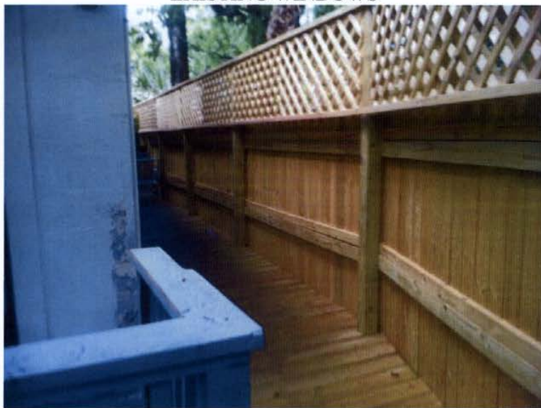
SOUTH WEST SIDE OF HOUSE LOOKING TOWARDS THE FRONT RED TAGGED DECK & FENCE
