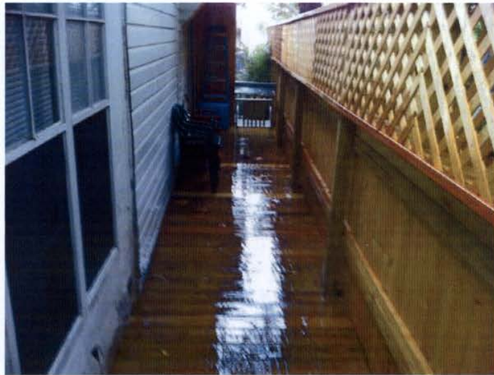
SOUTH WEST SIDE OF HOUSE LOOKING TOWARDS THE FRONT RED TAGGED DECK & FENCE
