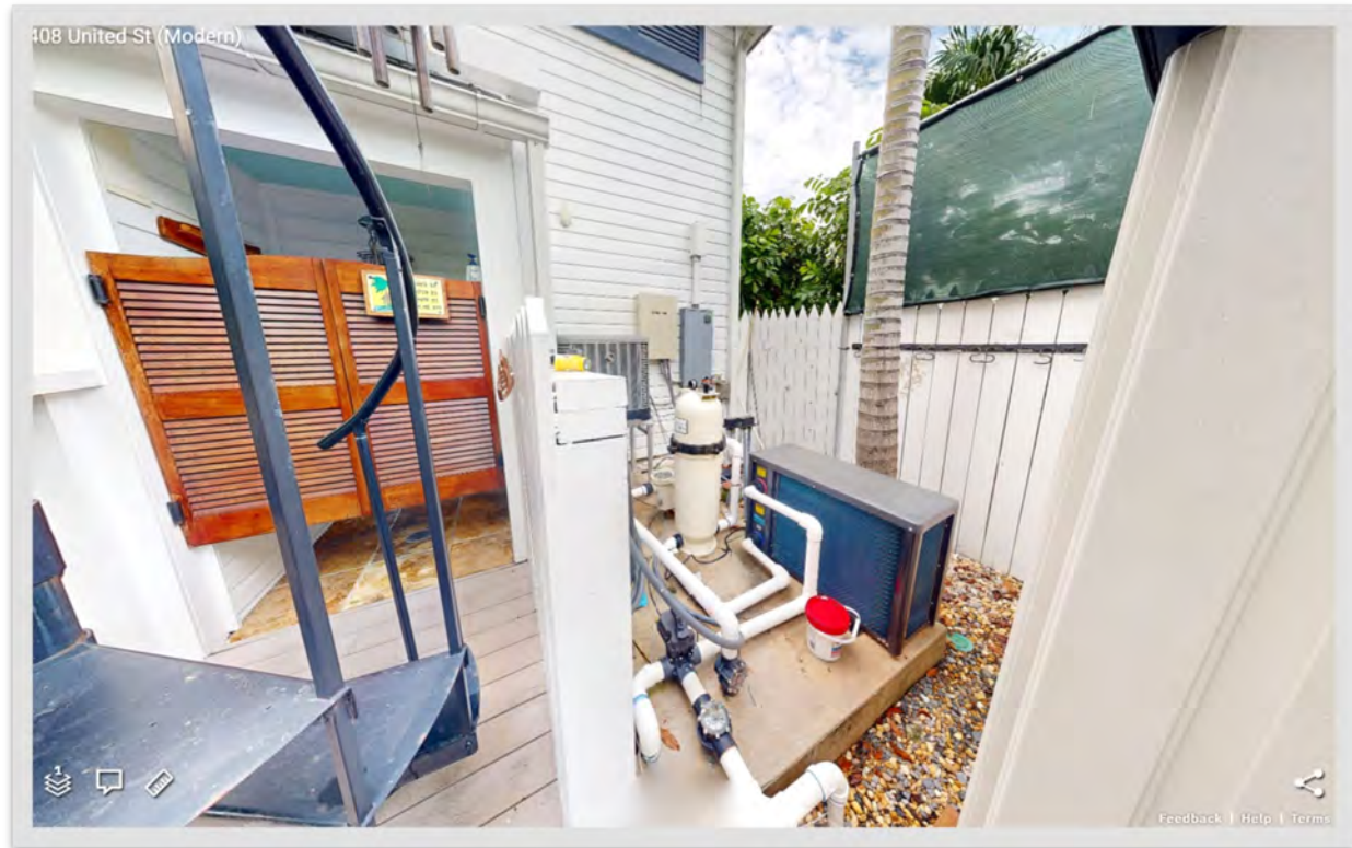
Concrete platform for pool equipment and AC unit.
