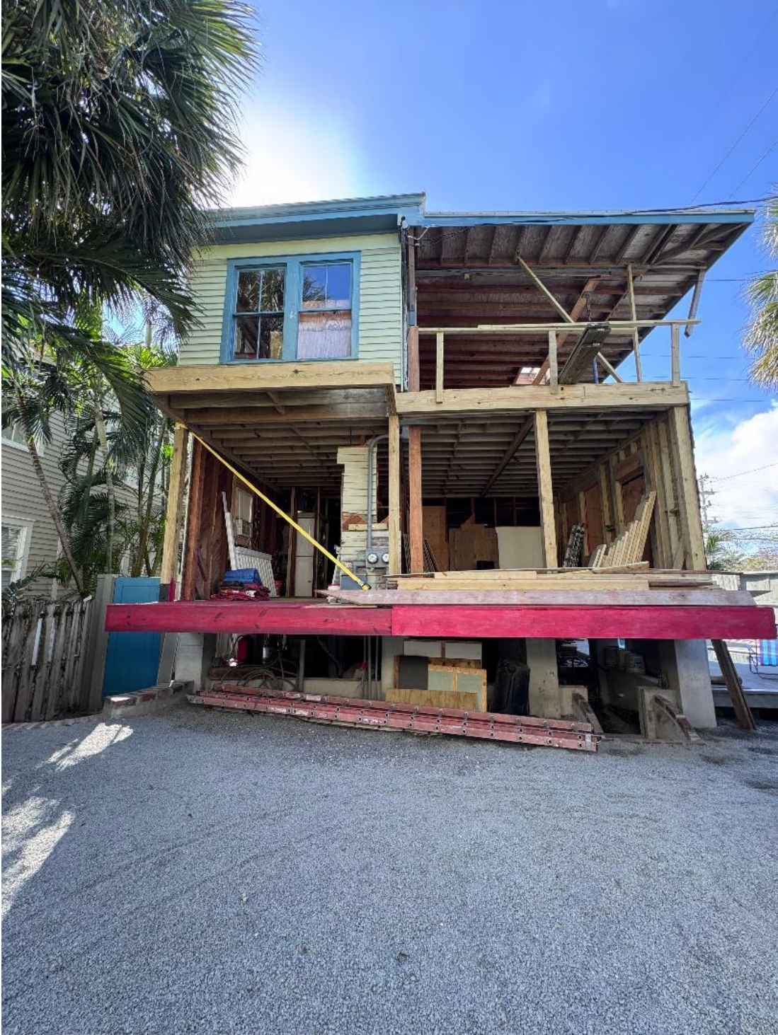
Rear of home view with upper porch demo completed with no replacement structure for 1 st floor rear wall or 2 nd floor porch ½ wall or screen
