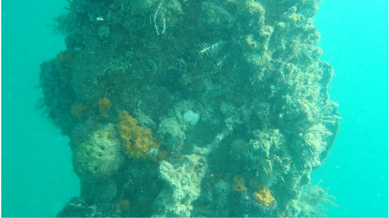
Photo 1. Typical piling at Mallory Pier with dense cover of sponges and invertebrates.
