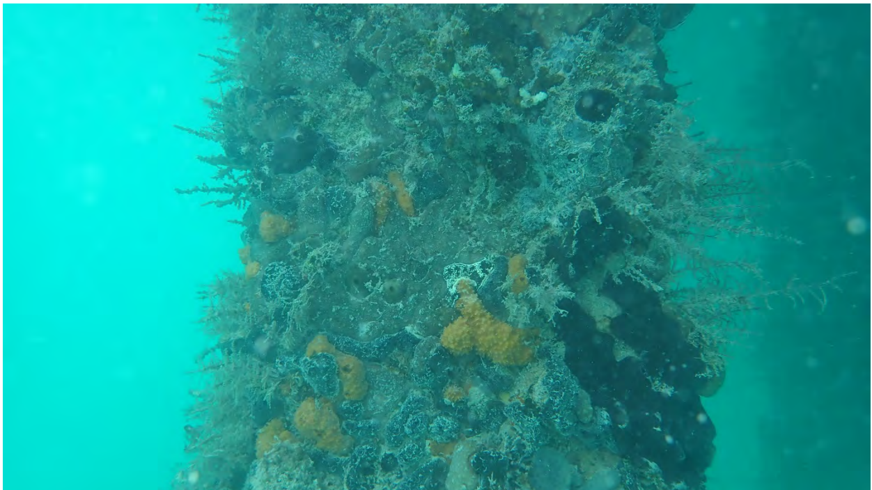
Photo 2. Typical piling at Mallory Pier with dense cover of sponges and invertebrates.
