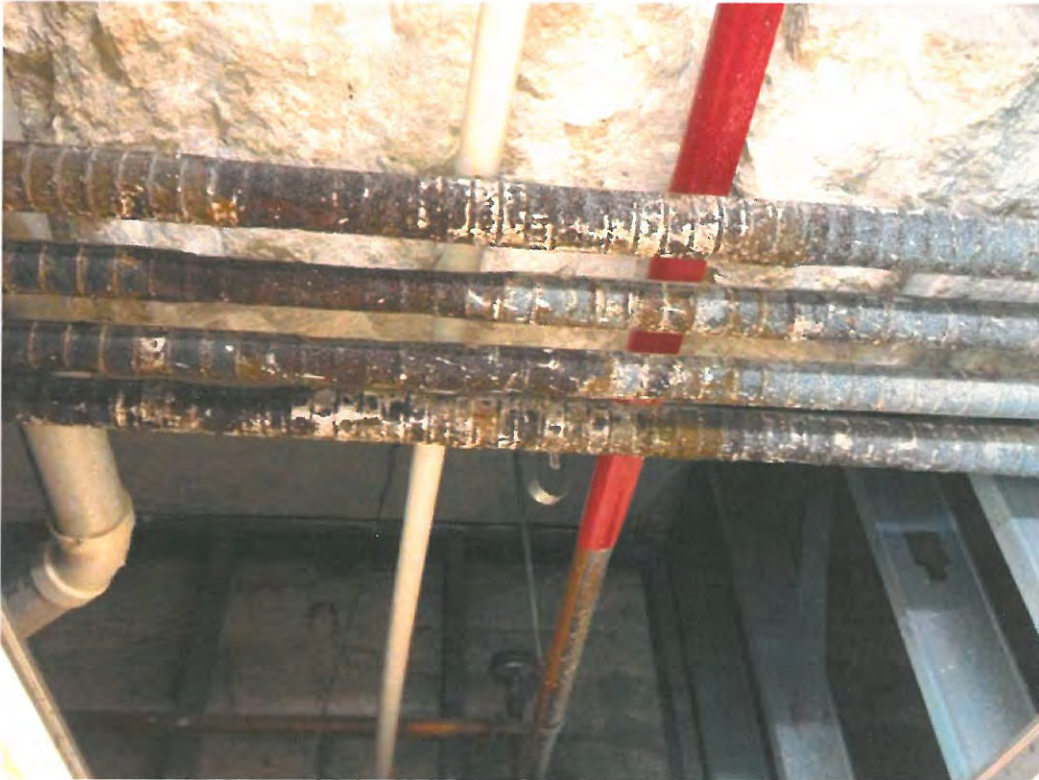
Note bottom of concrete 8" of concrete beam has been chipped away and rebar exposed
