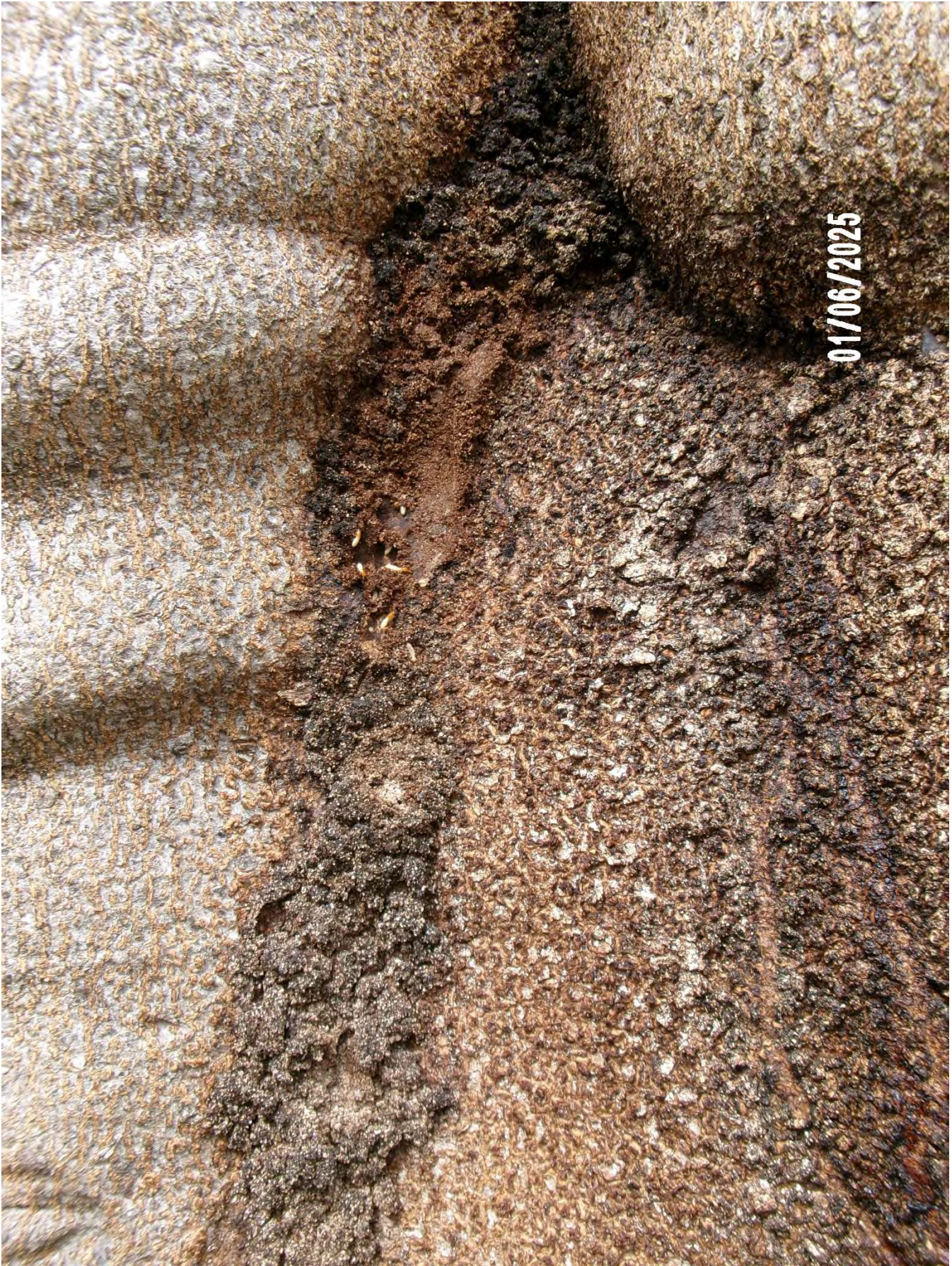
Active termites in mud trail on main trunk.
