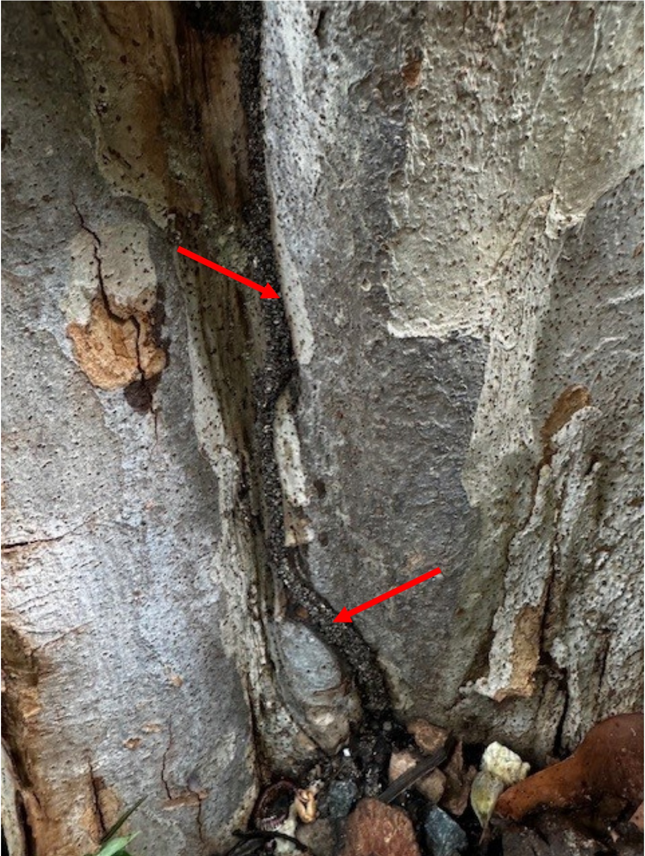
Asian subterranean termite "mud tube" visible in one area. The entire tree could not be inspected because it is on the fence.
