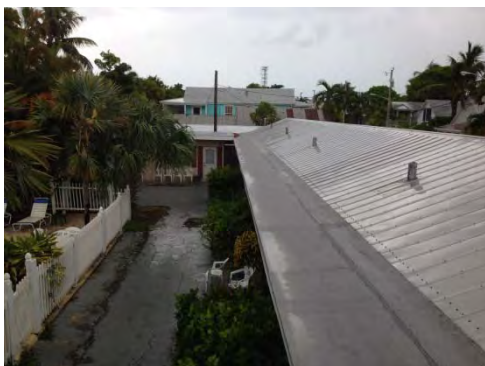
Photograph 6 showing inadequate fire separation between the L shaped building on the left and the adjacent structure. Note the non-code compliant egress windows.
