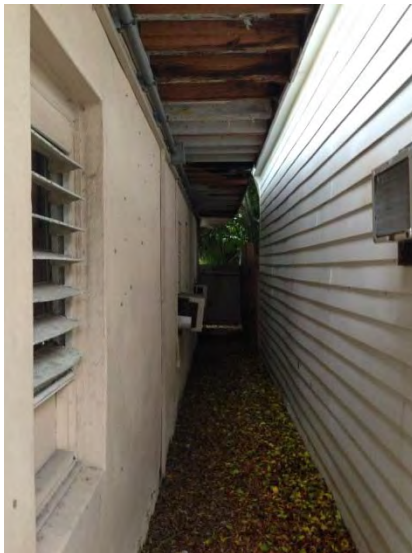
Photograph 5 showing the egress window blocked with an air conditioning unit.
