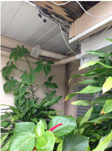
Photograph 9 of what appears to be an end of the line cleanout for the L shaped structure. The pipe appears to be made of cast iron and does not have a clean out box around it.
