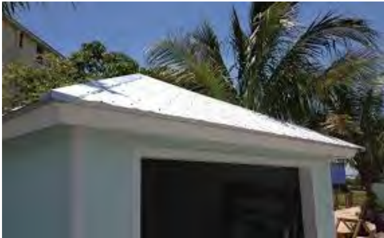
Low Slope Shed Roof over bathroom: Liberty Self Adhering - white in color
