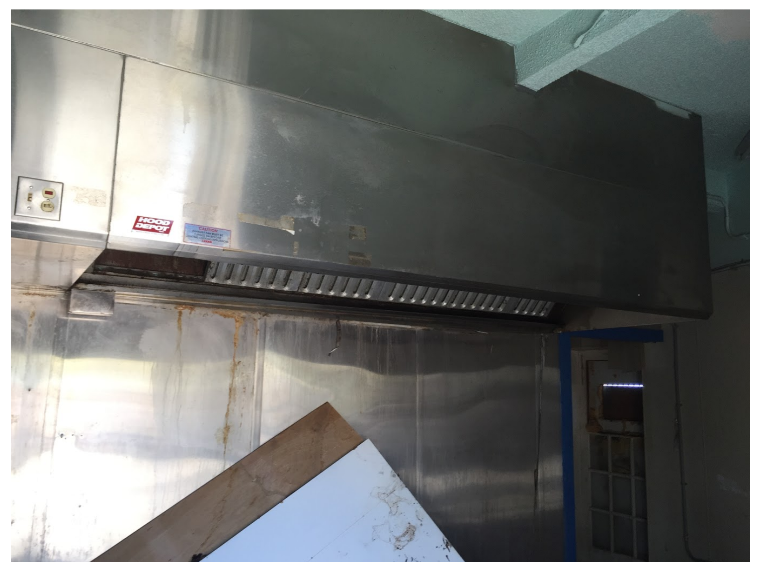
EXISTING CABLE HUT INTERIOR REMOVE ALL INTERIOR KITCHEN EQUIPMENT & NON HISTORIC MATERIALS
