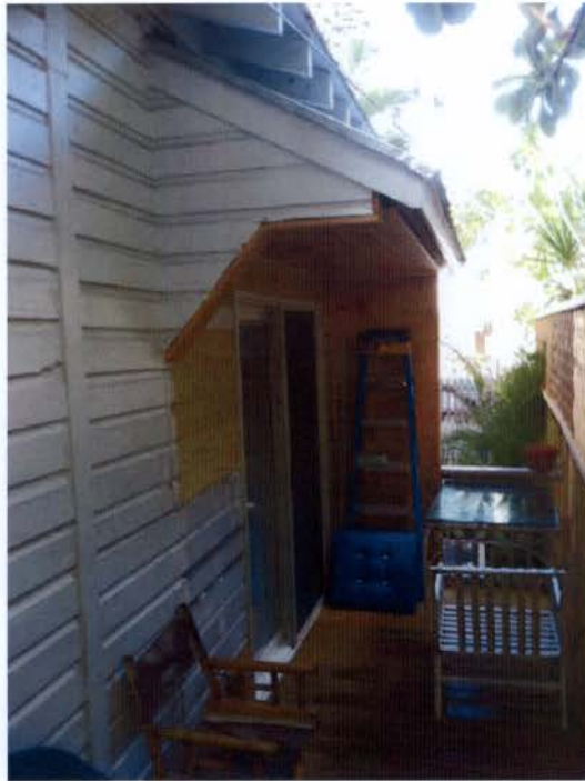
SOUTH WEST SIDE OF HOUSE LOOKING TOWARDS FRONT AREA WHERE SHED WAS REMOVED, ROOF STRUCTURE TO REMAIN
