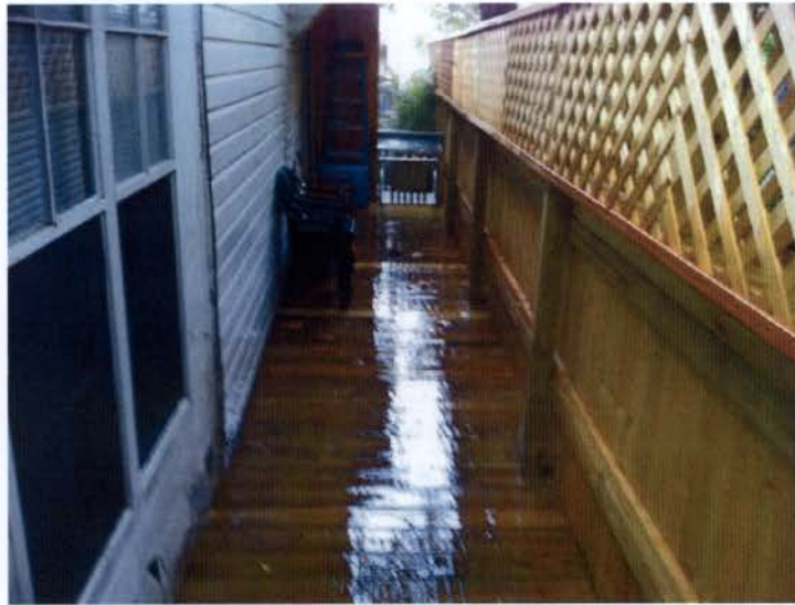
SOUTH WEST SIDE OF HOUSE LOOKING TOWARDS THE FRONT RED TAGGED DECK & FENCE
