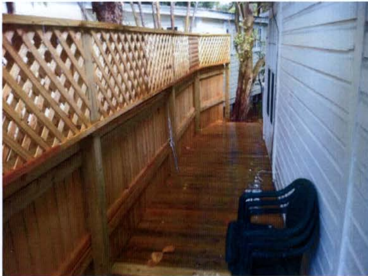
SOUTH WEST SIDE OF HOUSE LOOKING TOWARDS THE REAR RED TAGGED DECK & FENCE
