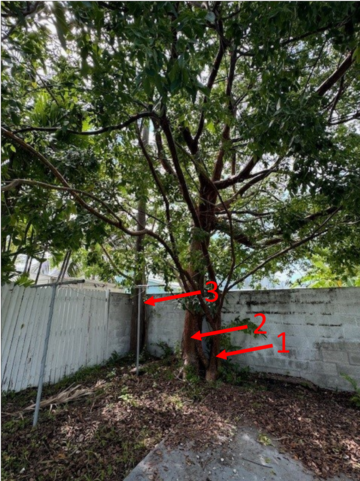
A closer view of the trees (three gumbo limbos) being requested for removal. The trees are causing damage to the cement fence and are dangerously close to the electric lines.
