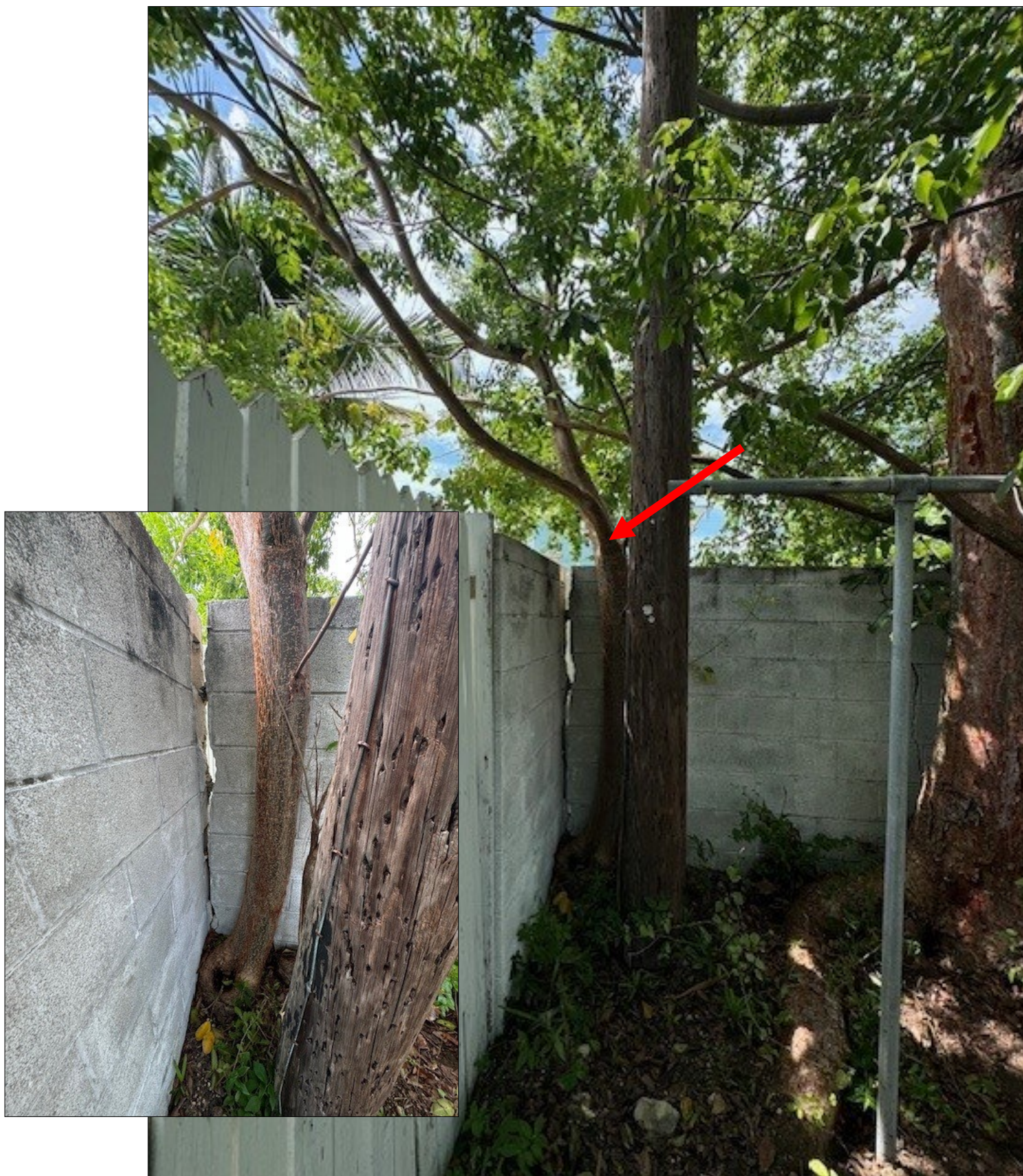
The third gumbo limbo tree is growing behind the electric pole, pushing into the cement block wall and has busted the corner open.
