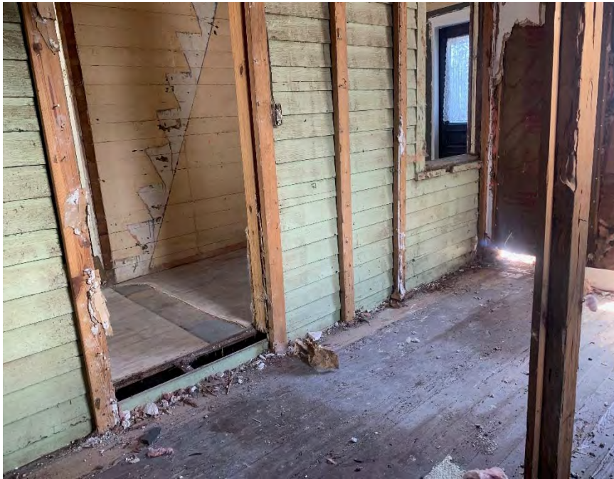
WEST WALL OF ORIGINAL HISTORIC STRUCTURE TO BE EXPOSED WITH REMOVAL OF WEST ADDITIONS
