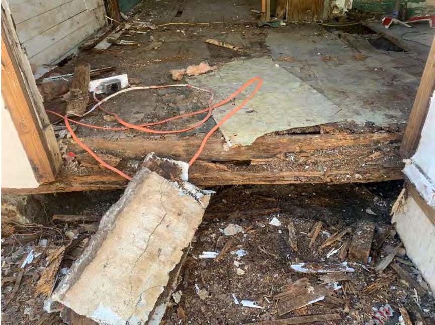
DETERIORATED REAR SILL BEAM AT SAWTOOTH
