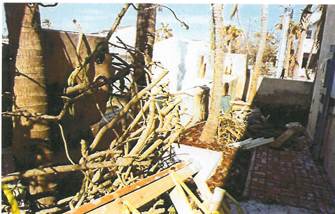
Photo 9 - View looking east at the area behind the seawall on the subject property after a storm showing the damaged walkway and landscape.
