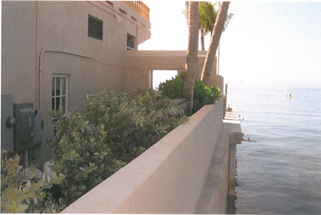
Photo 5 - View looking South from Southernmost Point showing the existing concrete cap and top wall of the vinyl sheet pile wall at the project area.
