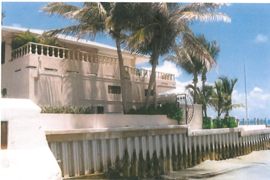
Photo 2 - View looking East from the Southernmost Point Buoy showing the existing vinyl sheet pile wall and nearby house at the area of concern.
