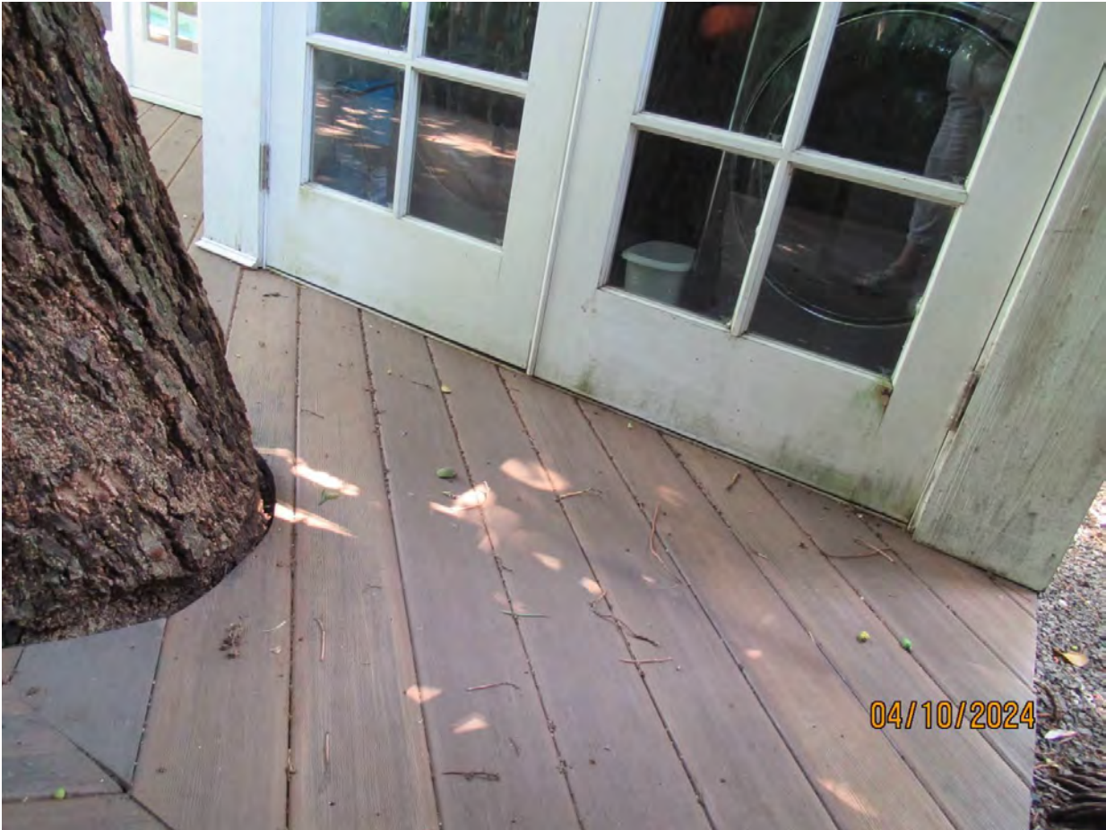
Photo of base of tree in relation to laundry door.
