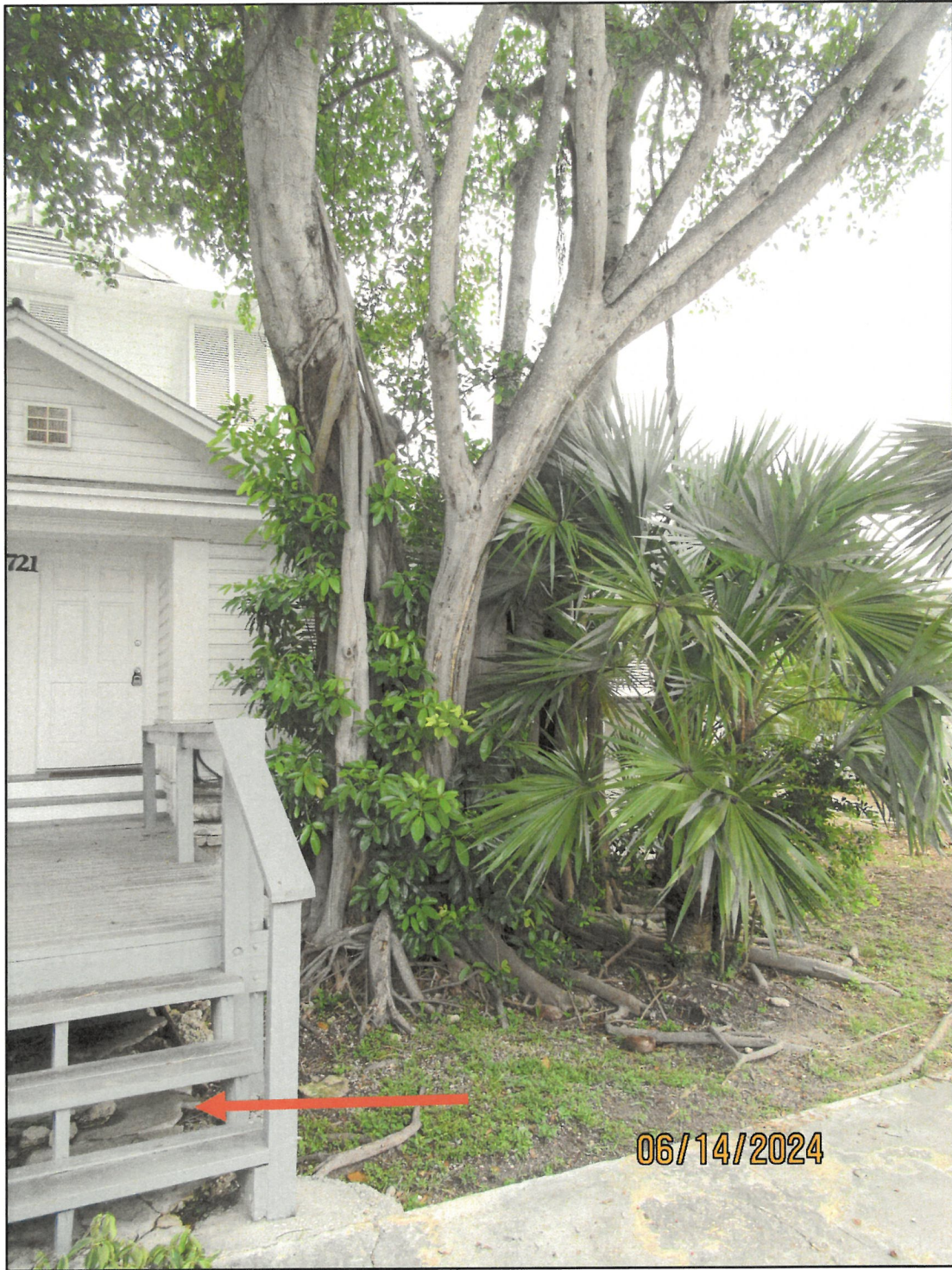
The tree is growing on the front right corner of 721 Waddell. At current, it is behaving and not causing visible significant damage. Appears original porch was built over with wood and lifted.
