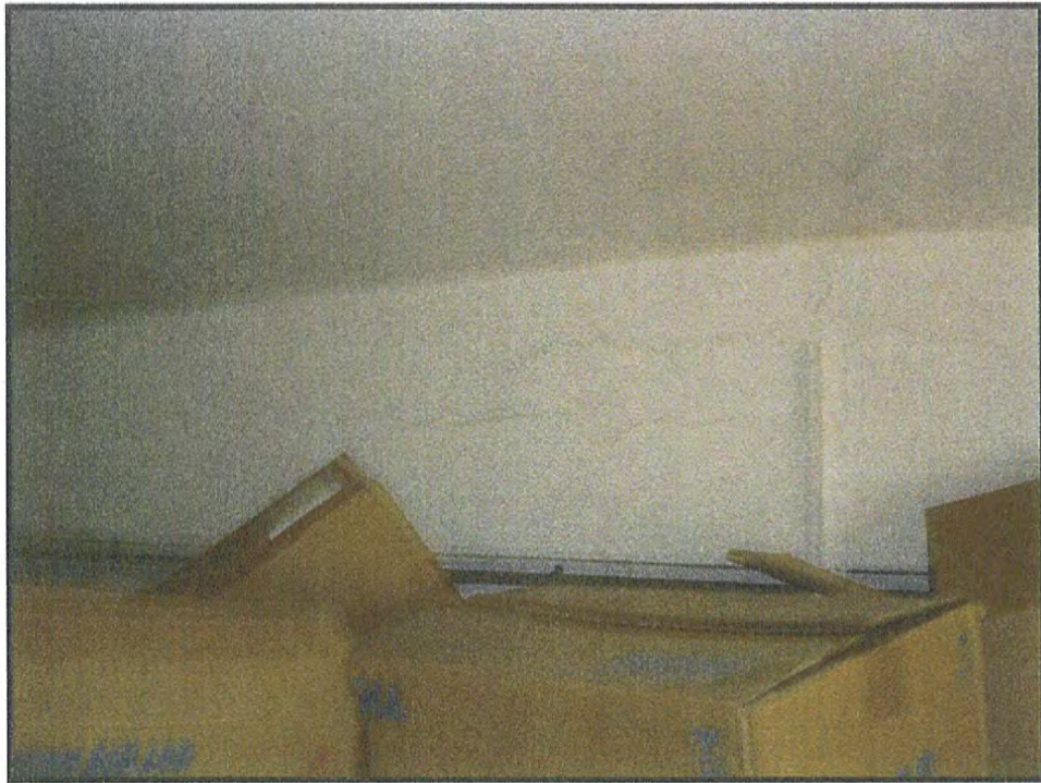
Photo No. 23 - Horizontal crack outlining the delamination along the side face of 2 nd level transverse support beams. Condition is typical for beams within service areas.
