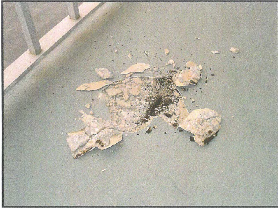
Photo No. 31 - Spalling due to lack of cover along top side of balcony slab typically found North of column line 7.
