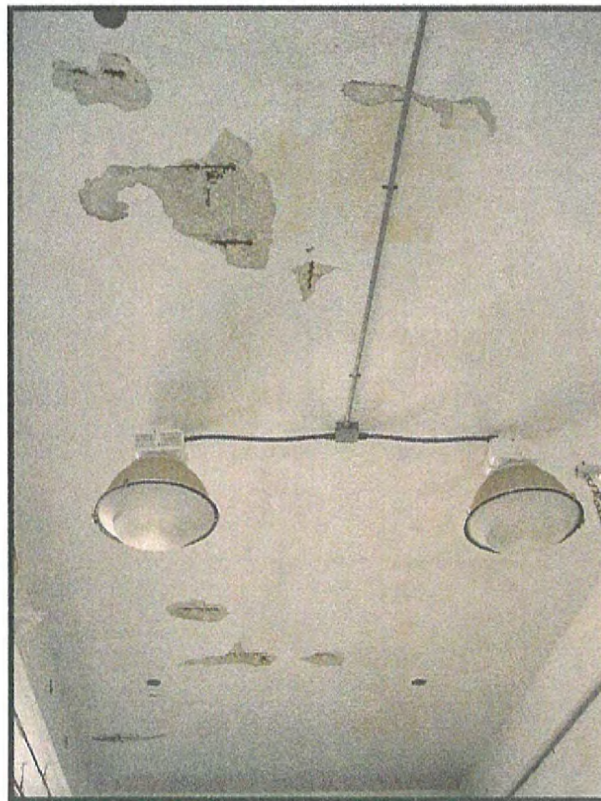
Photo No. 26 - Delaminations along underside of second level slab typically found in all six service bay areas.
