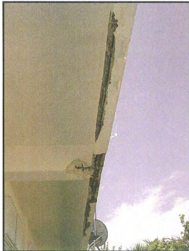
Photo No. 14 - Concrete spall with exposed corroded reinforcement on bottom face of balcony edge beam along the West side of building.
