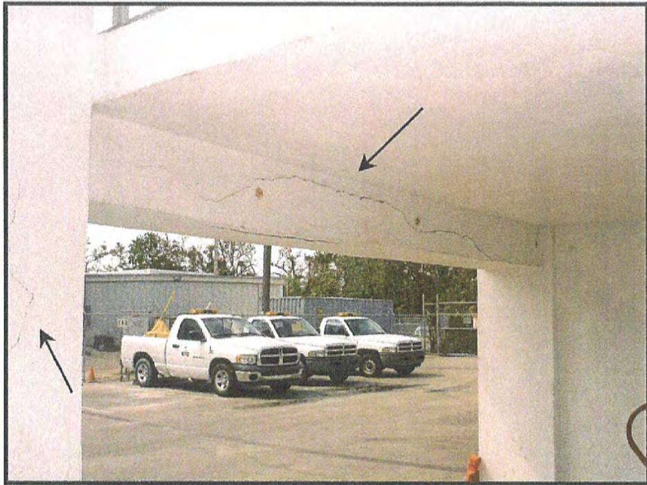
Photo No. 5 - Delaminations along concrete support beams and columns for North exterior stair.
