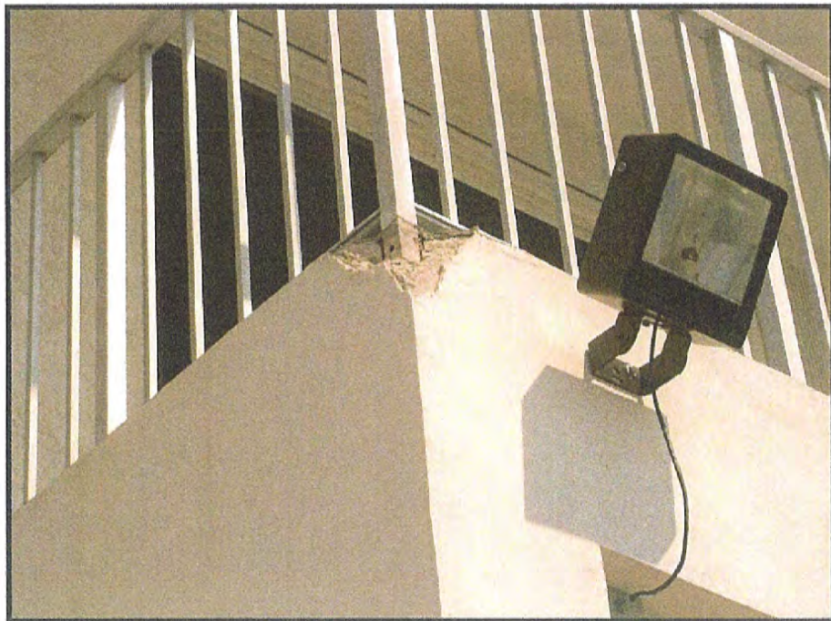
Photo No. 4 – Exposed balcony post rail at Southeast corner of building.
