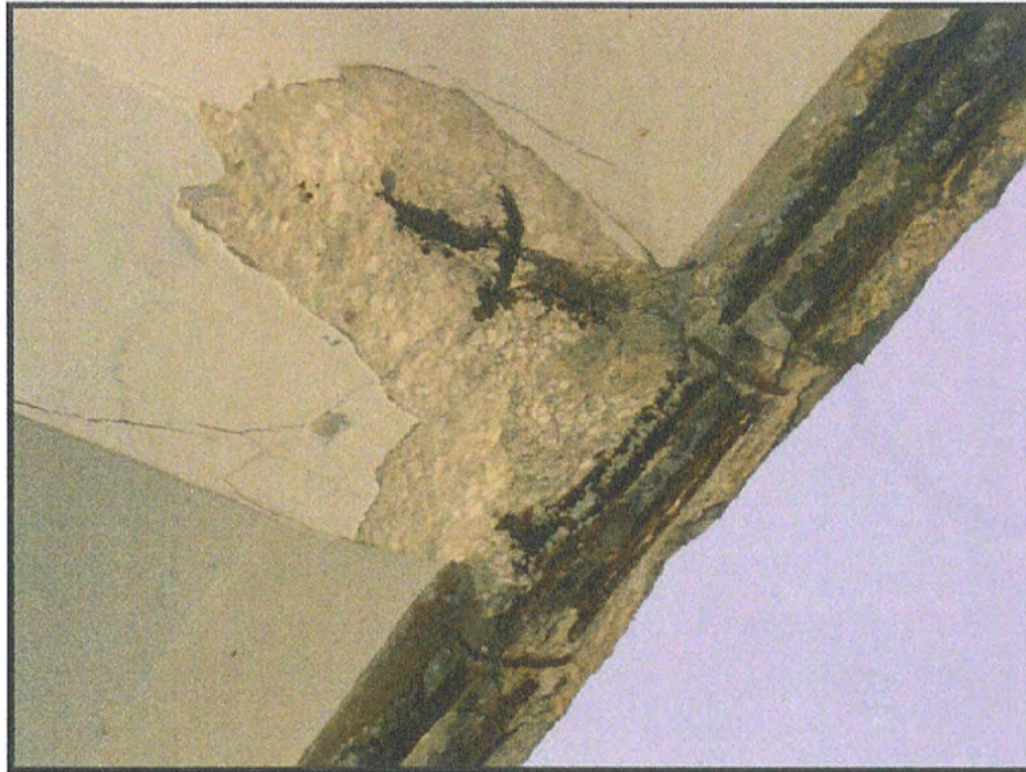
Photo No. 15 – Close up of spalled area along balcony support beam.
