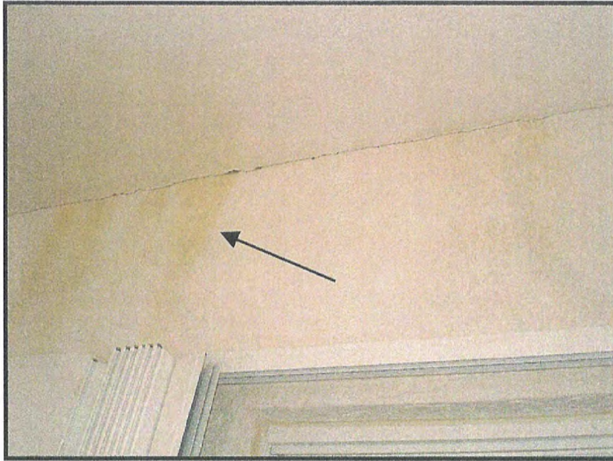
Photo No. 1 - Water stains along East wall below eave of roof.
