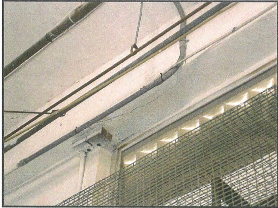
Photo No. 29 - Horizontal crack outlining the delamination along the side face of 2 nd level perimeter support beams. Condition is typical for beams within service areas.
