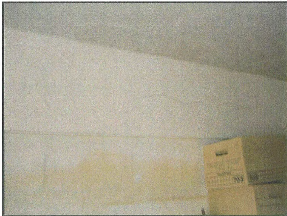
Photo No. 24 - Horizontal crack outlining the delamination along the side face of 2 nd level transverse support beams. Condition is typical for beams within service areas.
