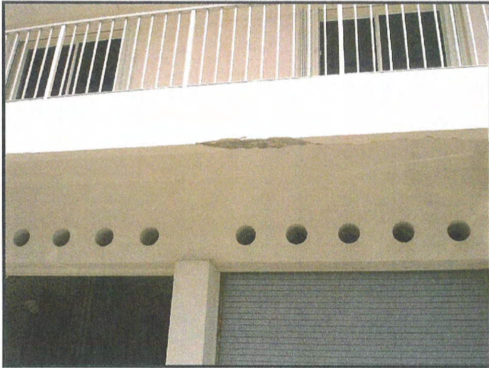
Photo No. 17 – Spalling on bottom face of balcony edge beam along the East side of building.
