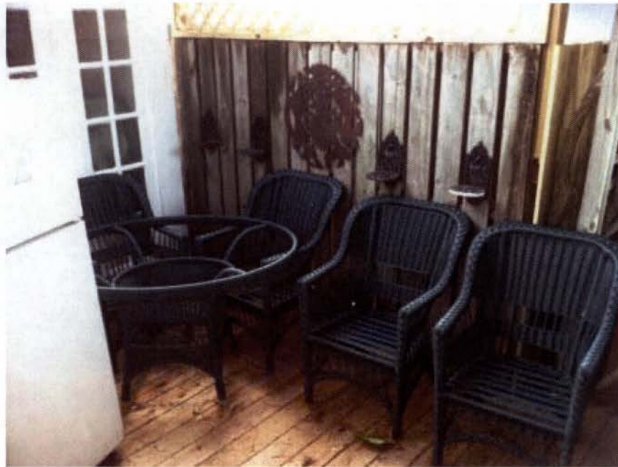
REAR DECK TO BE REPLACED
