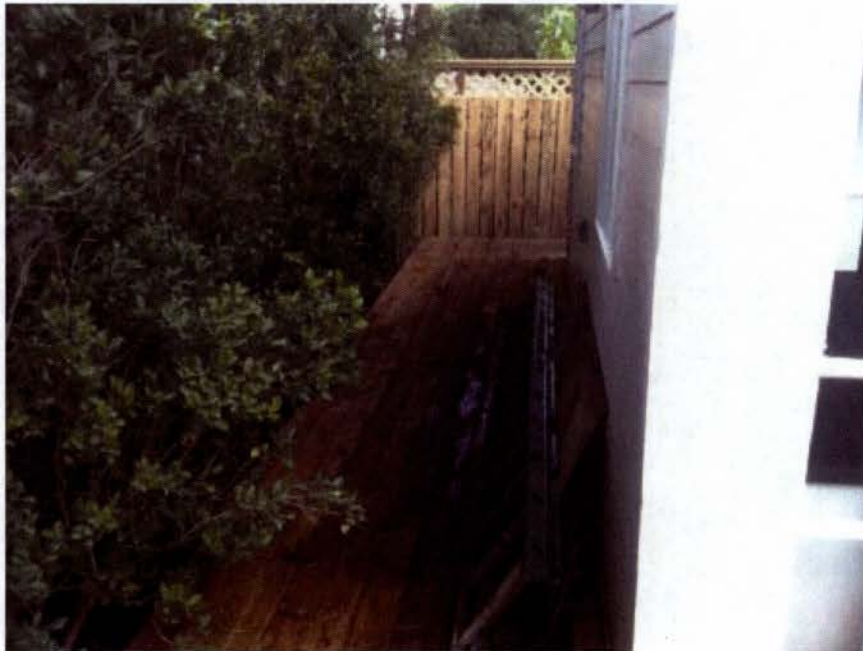
REAR DECK TO BE REPLACED
