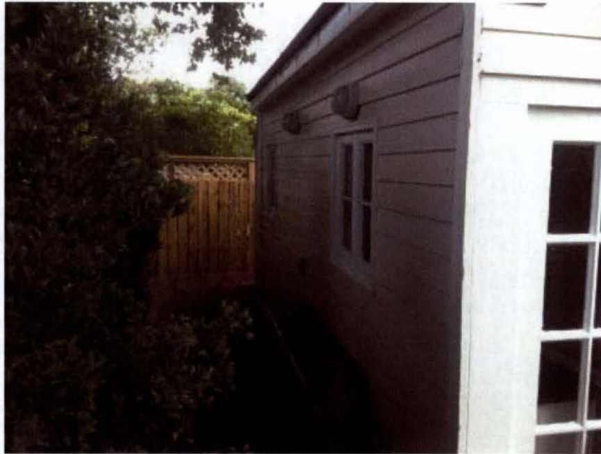
REAR DECK TO BE REPLACED
