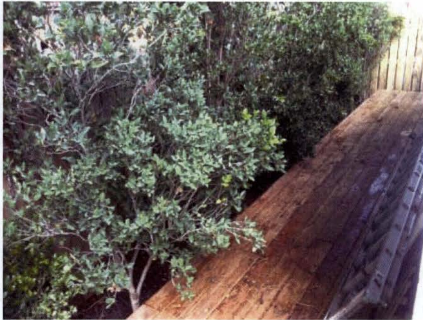
REAR DECK TO BE REPLACED
