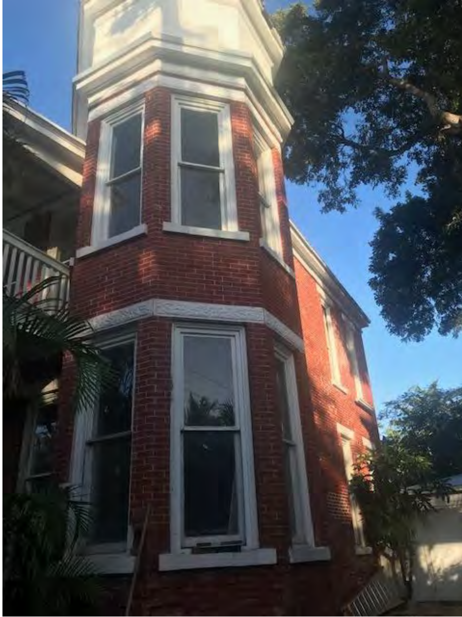
Current conditions front view of turret as removal of layers of paint has finished. New repointing at the upper portion of the turret.
