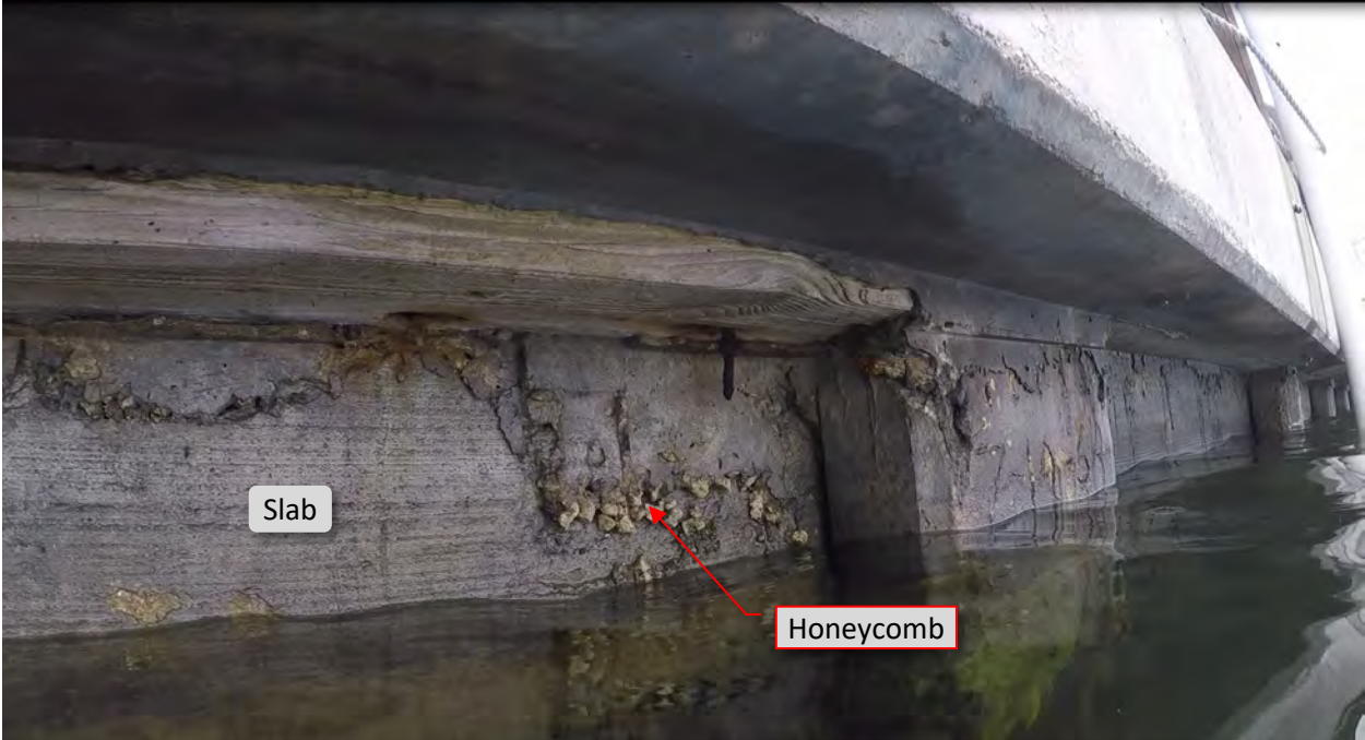
Figure 30: S7. STA 3+21 - 3+23. Honeycomb at slab.
