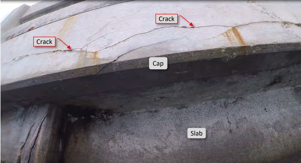
Figure 136: C12. STA 6+14 - 6+21. Crack at cap's bottom and vertical faces.
