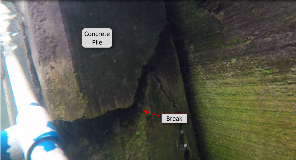
Figure 62: P23. STA 4+28. Break/spall at east flange at pile. Loss of concrete.
