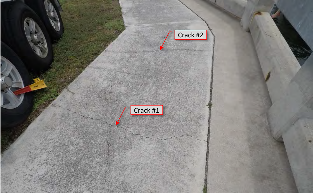
Figure 2: STA 6+00 - 6+10. Cracks in concrete slab to sidewalk. Closer view of the cracks.
