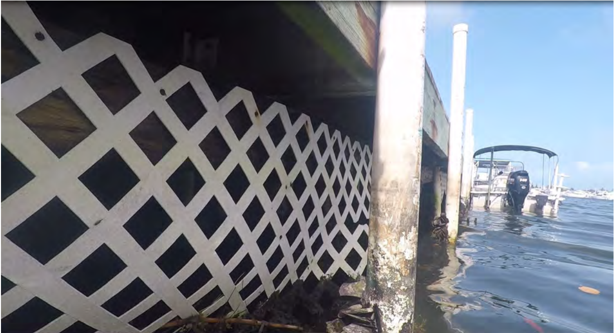
Figure 8: STA 0+40. Northeast direction view. Obstructions in front of seawall.
