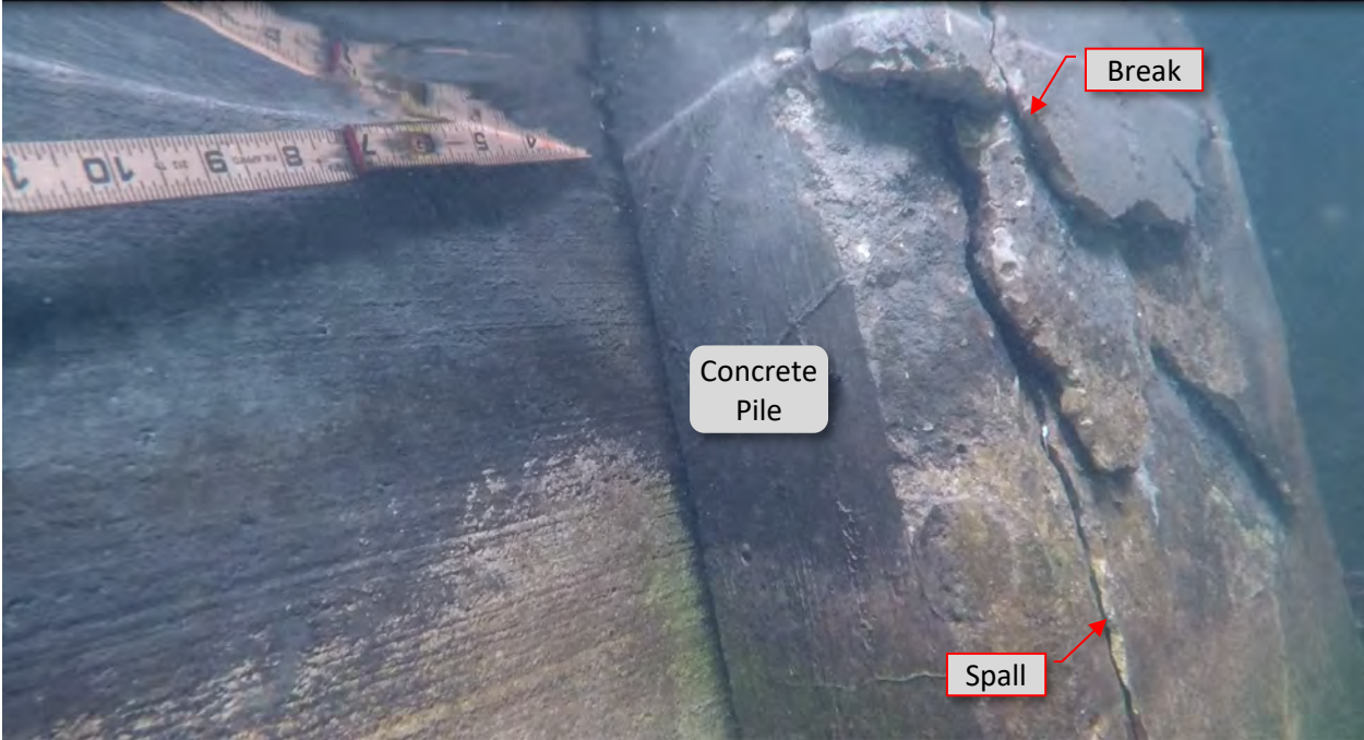
Figure 60: P22. STA 4+20. Break/spall at west and east flanges at pile. Loss of concrete. Underwater view.
