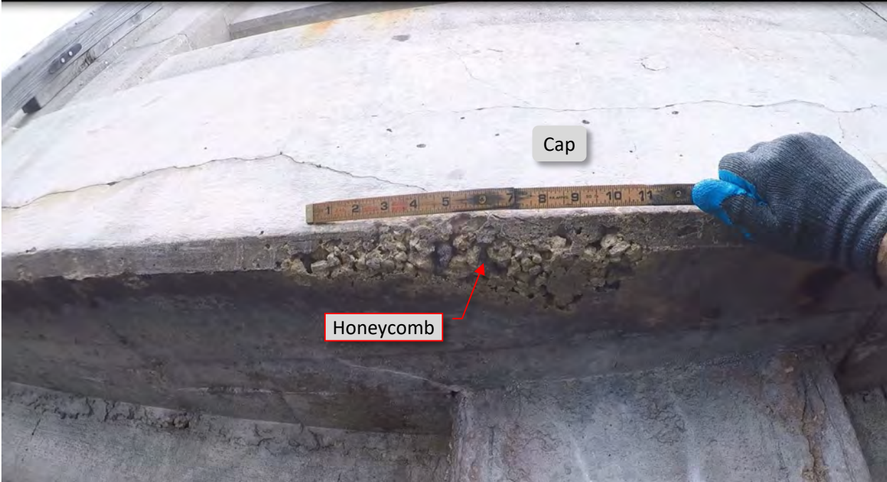
Figure 126: P43. STA 5+93 - 6+00. Honeycomb area at cap's bottom edge.
