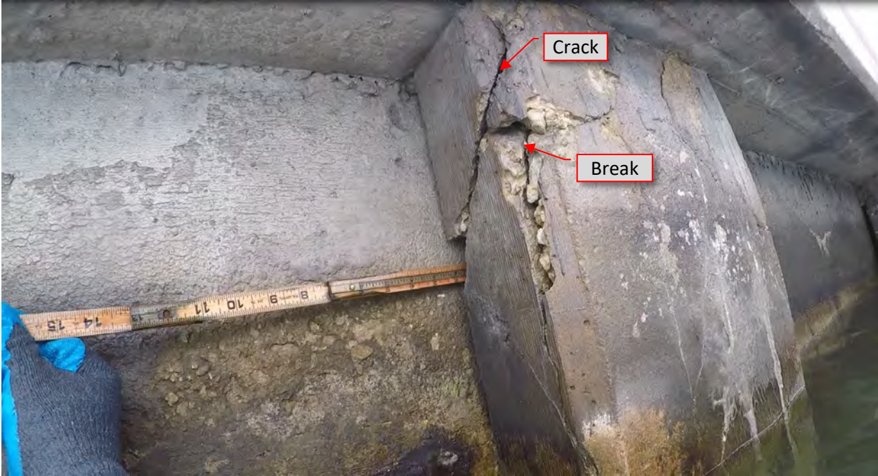
Figure 99: P34. STA 5+30. Cracks/spalls at top of pile west flange and loss of concrete.
