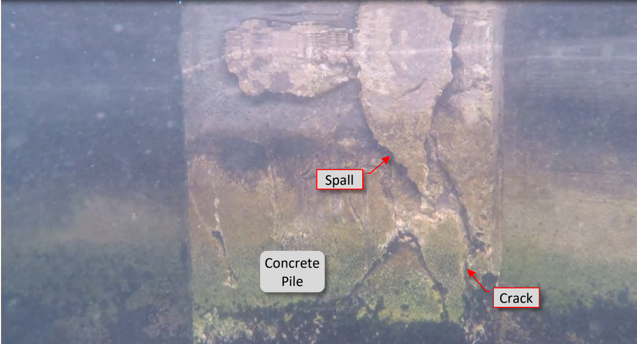
Figure 29: P11. STA 3+16. Crack/spall at east flange at pile. Underwater view.
