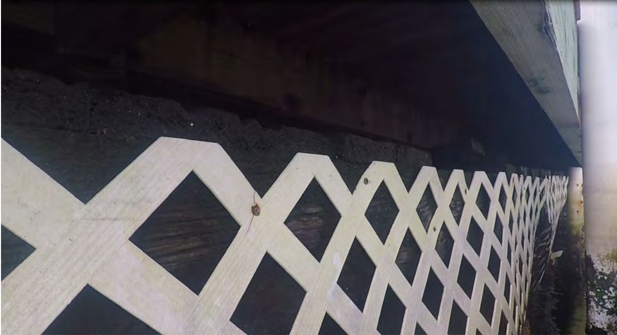
Figure 13: STA 0+80. Northeast direction view. Obstructions and debris in front of seawall.
