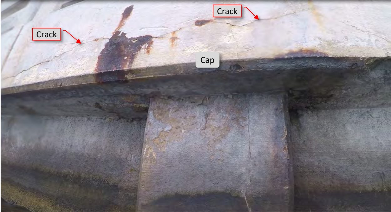
Figure 139: C14. STA 6+22 - 6+40. Crack at cap's vertical face.
