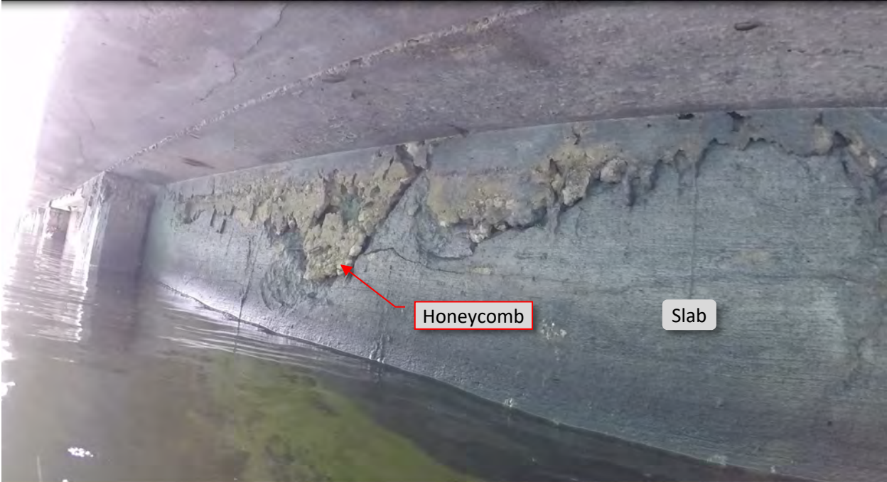
Figure 22: S5. STA 2+93 - 2+99. Honeycomb at top of slab. West direction view.
