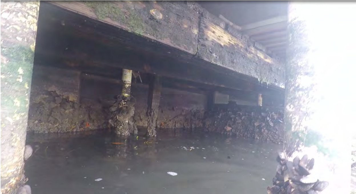
Figure 4: STA 0+10. Northeast direction view. Partial view of seawall, debris, and obstructions.
