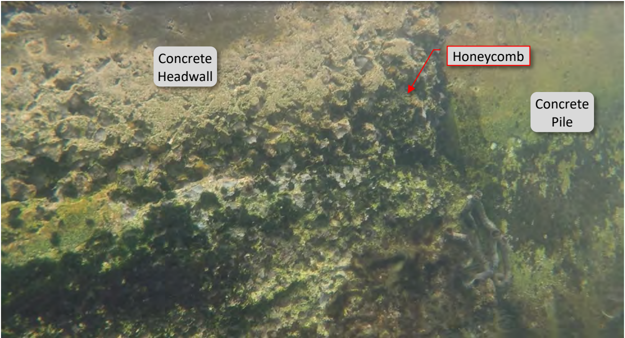
Figure 12: HW1. STA 2+49 - 2+50. Honeycomb area at culvert headwall.
