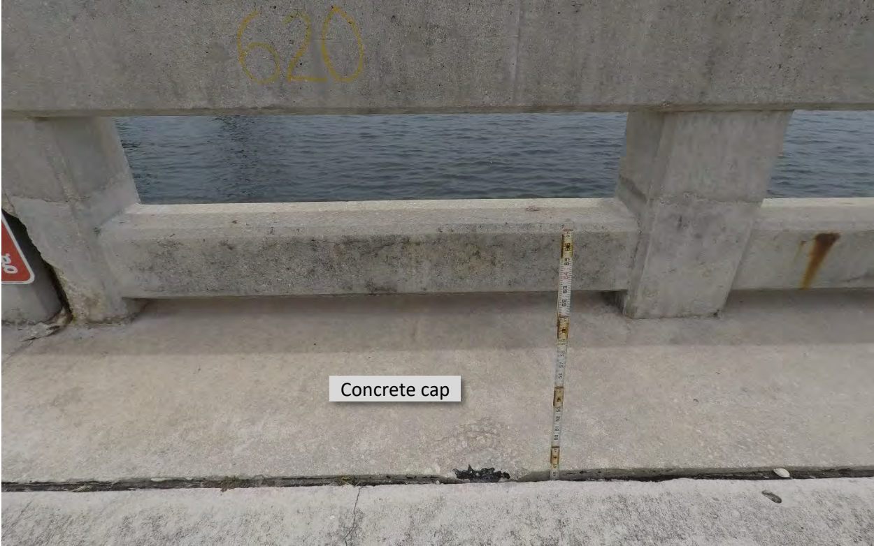
Figure 6: STA 6+20. 48-Inch void at gap between seawall cap and concrete slab at sidewalk.
