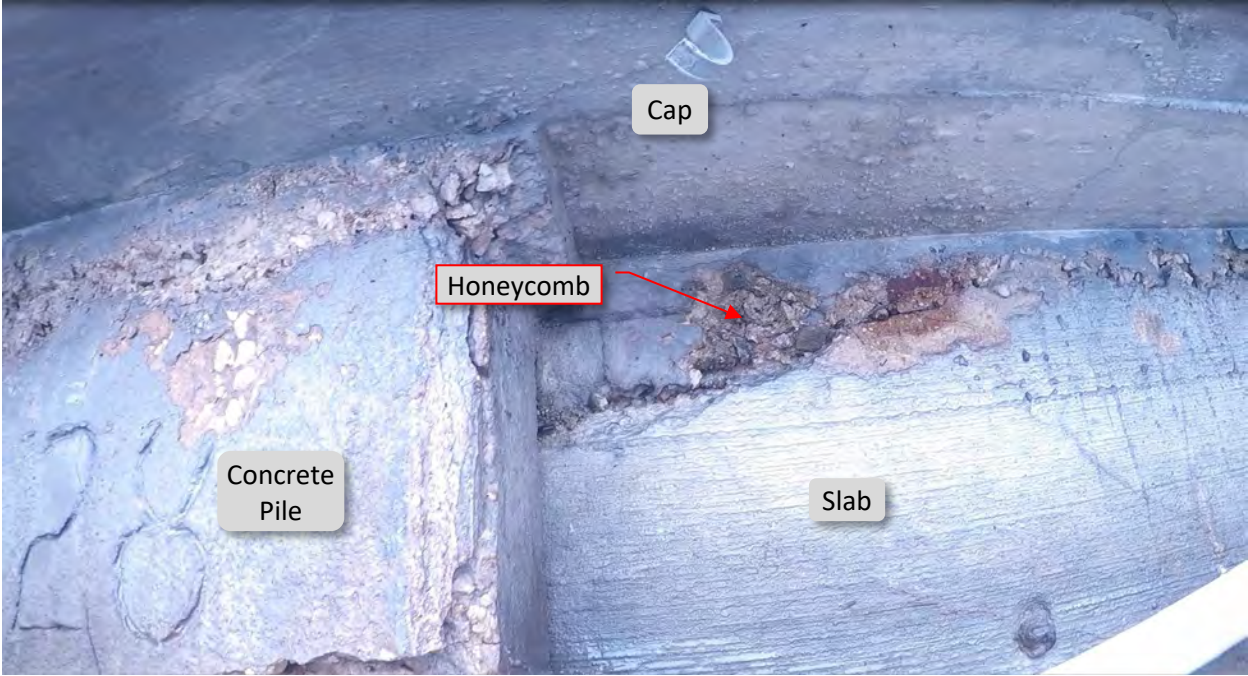
Figure 67: S16. STA 4+37 - 4+38. Honeycomb area at west top corner of slab.
