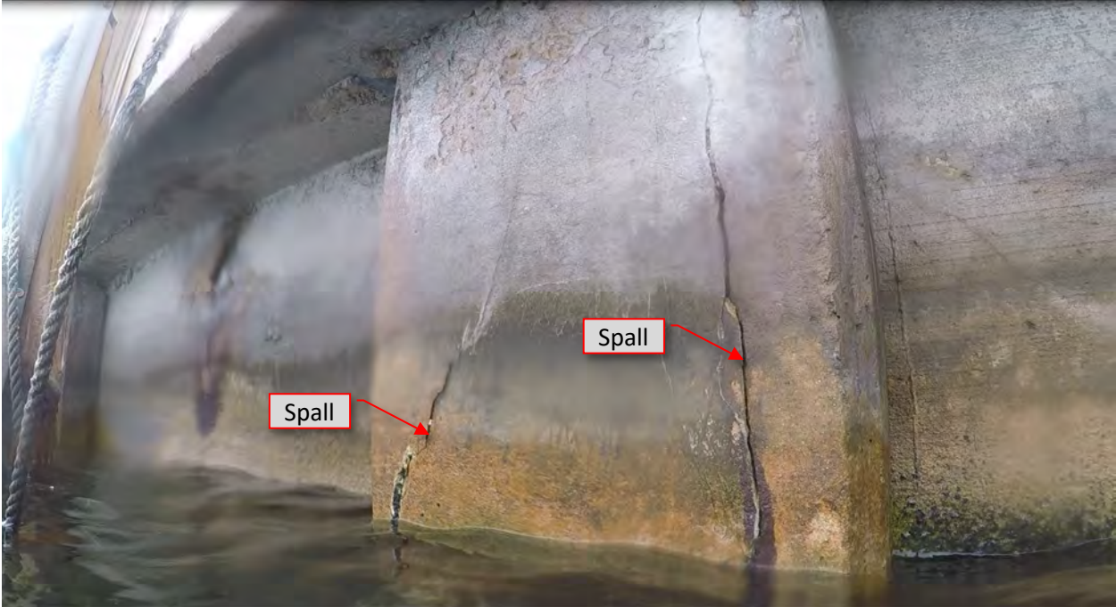
Figure 123: P42. STA 5+93. Crack/spalls at both flanges at pile.
