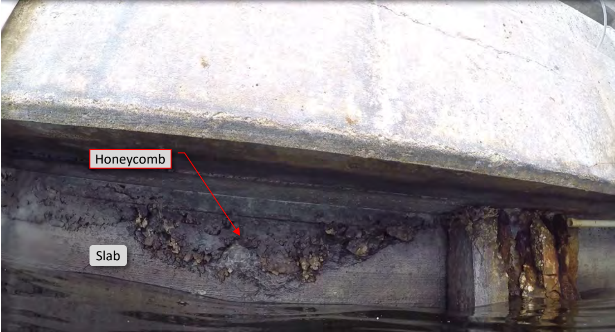
Figure 57: S14. STA 4+08 - 4+11. Honeycomb at top of slab.
