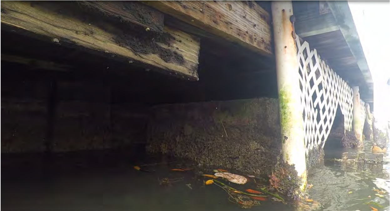
Figure 10: STA 0+50. Northeast direction view. Obstructions and debris in front of seawall, and partial view of seawall.
