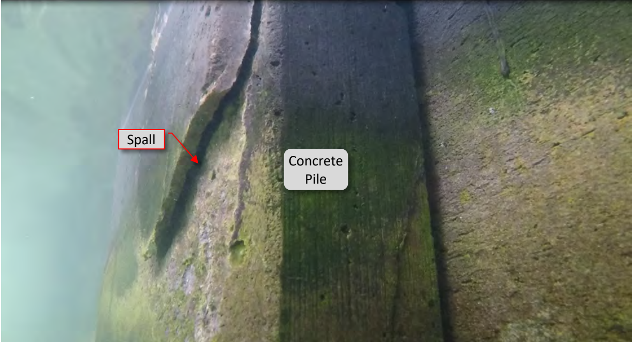
Figure 43: P16. STA 3+56. Spall/crack on south side and near east flange at pile.
