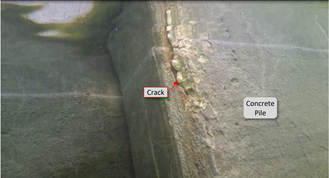
Figure 46: P17. STA 3+63. Crack at west top of flange at pile. Underwater view.
