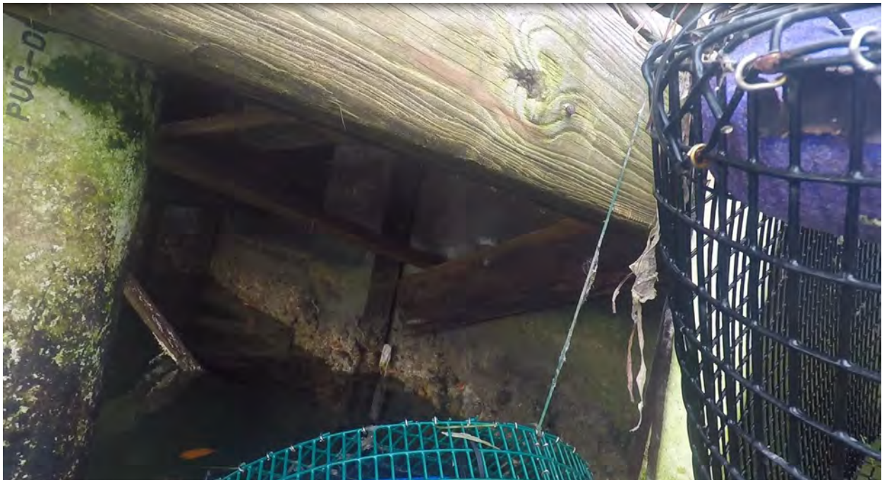
Figure 16: STA 1+20. Northwest direction view. Seawall partial view with present overhead and in the water hazard.
