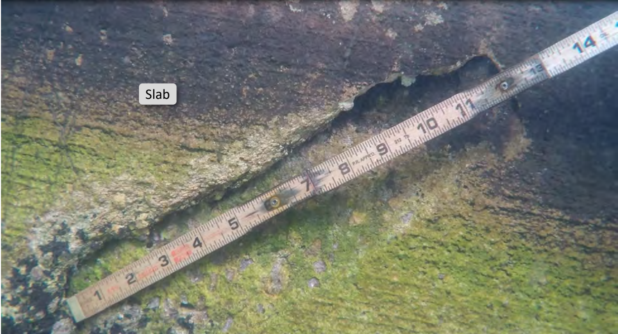
Figure 35: S8. 3+33 - 3+41. Crack at slab midspan. Underwater view.
