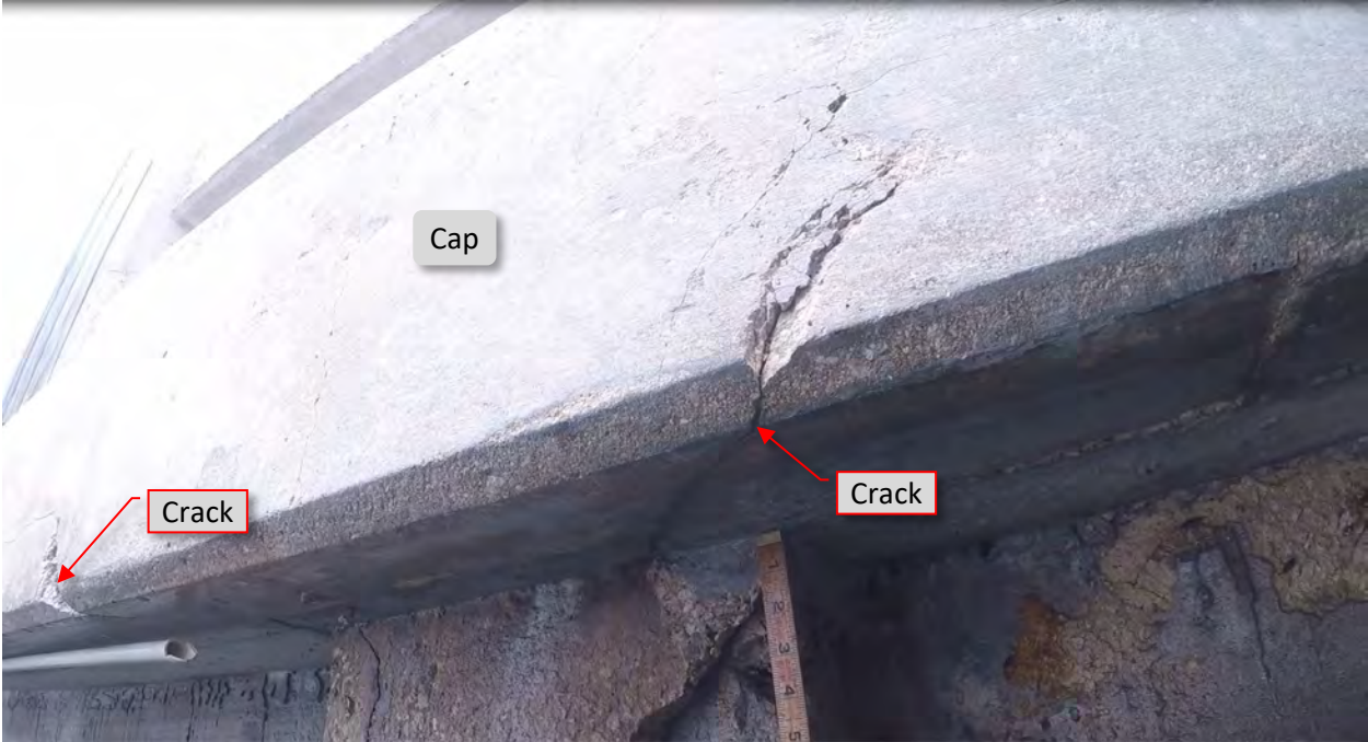
Figure 81: C1. STA 4+84 - 4+93. Two cracks spalled west and east direction on cap from pile's top.
