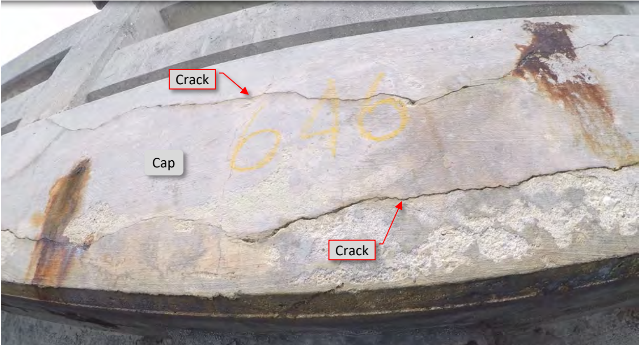
Figure 144. C15. STA 6+40 - 6+50. Crack at cap's vertical face.
