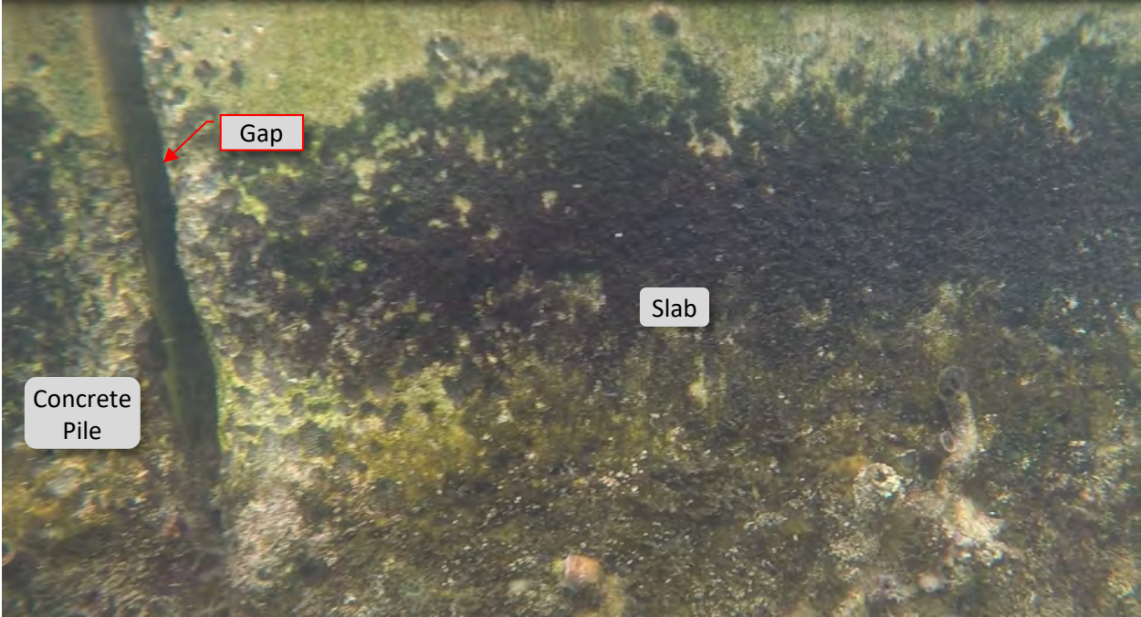
Figure 119: P40. STA 5+80. Gap at construction/expansion joint. Underwater view.
