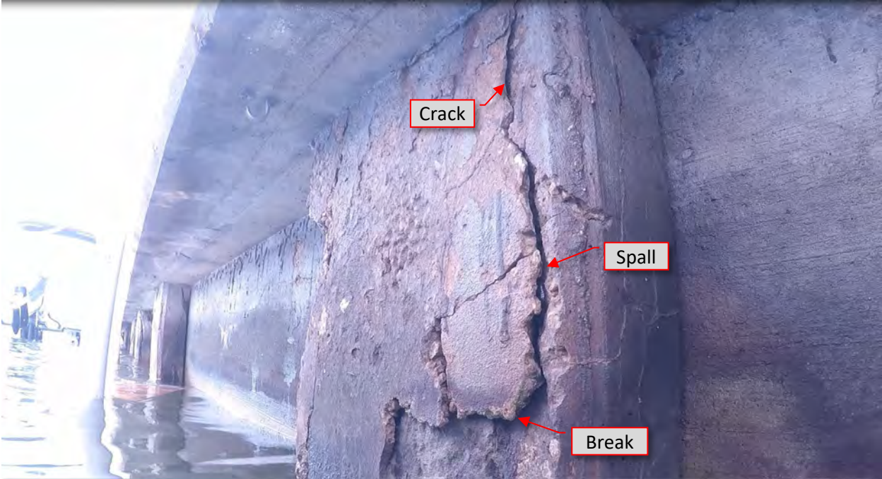
Figure 101: P35. STA 5+40. Cracks/spalls at both flanges and loss of concrete. View of east flange.
