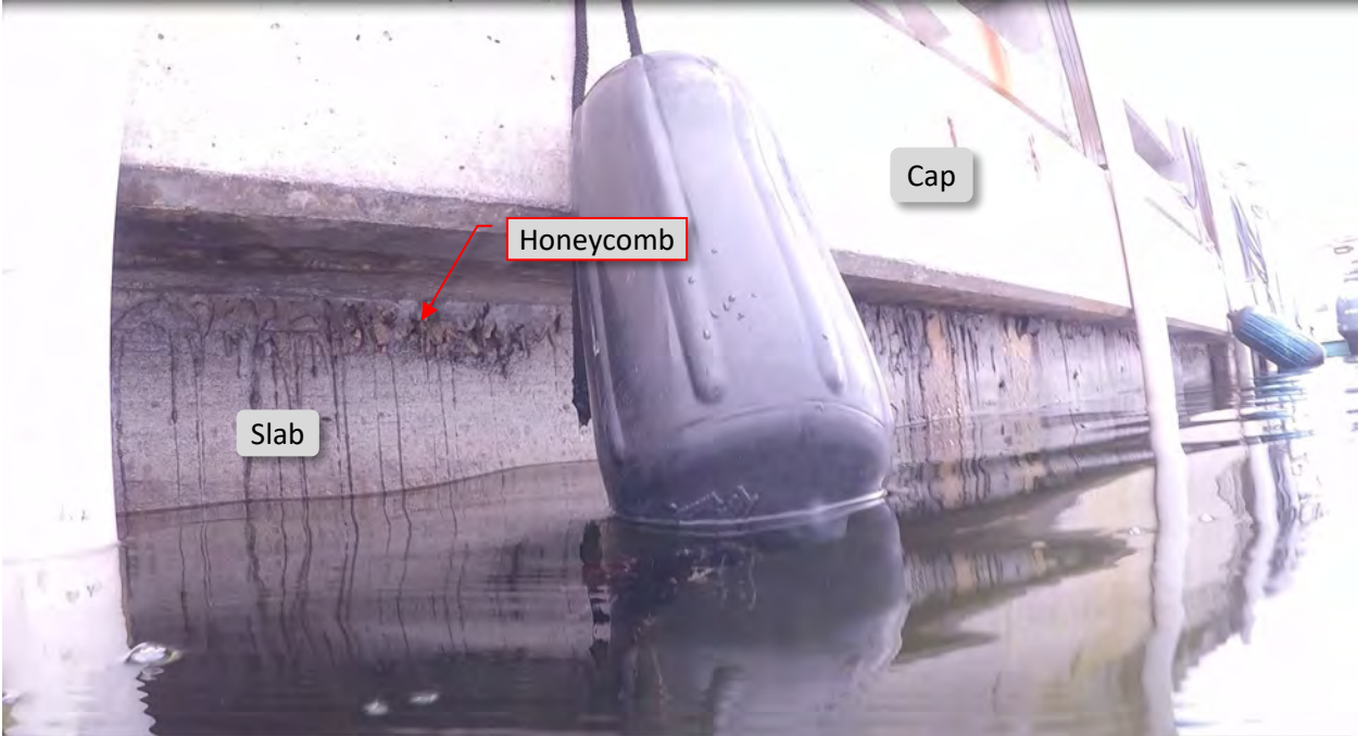
Figure 11: S3. STA 2+38 - 2+41. Concrete erosion at honeycomb area on slab.
