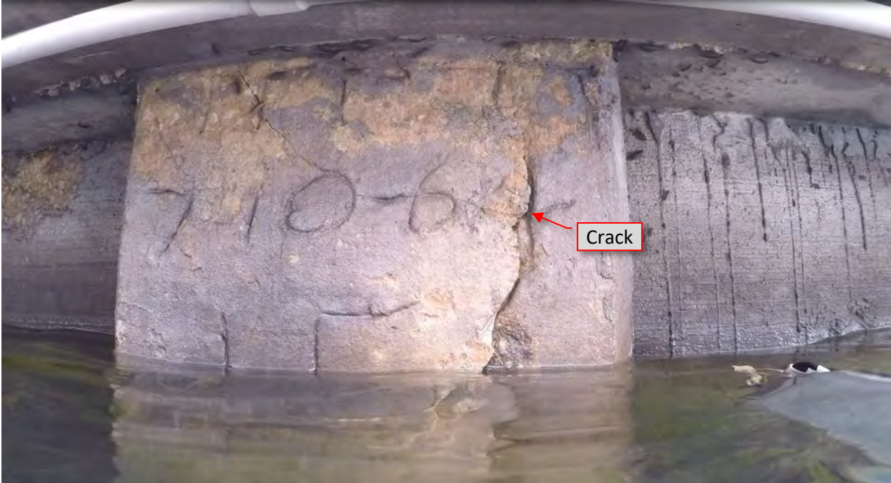
Figure 6: P3. STA 1+72. Crack/spall at pile.
