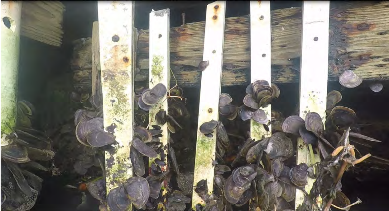
Figure 2: STA 0+00. North direction view. Obstructions and debris in front of seawall.
