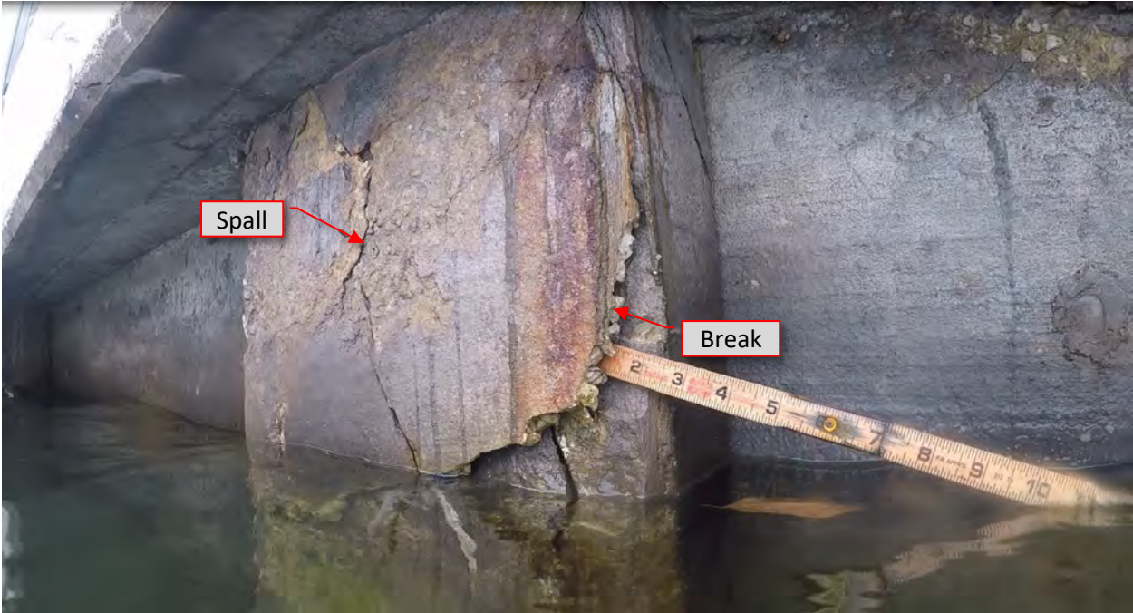
Figure 94: P32. STA 5+16. Cracks/spalls at both flanges and south face, loss of concrete, and rust staining.
