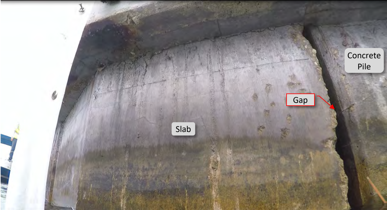
Figure 120: P40. STA 5+85. Gap at construction/expansion joint.
