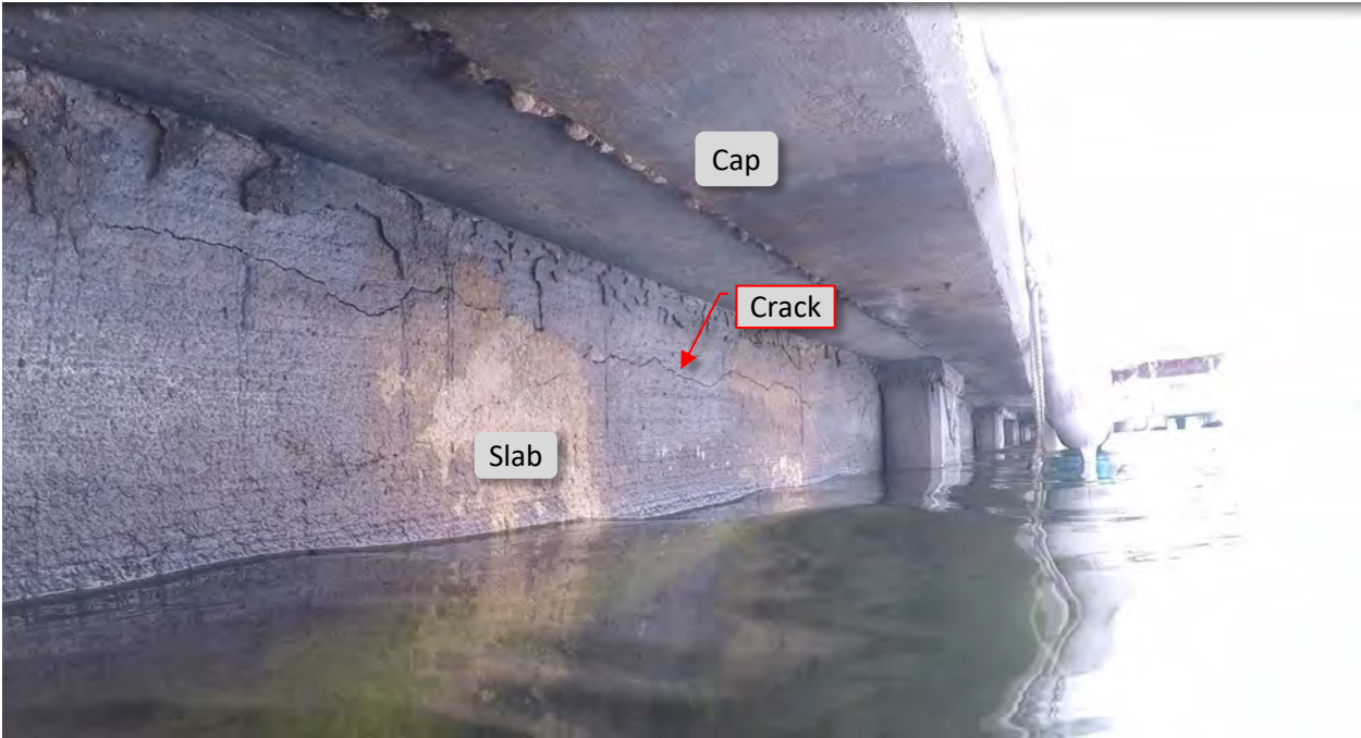
Figure 34: S8. 3+33 - 3+41. Crack/spall at top of slab.
