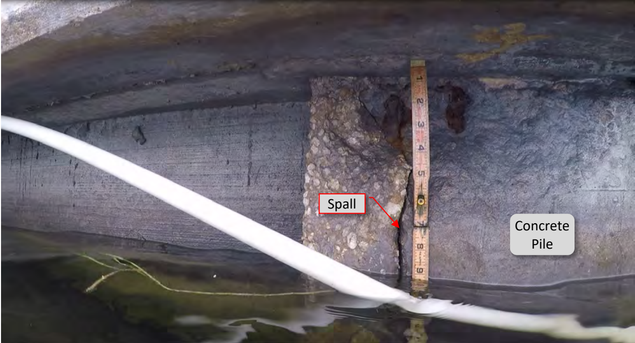
Figure 55: P20. STA 4+04. Spall/crack at west flange at pile.
