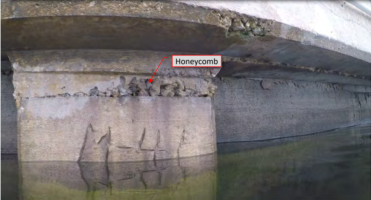
Figure 14: P5. STA 2+60. Honeycomb at pile top.
