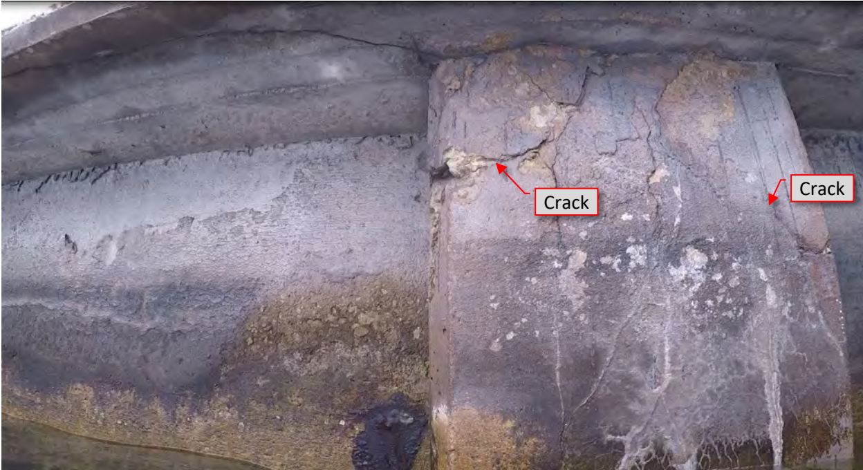
Figure 98: P34. STA 5+30. Cracks/spalls at top of pile west and east flanges, loss of concrete, and rust staining.
