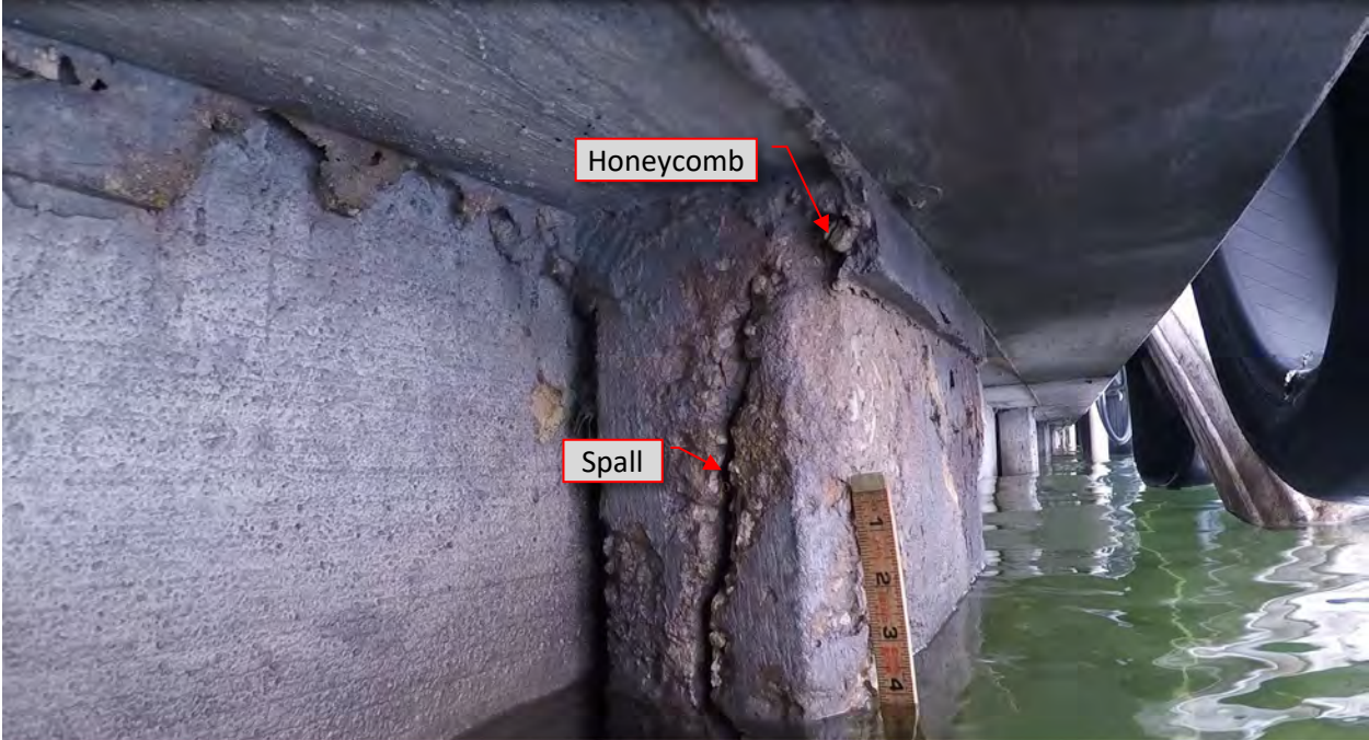
Figure 47: P18. STA 3+71. Spall/crack at west top of flange at pile. Honeycomb area.
