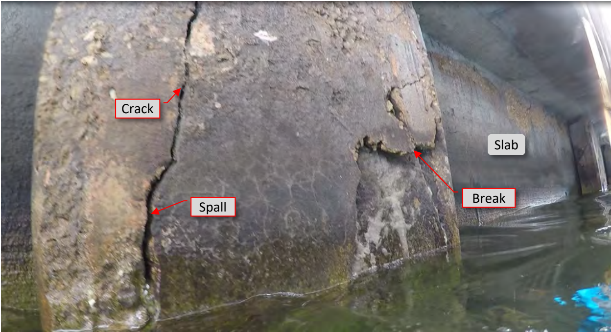
Figure 102: P35. STA 5+40. Cracks/spalls at both flanges at pile and loss of concrete. View of west flange.
