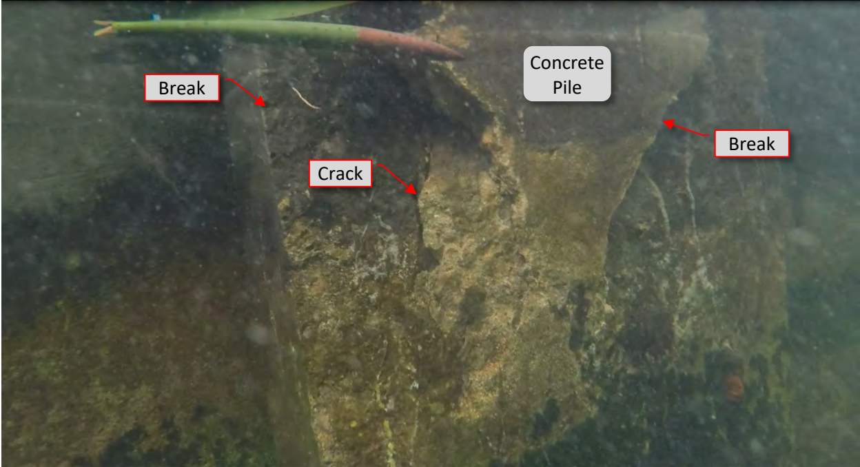
Figure 89: P30. STA 5+00. Cracks/spalls at both flanges and loss of concrete. Underwater view.
