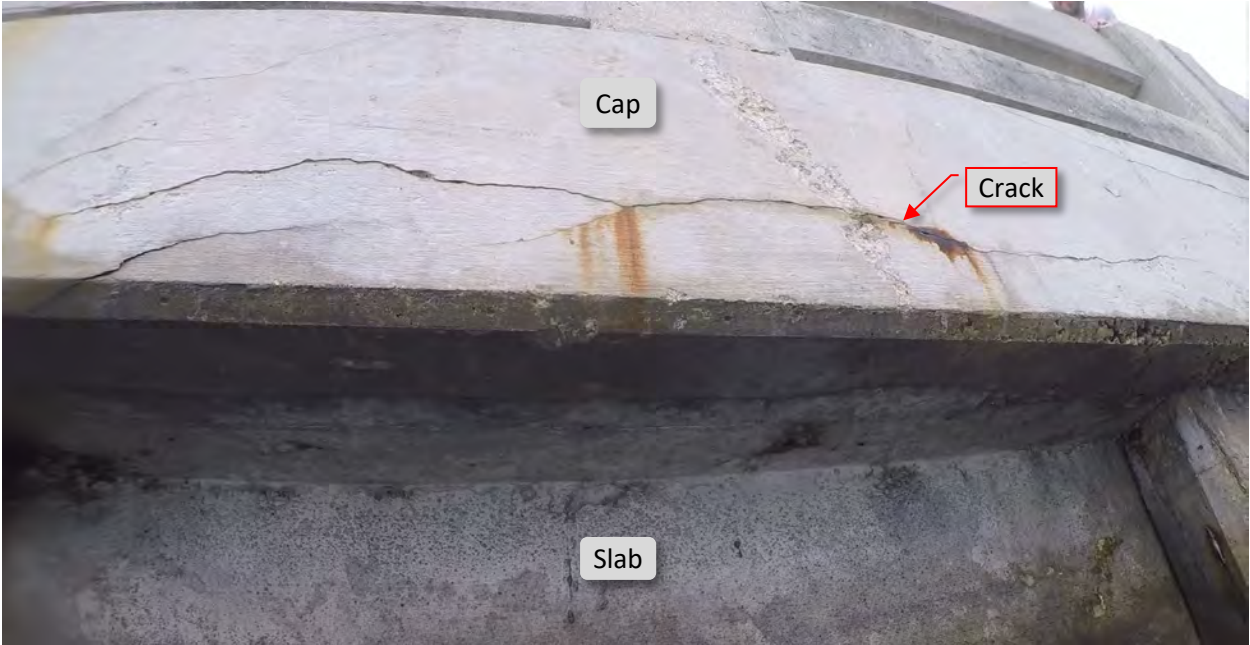
Figure 86: C2. STA 4+92 - 4+95. Crack at cap vertical face.
