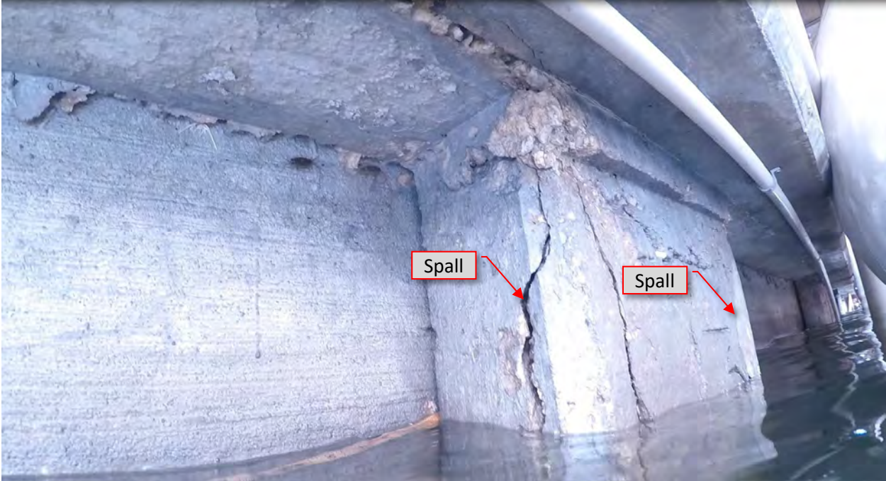
Figure 59: P22. STA 4+20. Break/spall at west and east flanges at pile.
