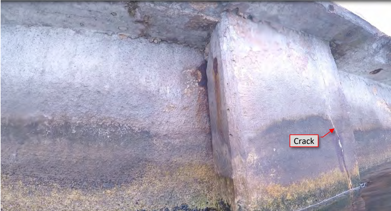
Figure 138: P47. STA 6+27. Crack at north flange at pile.
