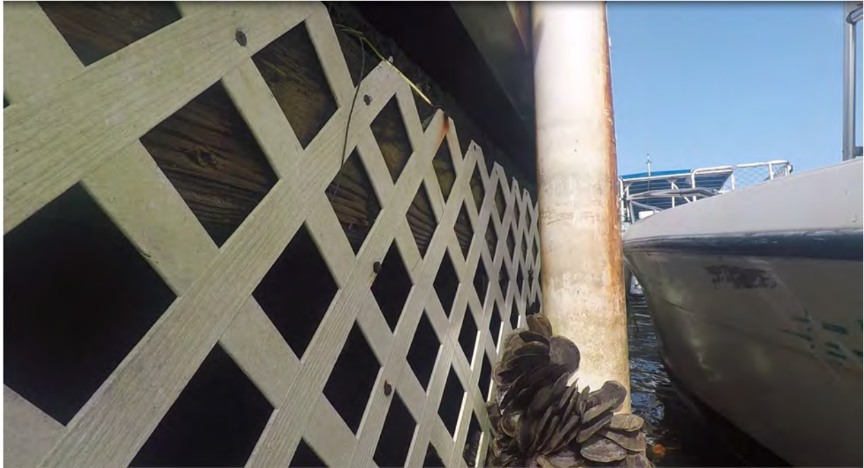
Figure 15: STA 1+00. Northeast direction view. Obstructions and debris in front of seawall.
