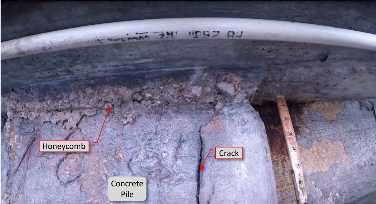
Figure 52: P19. STA 3+96. Crack at east flange at pile. Honeycomb area.
