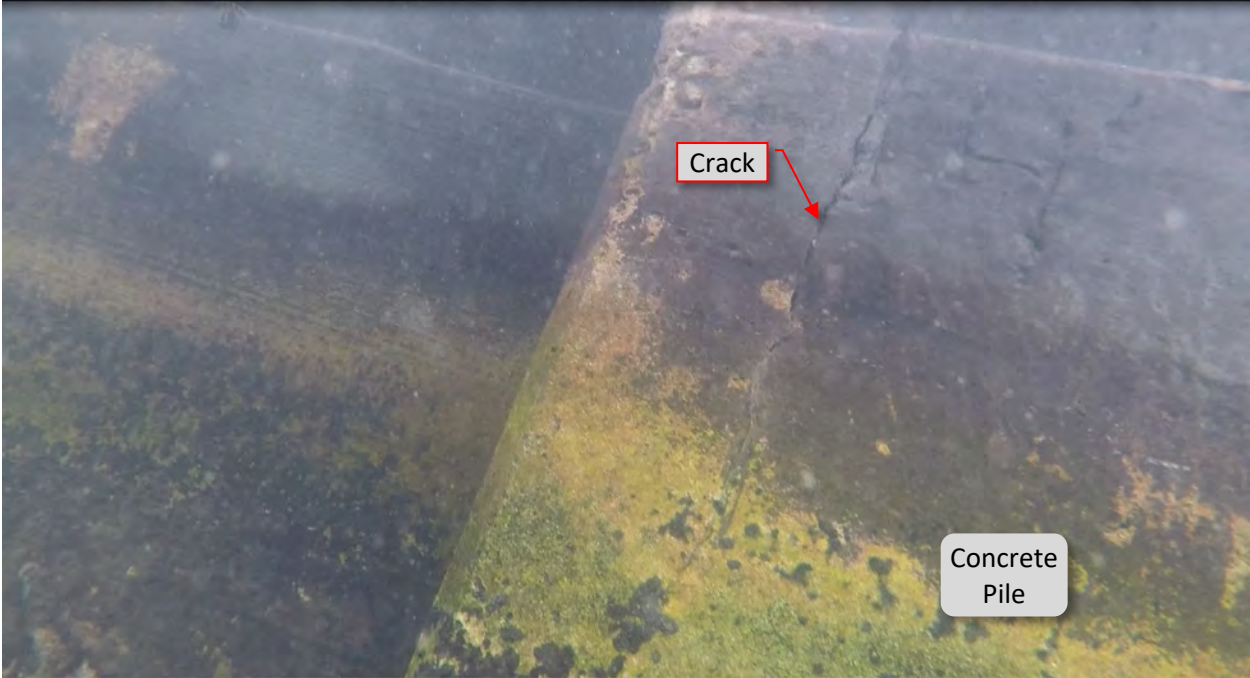
Figure 33: P13. STA 3+31. Crack at west flange at pile. Underwater view.
