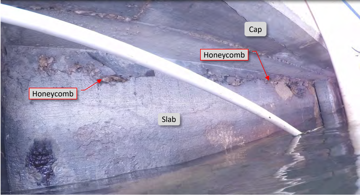
Figure 70: S17. STA 4+45 – 4+52. Honeycomb area along the top of slab.
