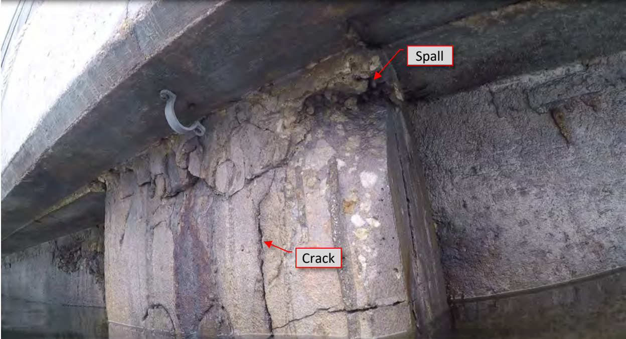
Figure 9: P4. STA 2+35. Multiple cracks and spalls at pile.
