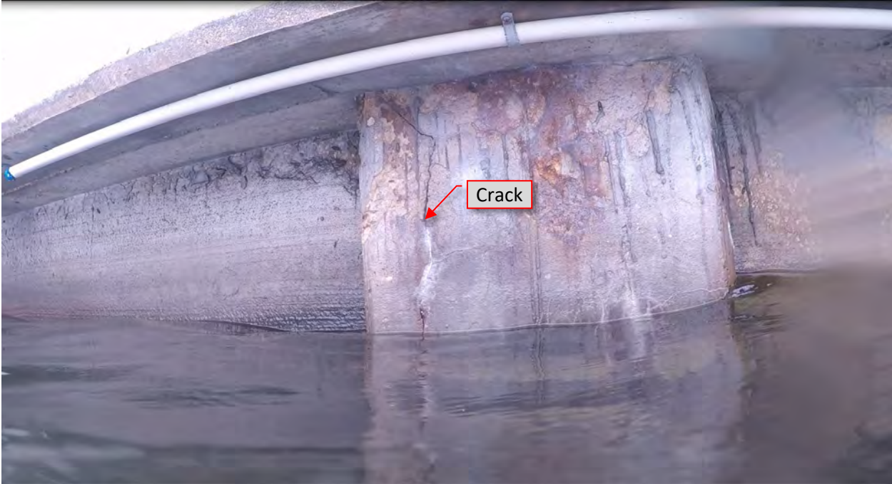
Figure 77: P28. STA 4+67. Crack at top of west flange with rust staining.
