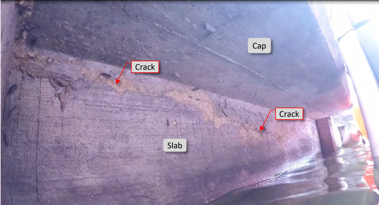
Figure 76: S19. STA 4+61 - 4+67. Crack at top of slab.
