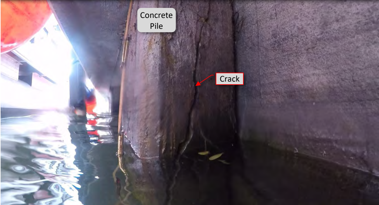
Figure 75: P27. STA 4+60. Crack/spall at top of east flange. View of east face at pile.
