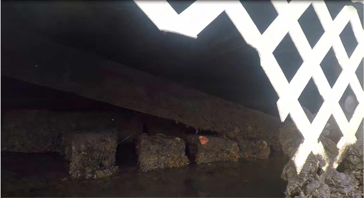
Figure 11: STA 0+60. Northeast direction view. Obstructions and debris in front of seawall, and partial view of seawall.
