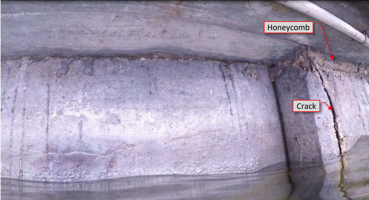
Figure 53: P19. STA 3+96. Crack at west flange at pile. Honeycomb area.
