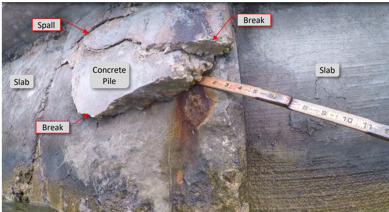
Figure 114: P39. STA 5+72. Cracks/spalls at both flanges at pile with rust staining at east flange, and loss of concrete.
