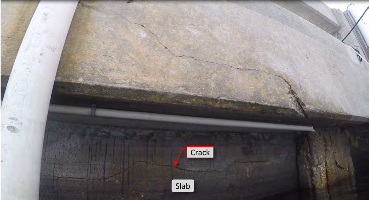
Figure 80: S20. STA 4+84 - 4+90. Crack at top of slab. View of mid to east span of slab.
