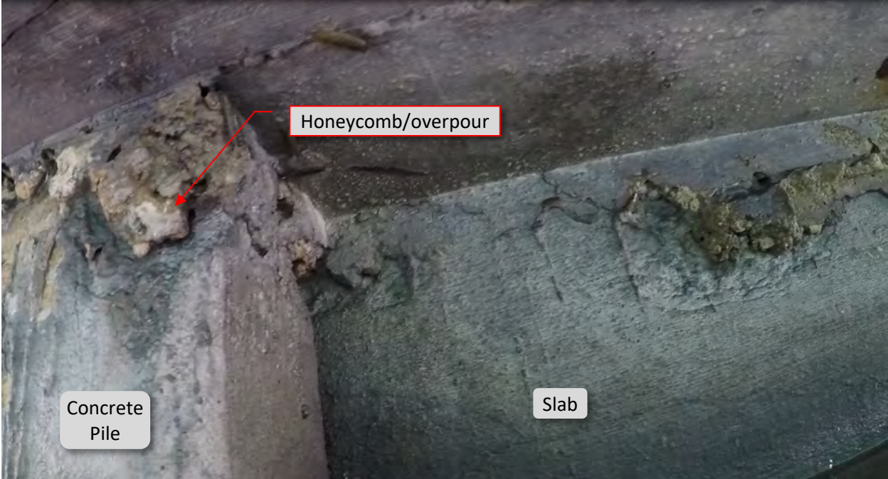
Figure 21: P8. STA 2+94. Honeycomb area and concrete overpour at east flange at pile.
