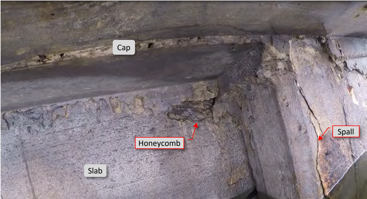
Figure 38: S10. 3+47. Honeycomb area at top east corner of slab. P15. STA 3+48. Crack/spall at west flange at pile.
