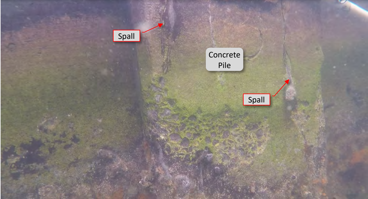
Figure 63: P23. STA 4+28. Spalls at both flanges at pile.
