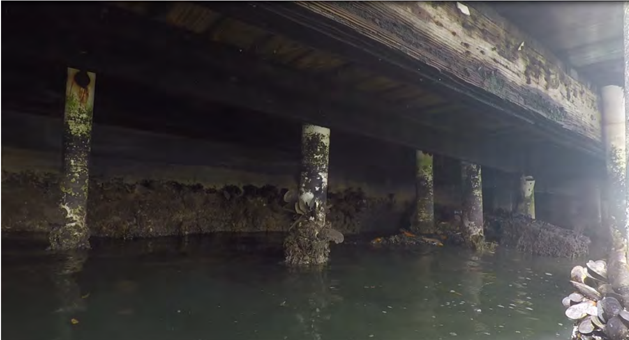
Figure 6: STA 0+20. Northeast direction view. Obstructions and debris in front of seawall, and partial view of seawall.
