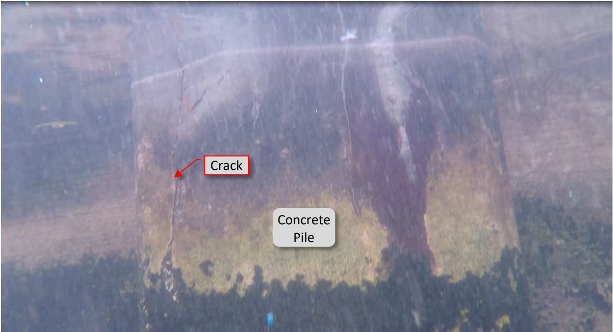
Figure 78: P28. STA 4+67. Crack at top of west flange with rust staining. Underwater view.
