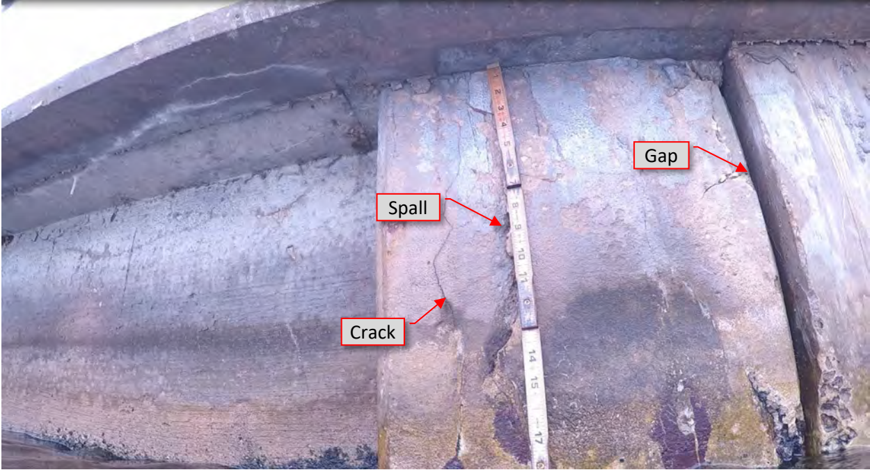
Figure 127: P44. STA 6+07. Cracks/spalls at both flanges at pile. Gap at construction/expansion joint.
