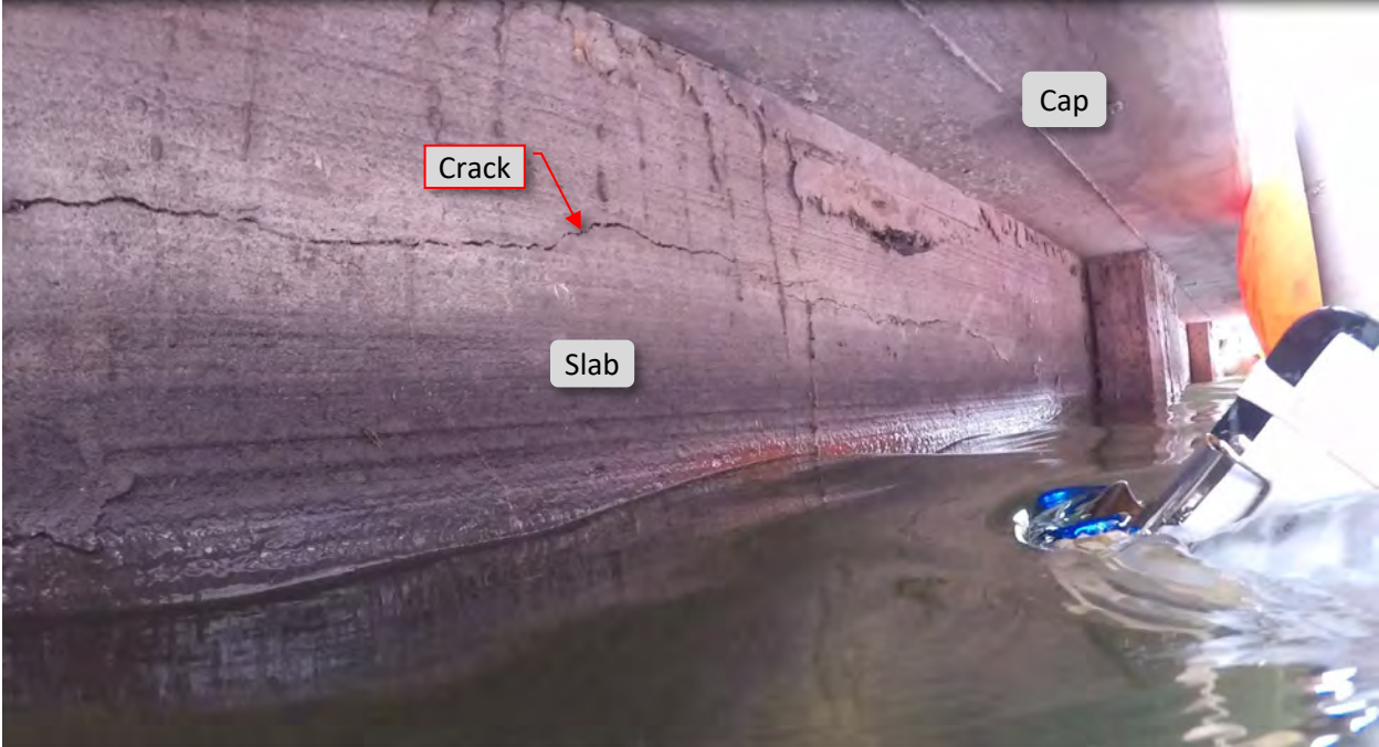
Figure 73: S18. STA 4+54 - 4+59. Crack at top of slab.
