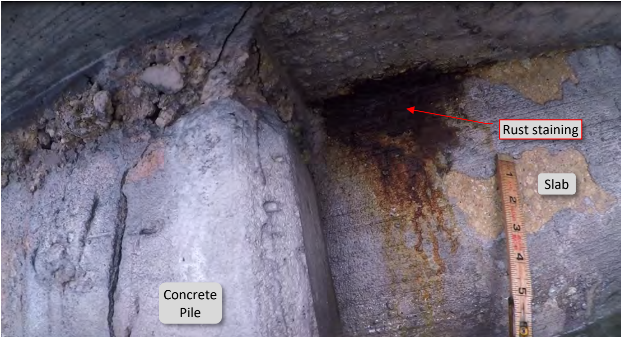
Figure 54: S13. STA 3+97. Rust staining area at top of slab west corner.
