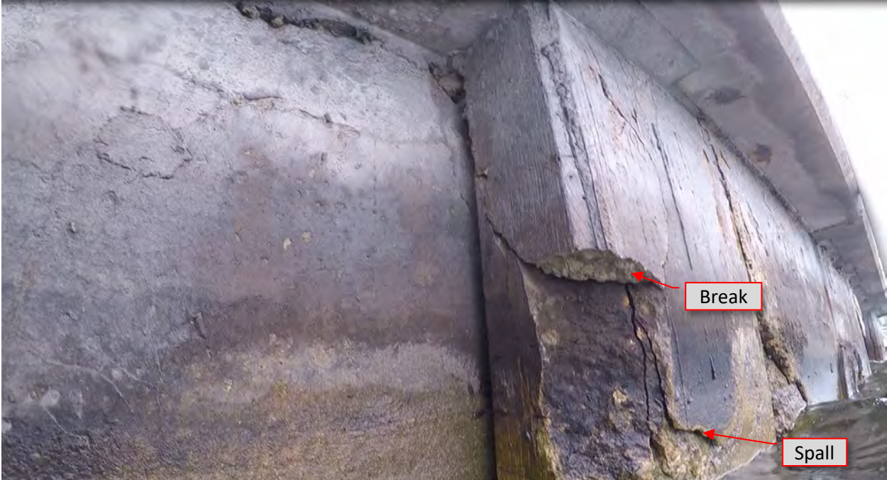
Figure 111: P38. STA 5+64. Cracks/spalls at both flanges at pile and loss of concrete. View of west flange.
