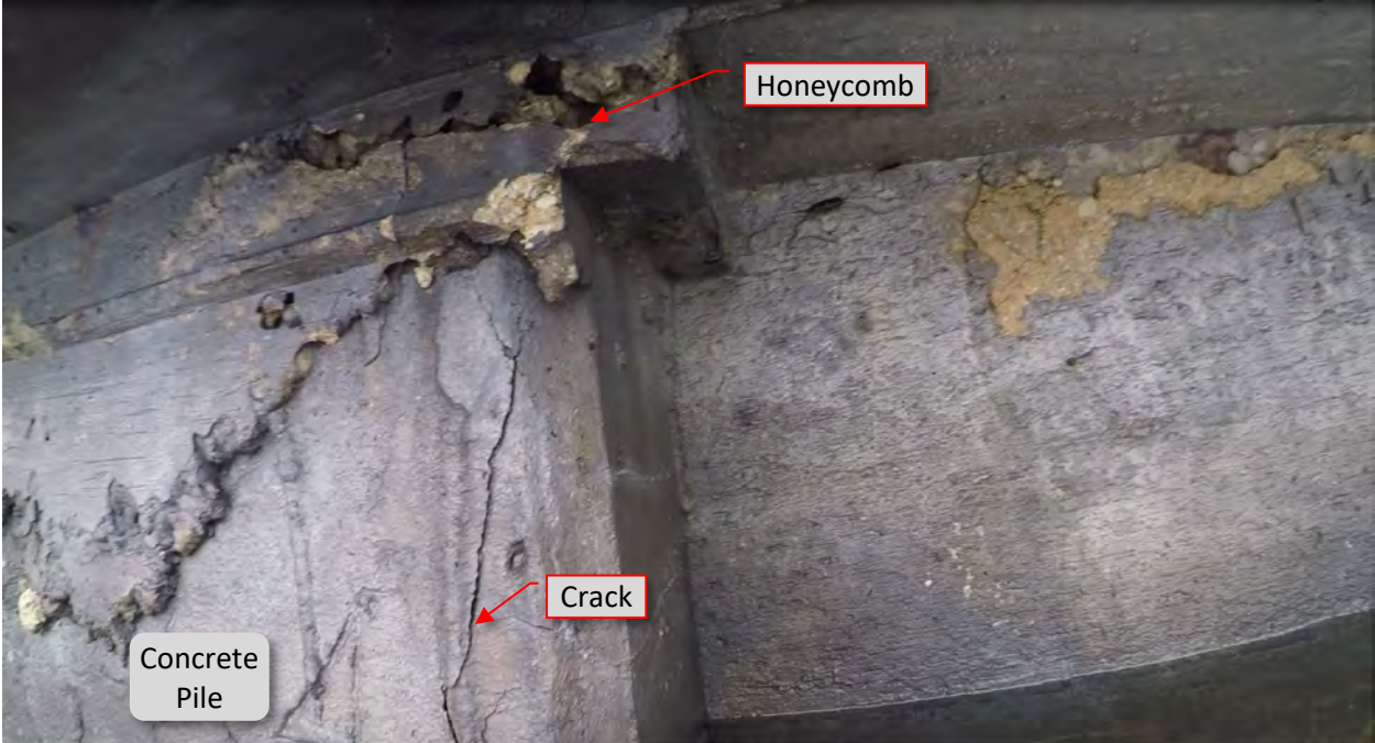
Figure 17: P6. STA 2+76. Honeycomb across the pile top. Crack/spall at east flange on pile.
