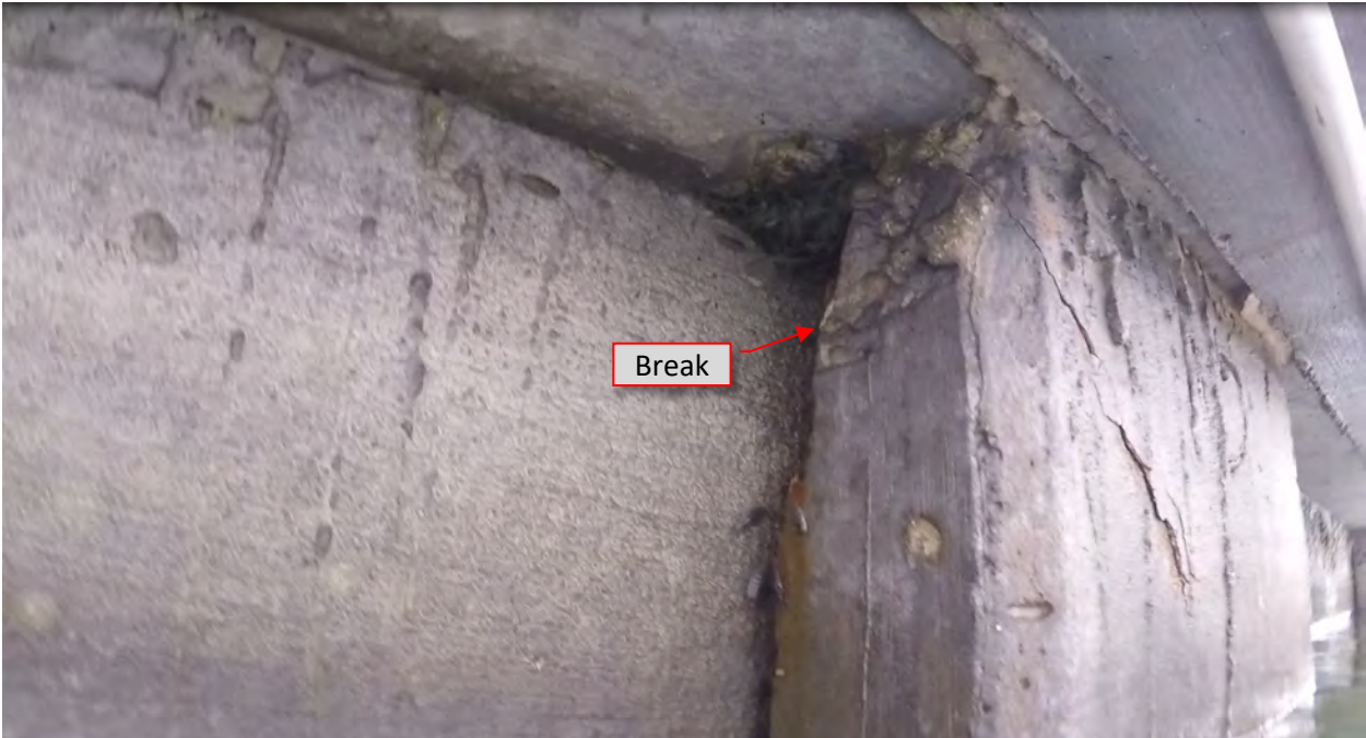
Figure 4: P2. STA 1+64. Break at top west flange and crack on south face on pile.
