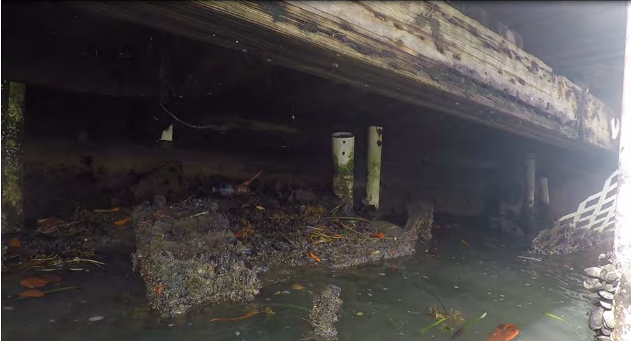
Figure 7: STA 0+30. Northeast direction view. Obstructions and debris in front of seawall, and partial view of seawall.
