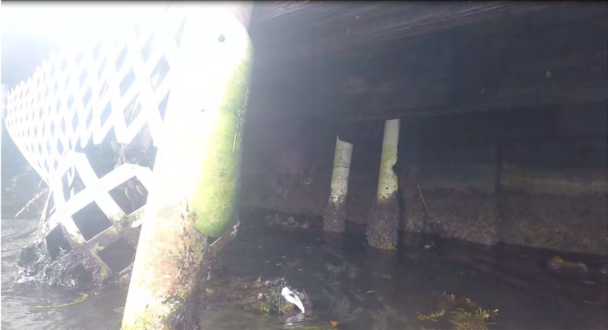
Figure 9: STA 0+40. Northwest direction view. Obstructions and debris in front of seawall, and partial view of seawall.
