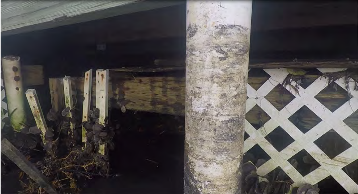
Figure 1: STA 0+00. Northwest direction view. Obstructions and debris in front of seawall.
