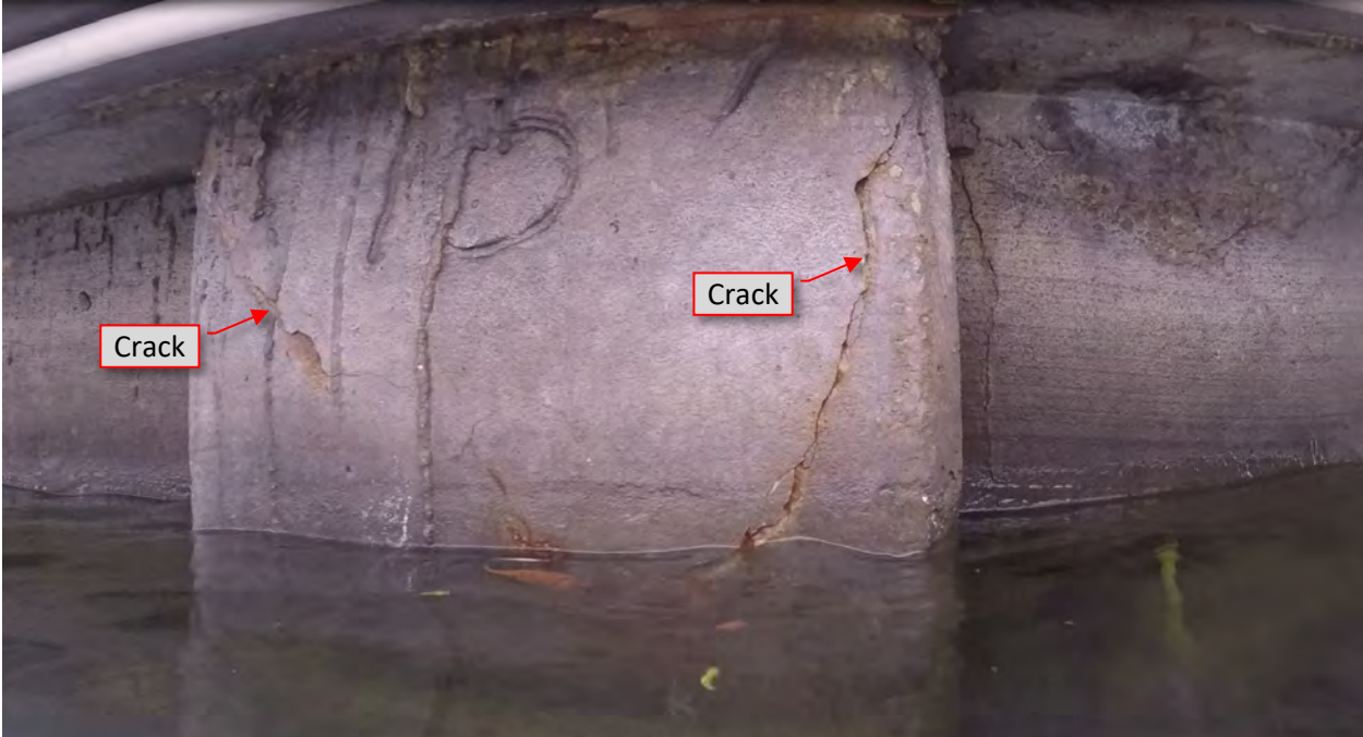
Figure 3: P2. STA 1+64. Crack/spall on pile.
