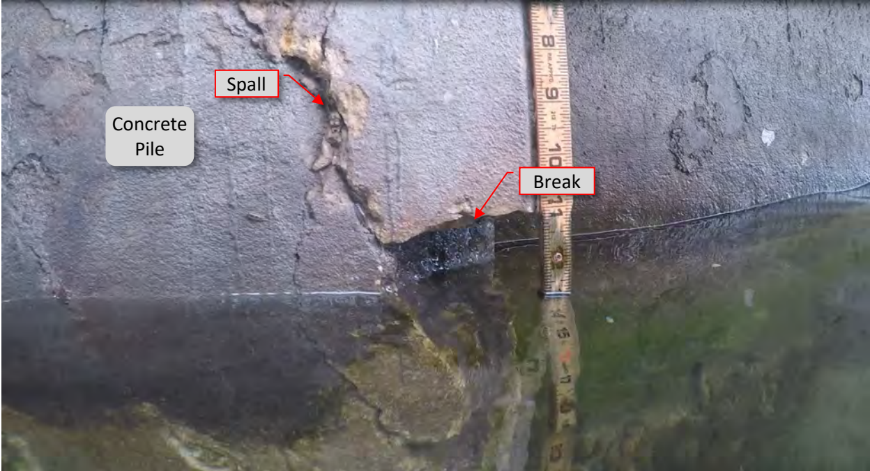
Figure 91: P31. STA 5+08. Cracks/spalls at east flange and loss of concrete.
