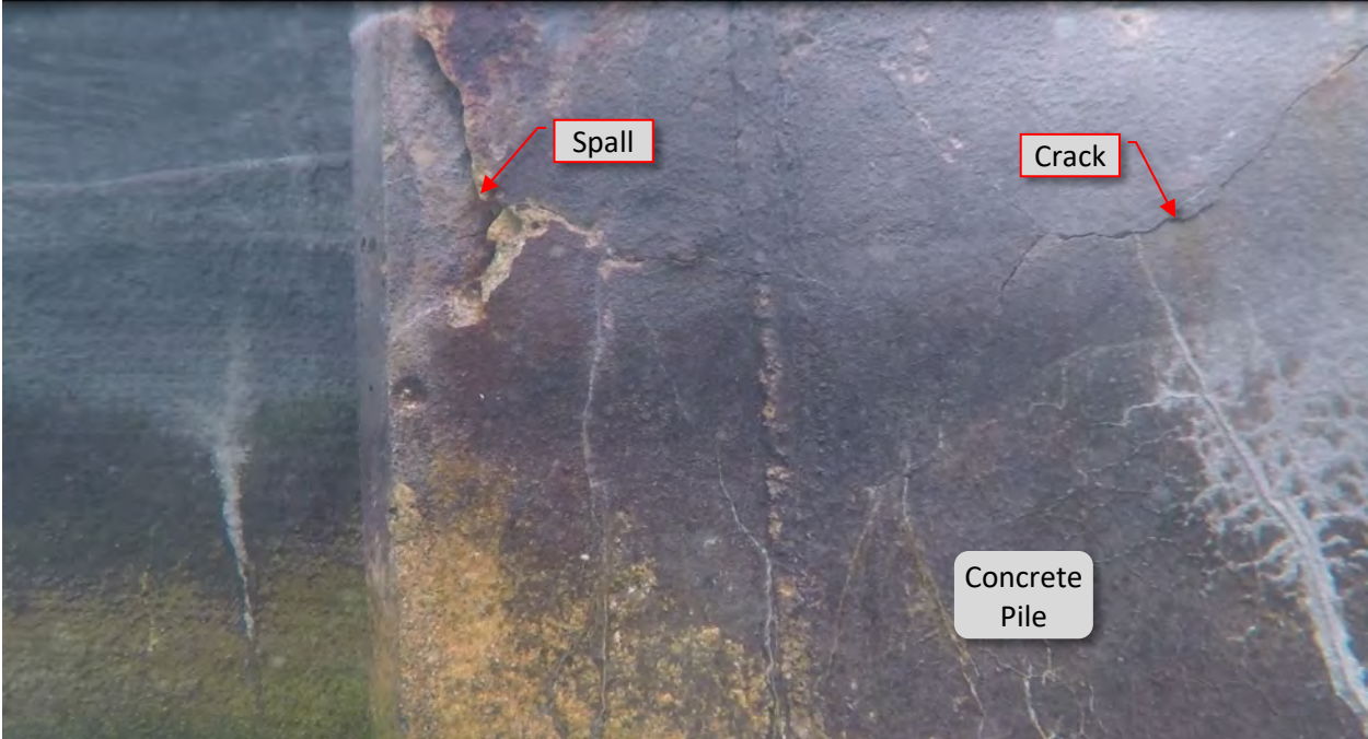
Figure 40: P15. STA 3+48. Cracks at south face and spall at west flange at pile.
