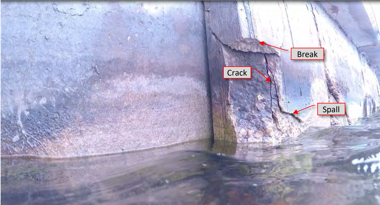
Figure 112: P38. STA 5+64. Cracks/spalls at both flanges at pile and loss of concrete. View of west flange at water level.
