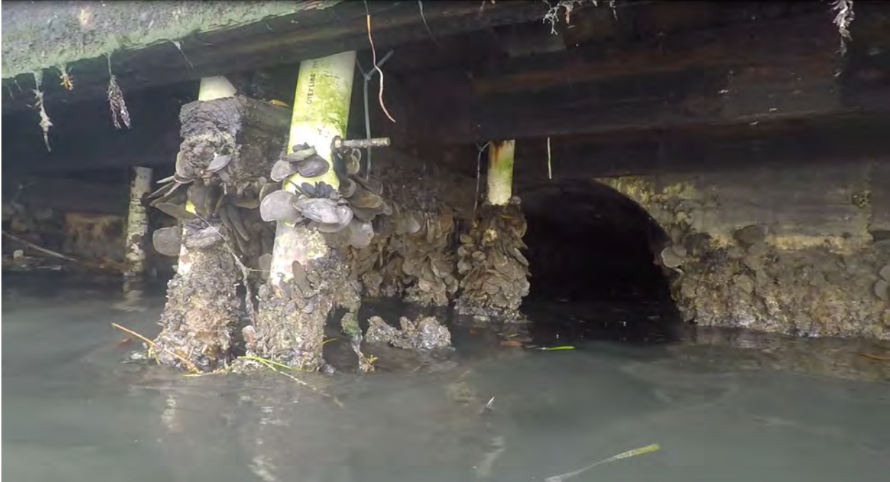
Figure 3: STA 0+10. Northwest direction view. Obstructions and debris in front of seawall and at culvert at STA 0+09.
