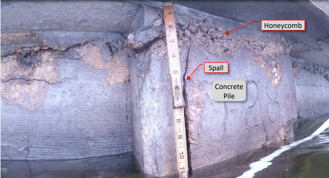
Figure 65: P24. STA 4+36. Break/spall at both flanges at pile. Honeycomb area.
