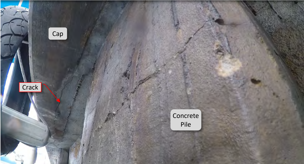
Figure 104: C7. STA 5+40 - 5+48. Crack at cap's bottom face.
