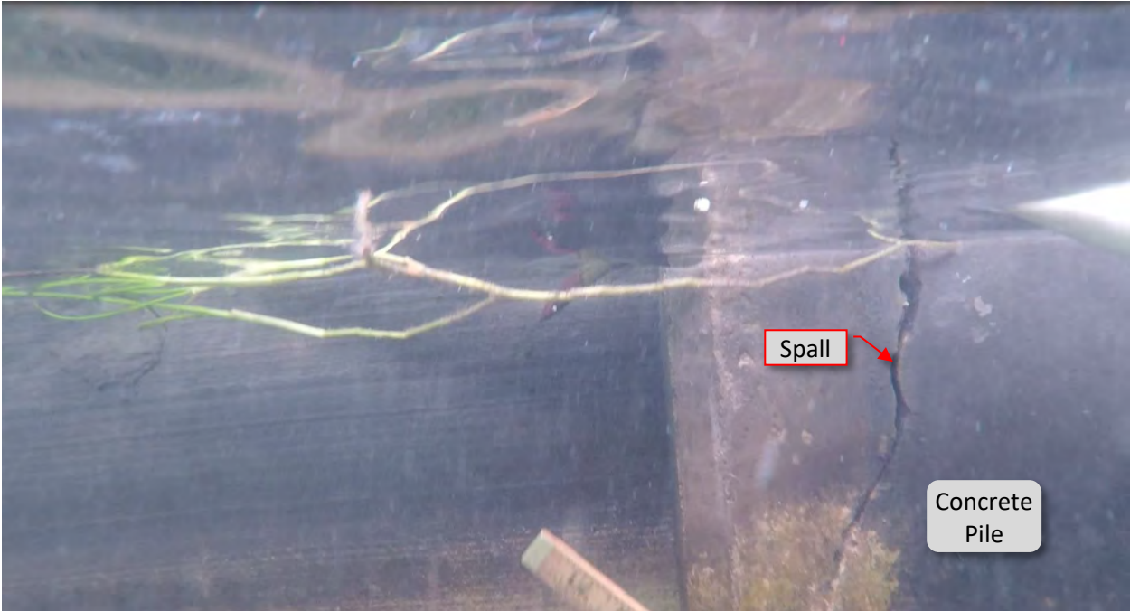
Figure 56: P20. STA 4+04. Spall/crack at west flange at pile. Underwater view.
