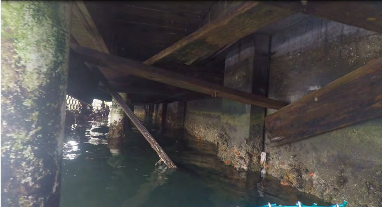
Figure 17: STA 1+20. West direction view. Seawall partial view with present overhead and in the water hazard.
