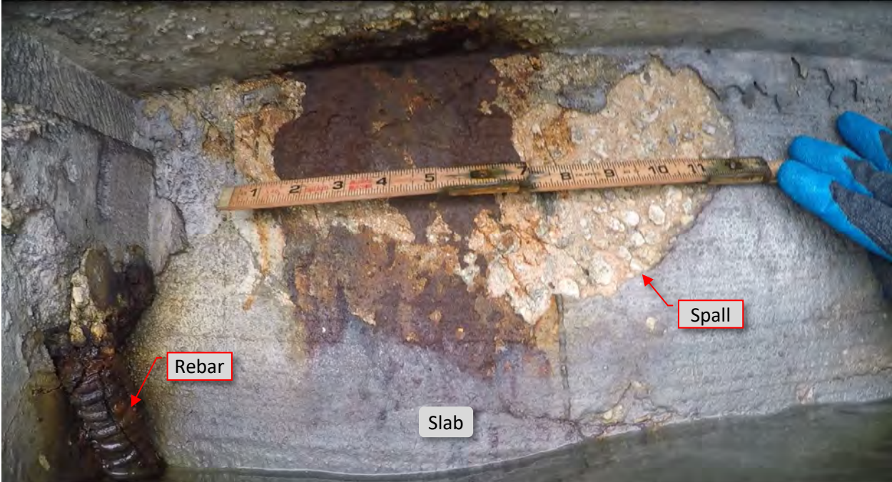
Figure 37: P14. STA 3+39. #11 Size rebar protrusion at east flange. S9. STA 3+41. Spall with rust staining at slab west corner.
