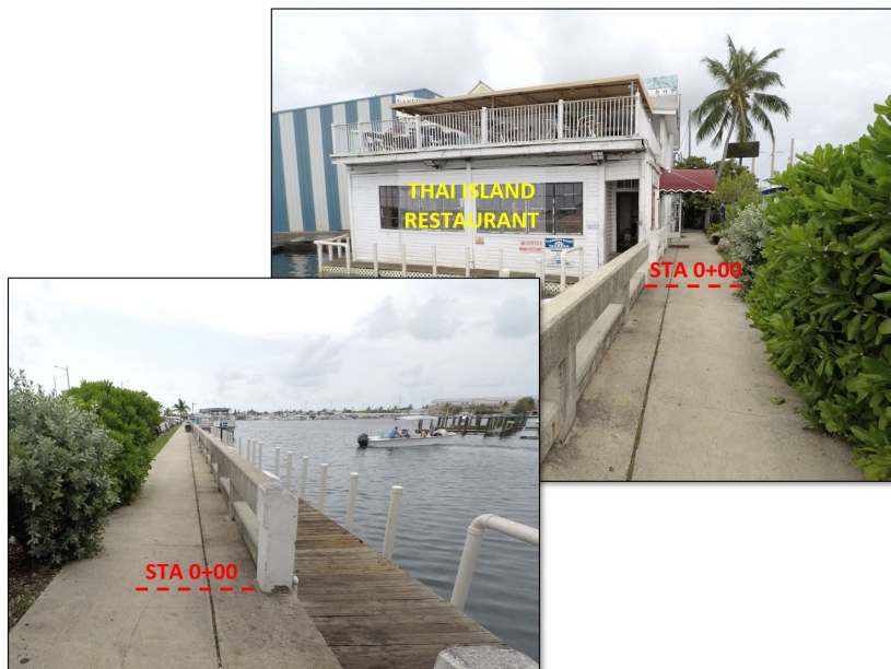
Figure 3: Inspection Starting Point (STA 0+00). West (top right) and east (bottom left) Direction Views.
