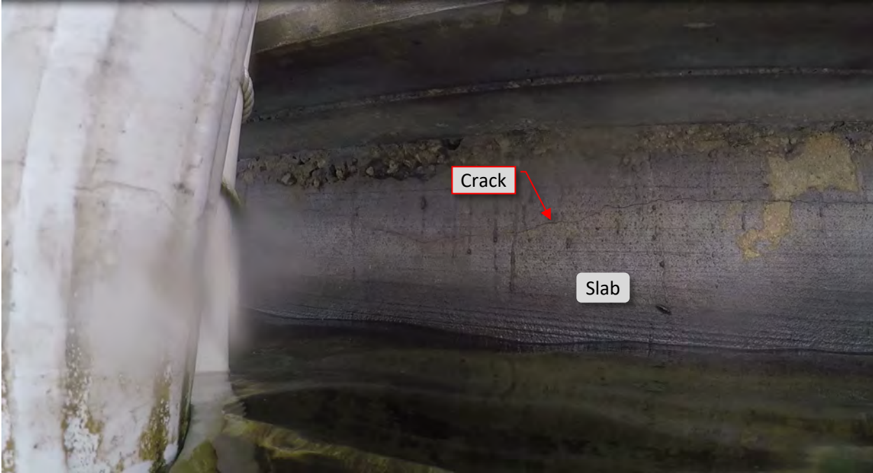
Figure 64: S15. STA 4+30 - 4+35. Crack at top of slab. Honeycomb area.
