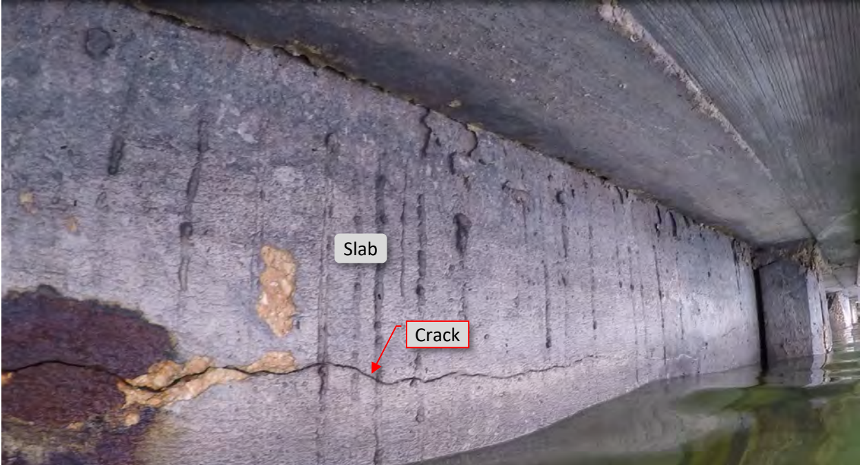
Figure 51: S12. STA 3+87 - 3+95. Crack at top of slab.
