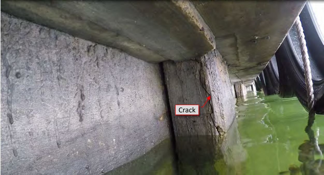
Figure 45: P17. STA 3+63. Crack at west top of flange at pile.
