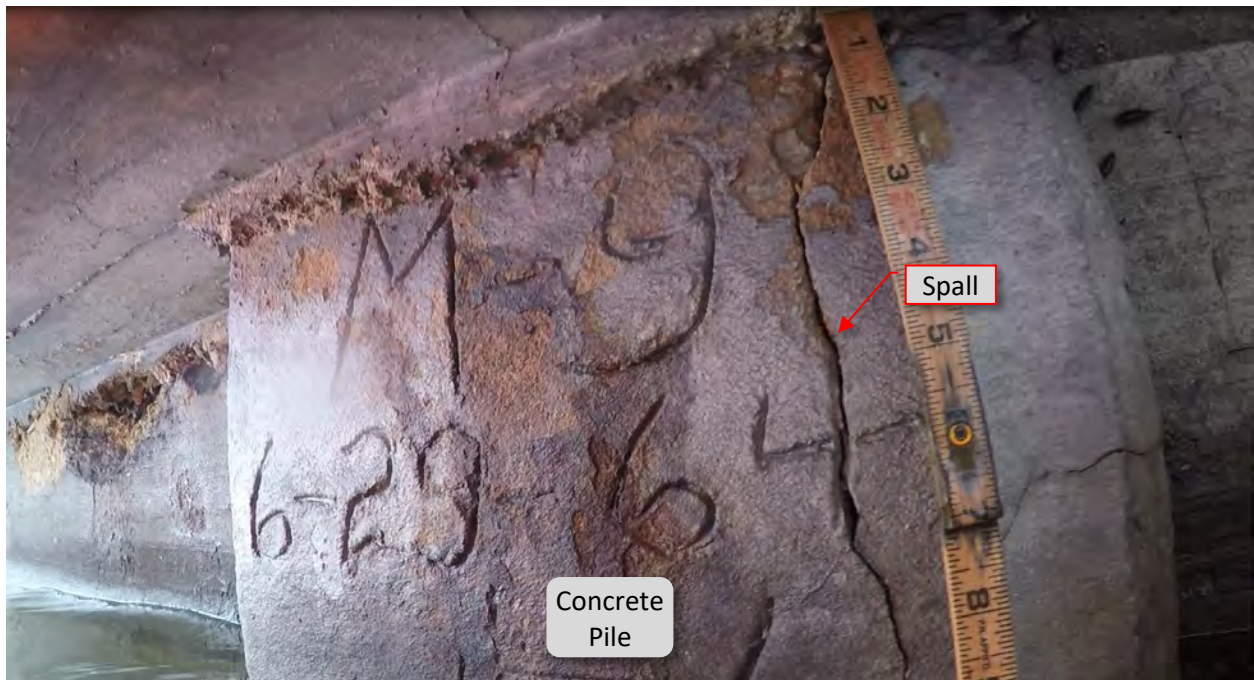
Figure 72: P26. STA 4+53. Breaks/spalls at both flanges at pile. Honeycomb area.
