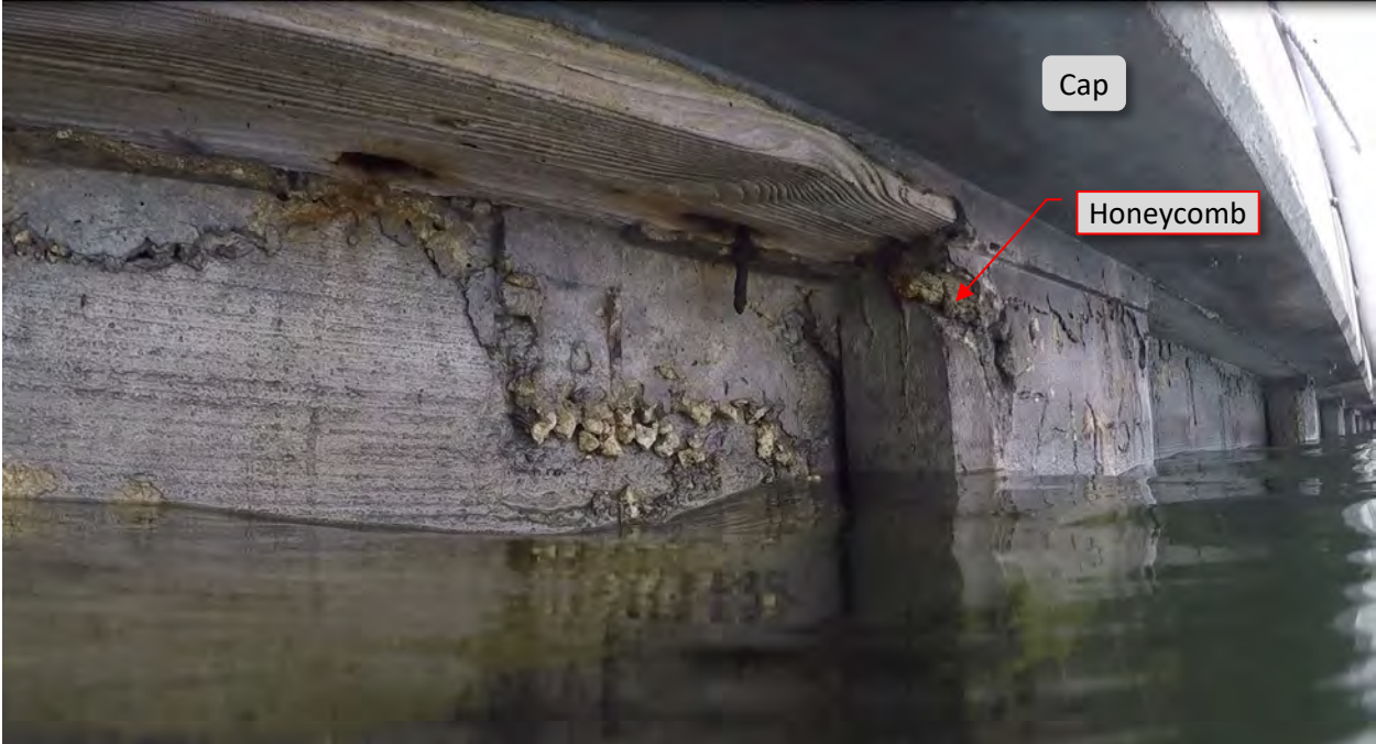
Figure 31: P12. STA 3+24. Honeycomb at pile top.
