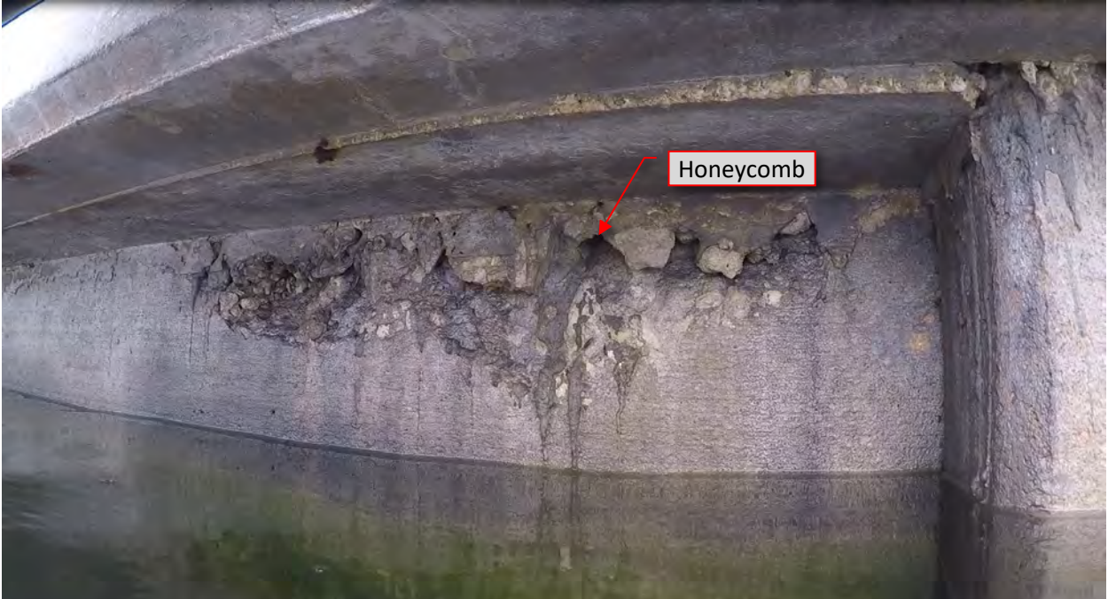
Figure 8: S2. STA 2+31 - 2+34. Concrete erosion at honeycomb area on slab.
