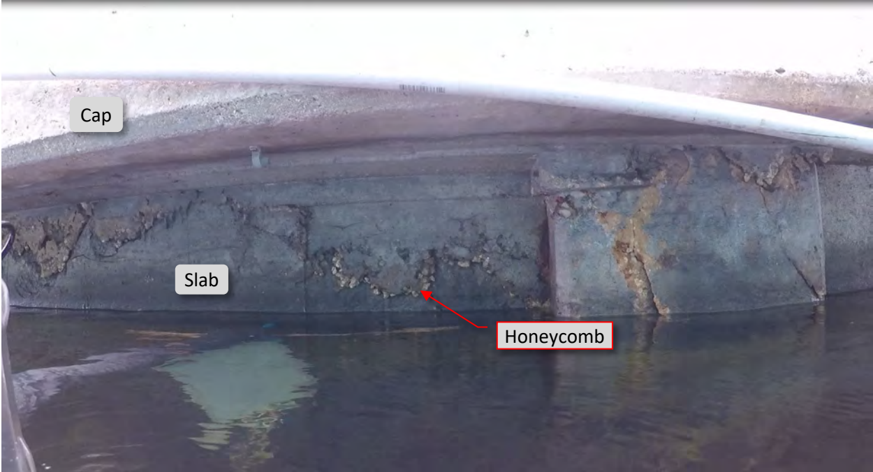
Figure 23: S5. STA 2+93 - 2+99. Honeycomb at top of slab. North direction view.
