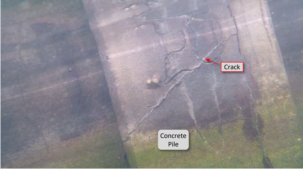
Figure 10: P4. STA 2+35. Multiple cracks and spalls at pile. Underwater view.
