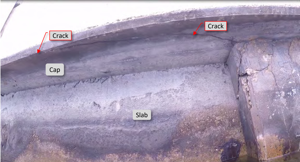
Figure 97: C6. STA 5+25 - 5+30. Crack at cap bottom face.
