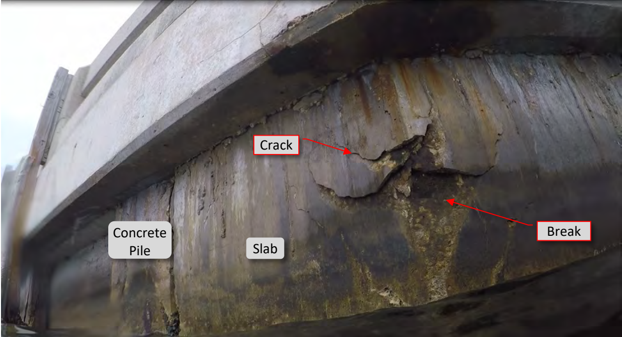
Figure 129: S24. STA 6+11. Crack at slab corner and loss of material.
