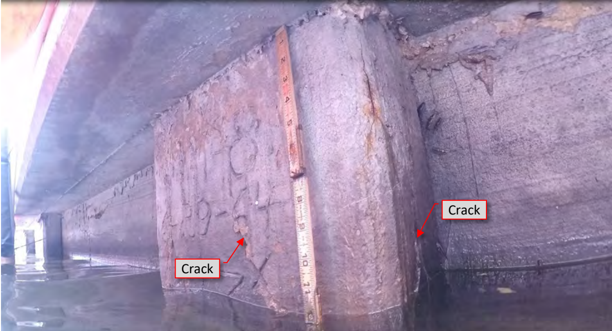
Figure 74: P27. STA 4+60. Crack/spall at top of east flange.
