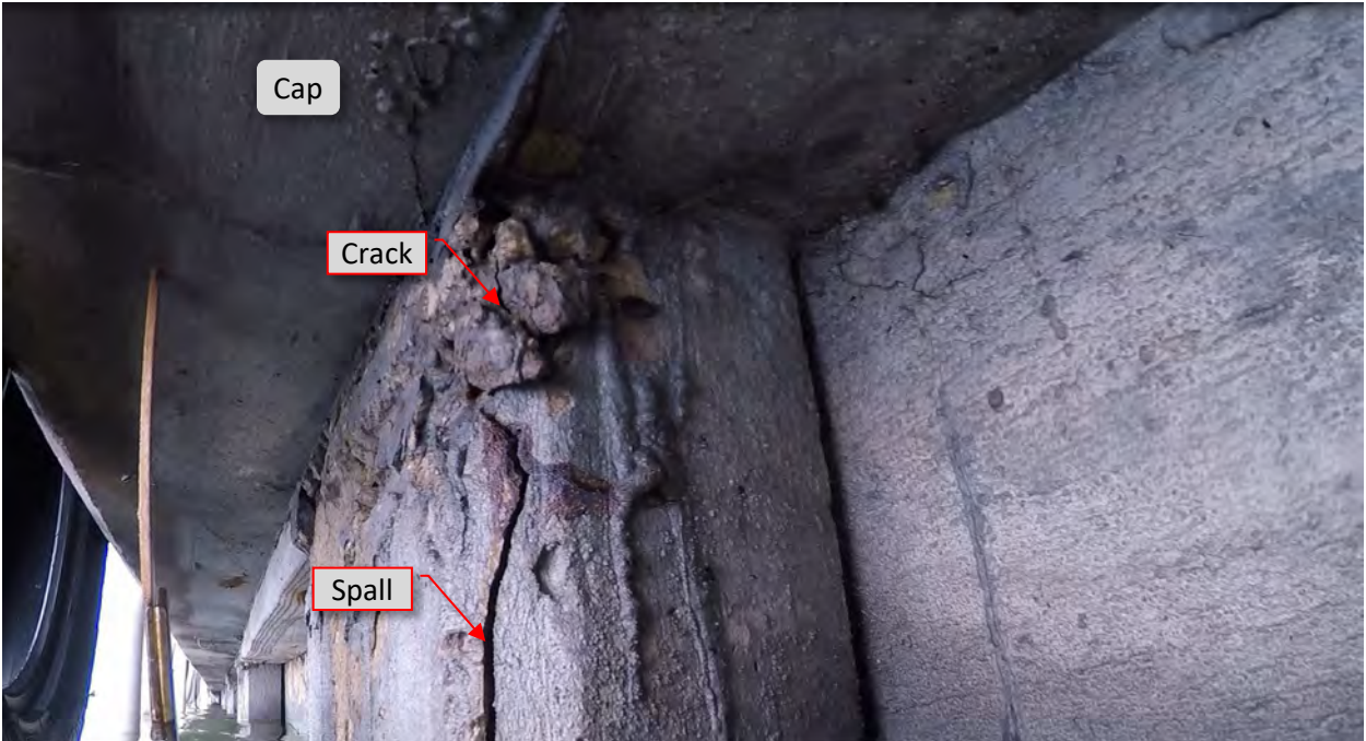
Figure 44: P16. STA 3+56. Spall/crack on south side and near east flange at pile. Honeycomb area at top of pile.
