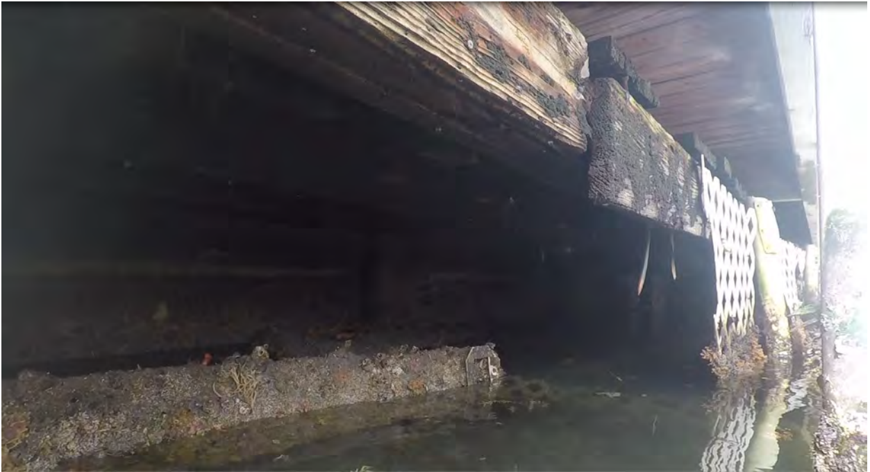
Figure 12: STA 0+70. Northeast direction view. Obstructions and debris in front of seawall, and partial view of seawall.
