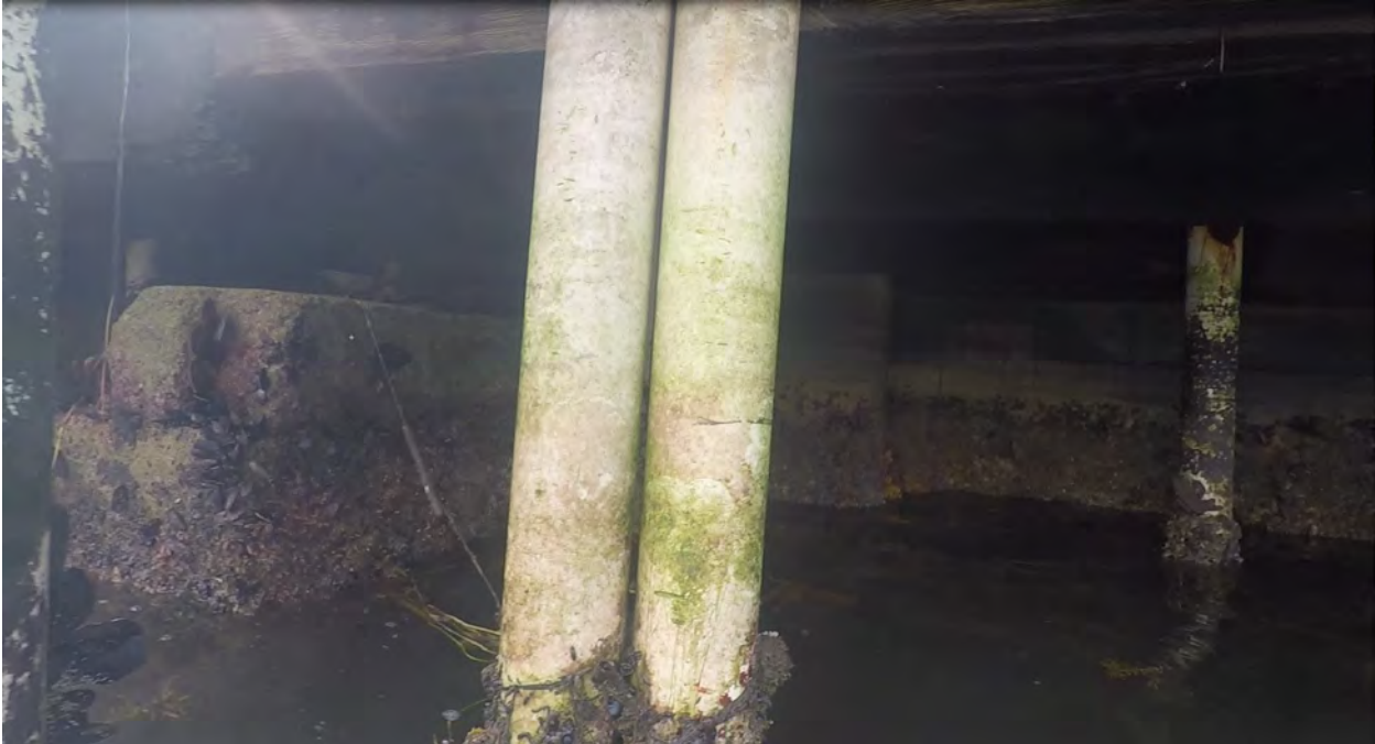
Figure 5: STA 0+20. Northwest direction view. Obstructions and debris in front of seawall, and partial view of seawall.
