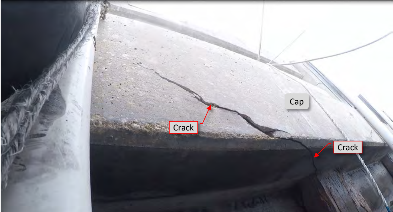
Figure 107: C8. STA 5+51 - 5+55. Crack at cap's bottom and south faces west of pile.
