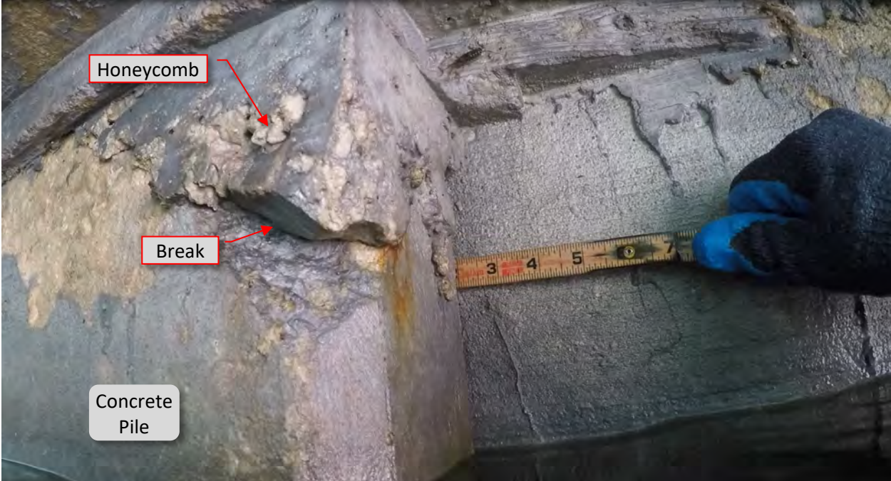
Figure 27: P10. STA 3+07. Break at top east flange corner at pile. Honeycomb area.
