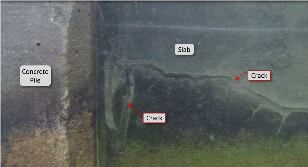
Figure 26: S6. STA 3+01 - 3+04. Two perpendicular cracks on slab at mid height from shelf to cap. Underwater view.
