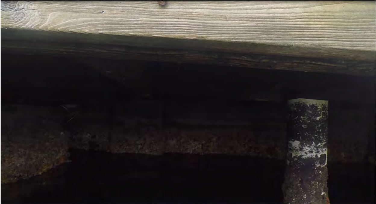
Figure 14: STA 0+90. North direction view. Seawall partial view with present debris, and partial view of seawall.
