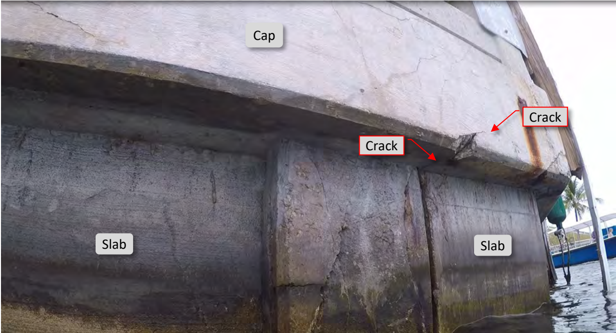
Figure 116. C9. STA 5+75 - 5+90. Crack at cap's bottom and vertical faces in the eastward direction, starts from pile.
