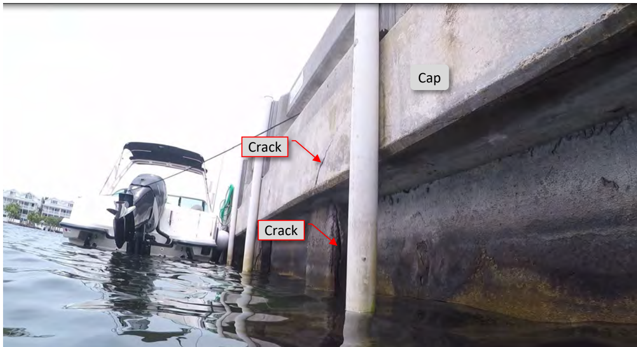
Figure 96: P33. STA 5+24. Crack/spall at top east flange with rust staining. C5. STA 5+24 – 5+26. Crack at cap south face.
