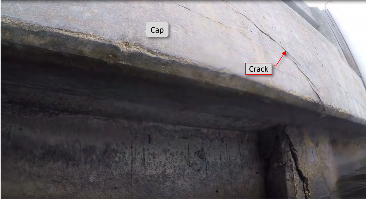
Figure 92: C4. STA 5+11 - 5+16. Crack on cap's south face.
