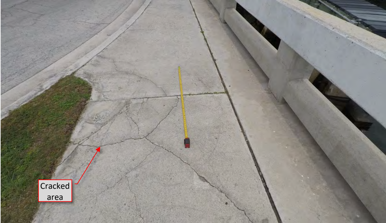
Figure 5: STA 6+50 - 6+60. Cracks in concrete slab to sidewalk.
