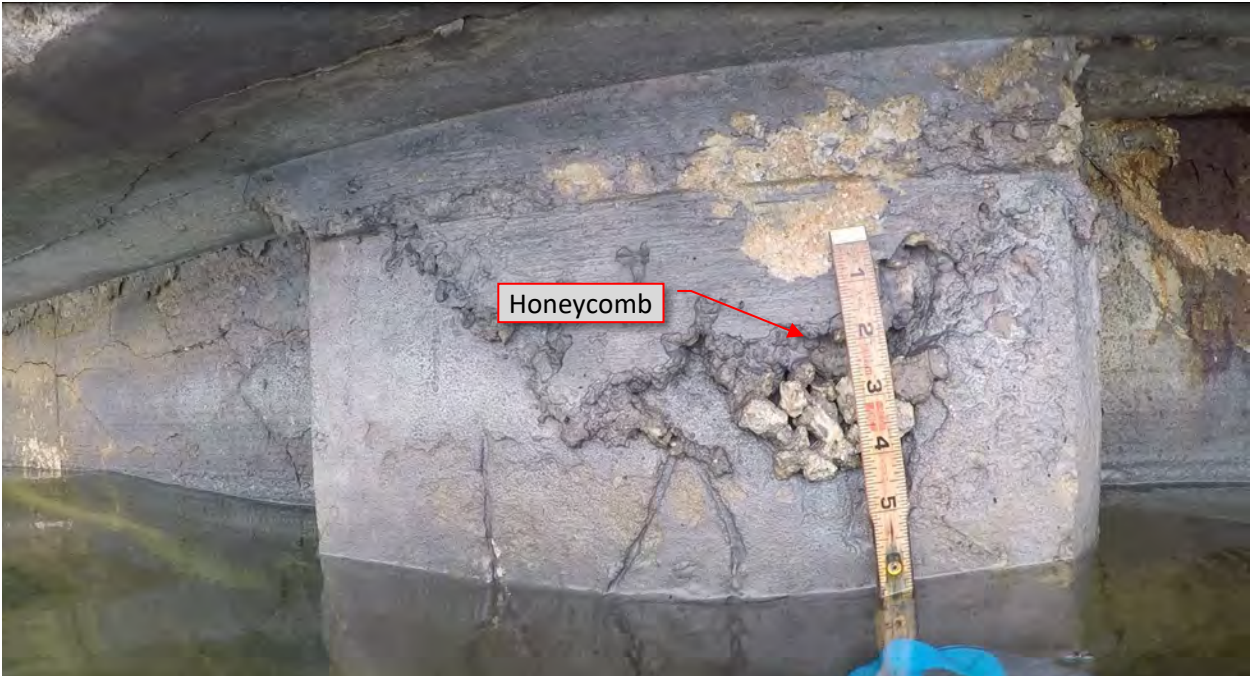
Figure 36: P14. STA 3+39. Honeycomb area at pile.
