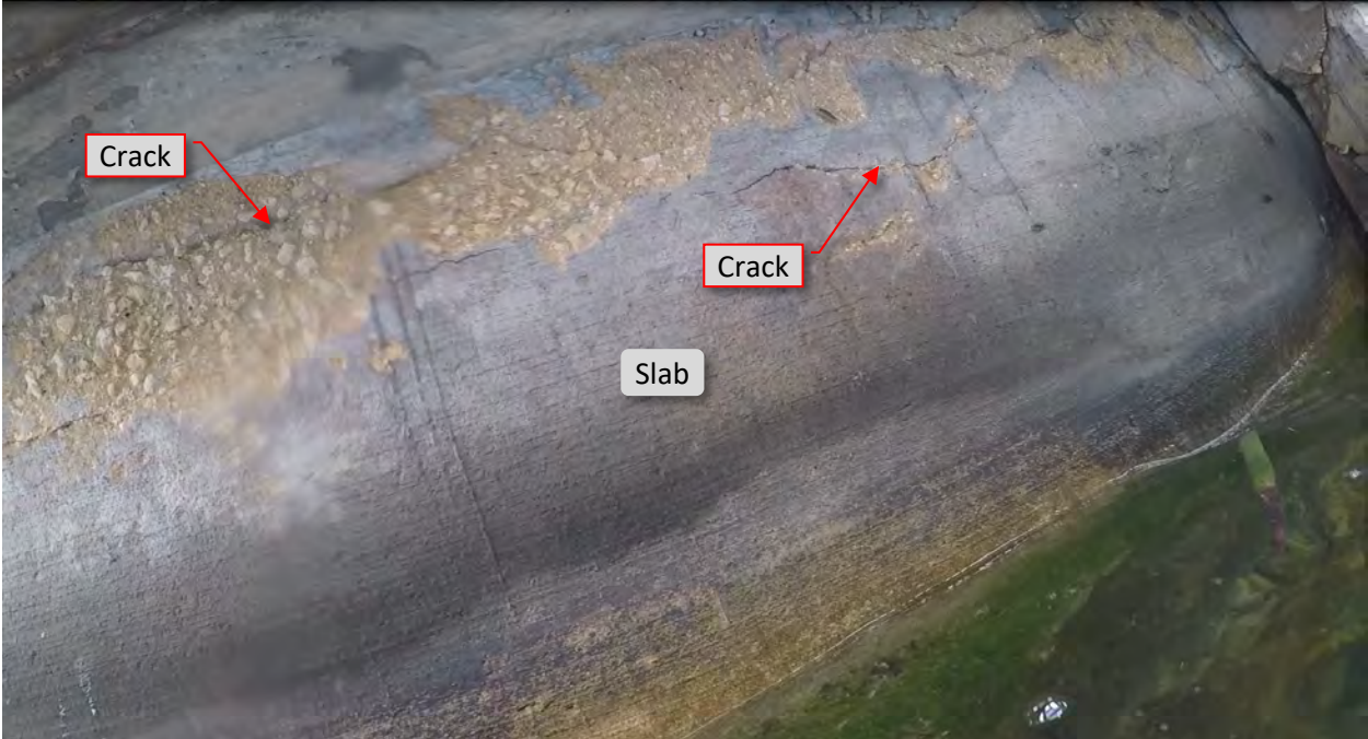
Figure 103: S22. STA 5+42 - 5+47. Crack at top of slab.
