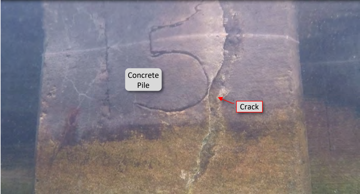
Figure 7: P3. STA 1+72. Crack/spall at pile. Underwater view.
