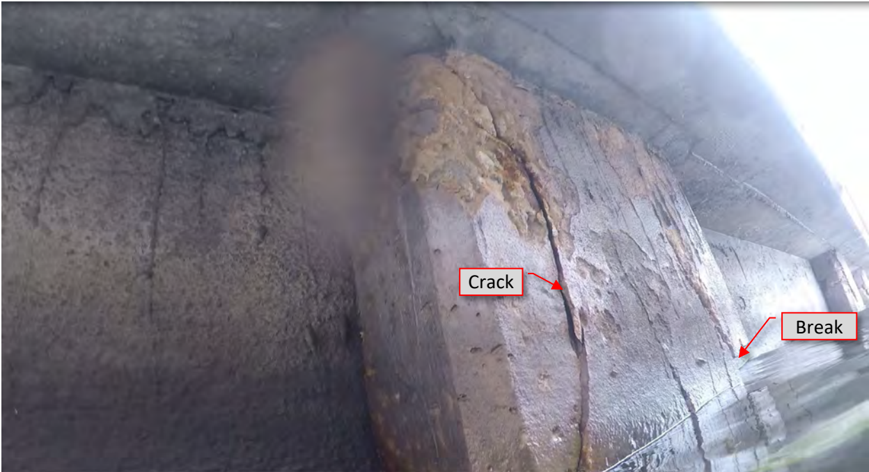
Figure 90: P31. STA 5+08. Cracks/spalls at both flanges at pile and loss of concrete.
