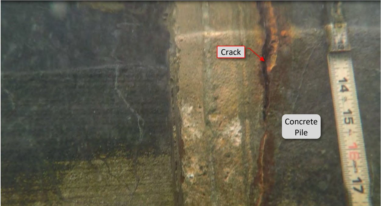
Figure 84: P29. STA 4+92. Cracked and spalled west flange and rust staining at pile
