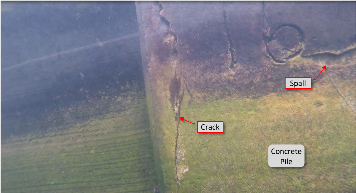
Figure 16: P6. STA 2+76. Crack/spall at west flange on pile. Underwater view.
