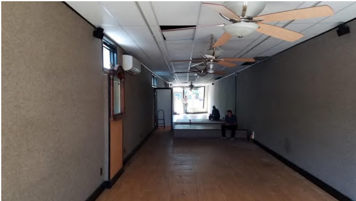
General view of the interior of building 2, the circa 1948-64 front addition. This is the long thin building fronting on Simonton, adjacent to the 1890's warehouse. It was built as commercial space.
