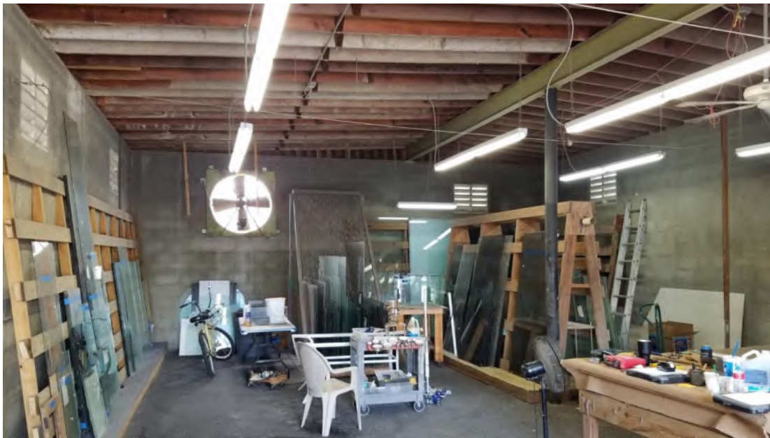
General view of building 5 interior. Constructed between 1948-65. Finishes include concrete floors, concrete walls, steel columns, and open wood roof framing.
