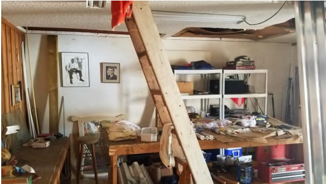
General view of 'Ice House' building 4 at rear of property. Circa 1948-65. Used as office space. Finishes include concrete floors and walls and ceilings.
