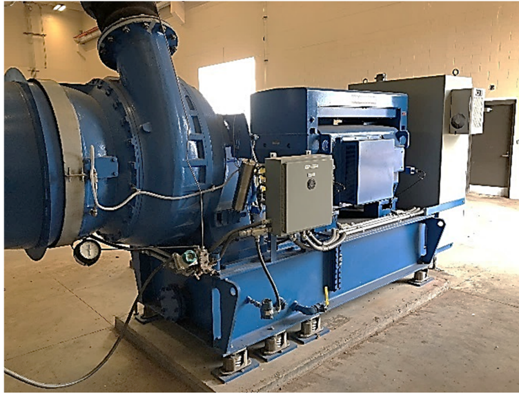
Figure 3-2: Single stage blower without enclosure
