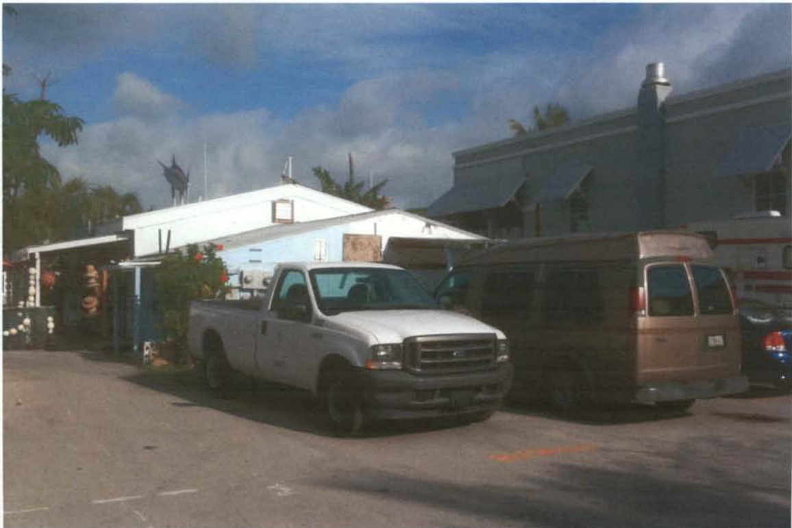
VIEW OF EXISTING BUILDING TO BE DEMOLISHED WITH BAIT SHOP IN BACKGROUND
