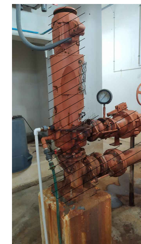
F PHOTO WAS PUMP (TYPICAL)
