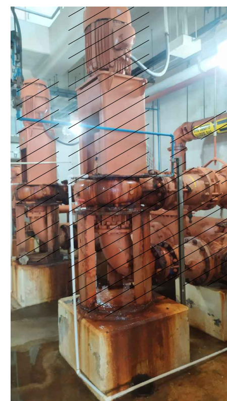
E PHOTO RAS PUMP (TYPICAL)
