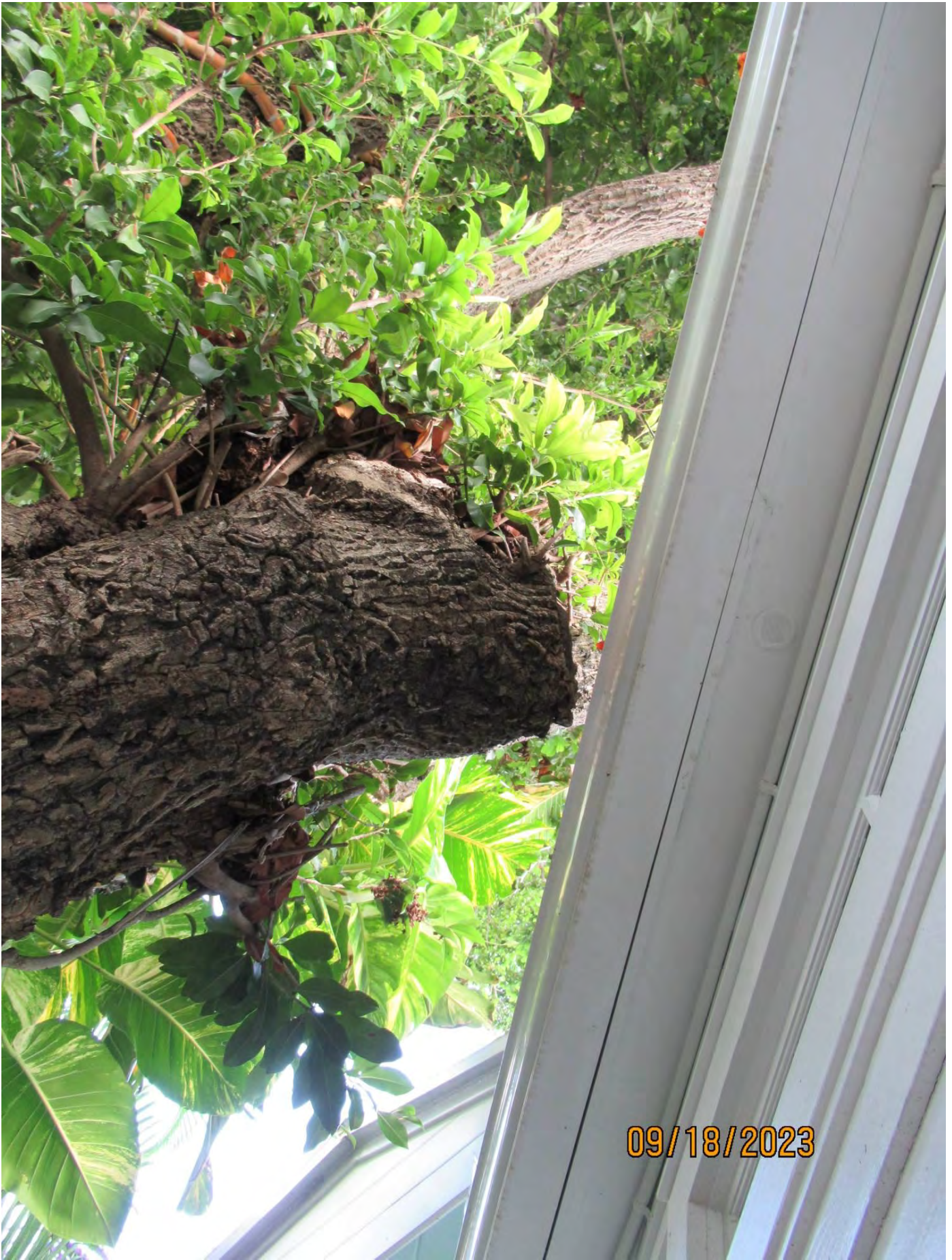
Photo showing large canopy trunk section over structure.
