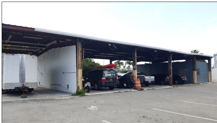
Image of the parking canopy with small structure at one end to be removed.
