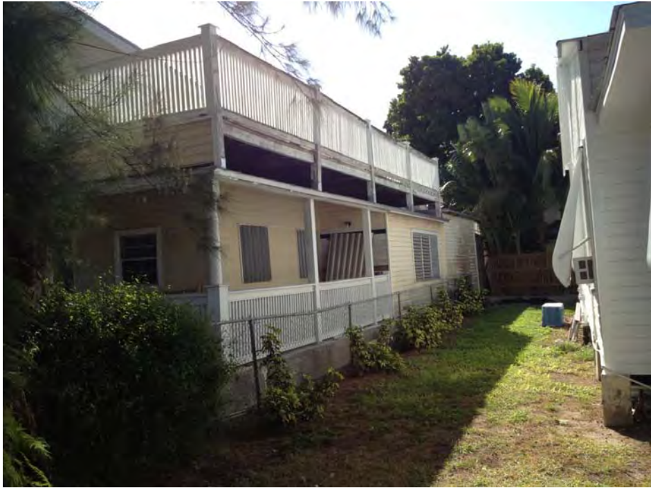
View of side of north side of structure (right side) from Georgia Street
