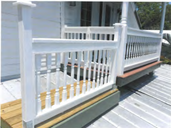
Partial Front View of the Walkway. Railing is exact same size and construction of the existing railing on Center Porch
