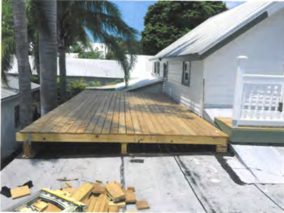
Deck as completed to date. There is no finish yet – it will be a solid color wood stain and sealer approximately the color of the existing shingle roof. Railing has yet to be constructed – it will match existing railing on Center Porch
