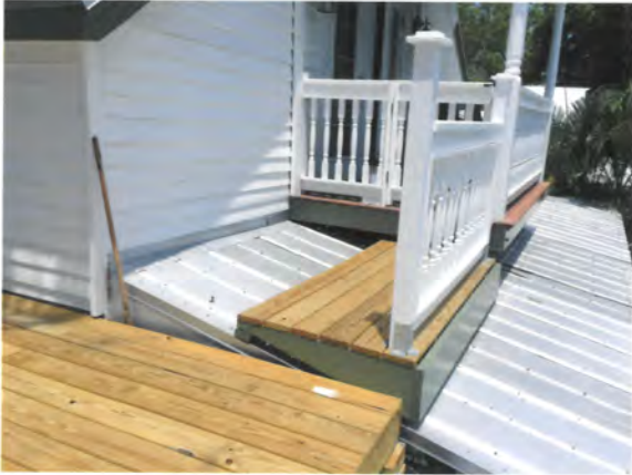
Partial View of deck and the Walkway between existing center porch and deck. There is no finish here either, but it will be the same as the deck
